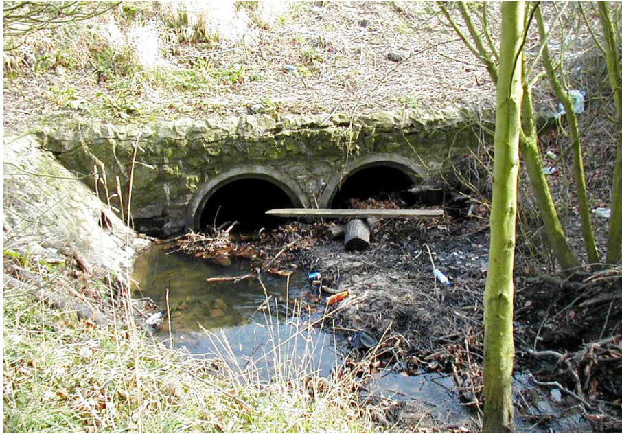
Figure 2.2 Example of reduction of flow area due to partial blockage at a culvert
