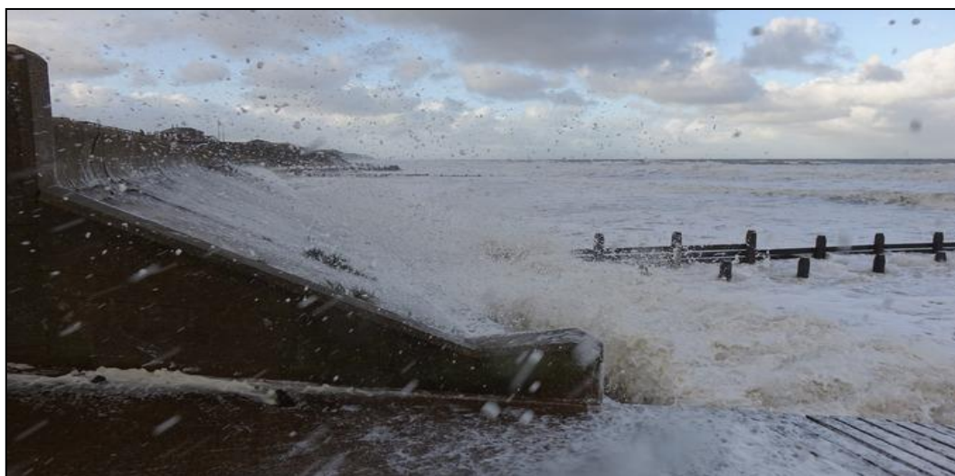
Figure 4.44 Waves impacting the seawall structure at Walcott in 2013
