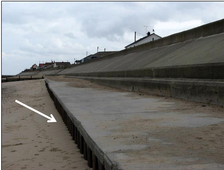
Figure 4.40 Seawall at Walcott showing partially exposed steel sheet pile wall (white arrow)
