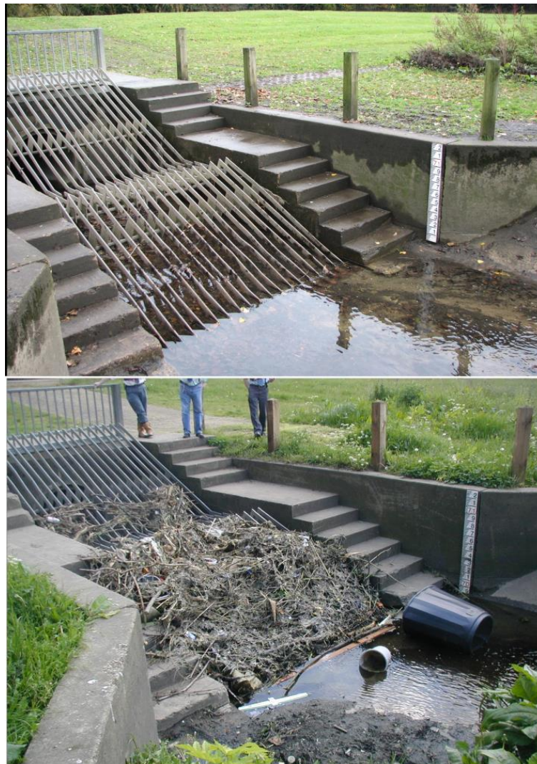
Figure 3.12 Simple screen without an intermediate platform, cleaned by manual raking from the sides and bed
