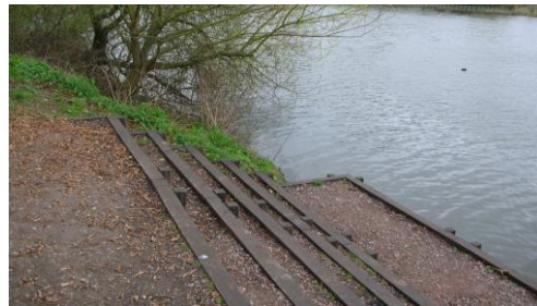
(d) New steps and lower fishing platform following lowering of retention level
