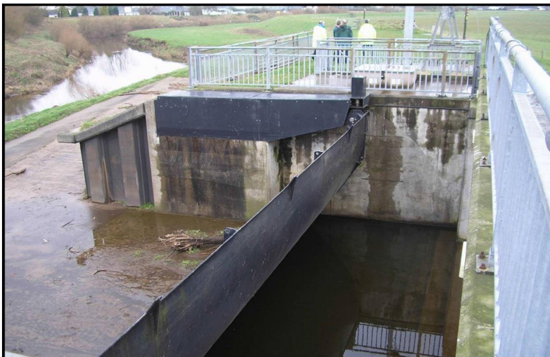
Figure 4.2 Fish belly gate control shown closed
