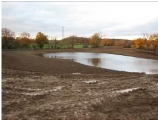
(a) Cobbins Brook borrow area reinstated as a wetland pond. The photograph was taken in November 2009 immediately following construction.
