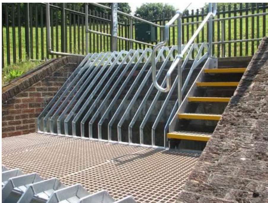
Figure 3.15 Two-stage screen retrofitted to a headwall: the platform and steps are constructed from a non-slip, free draining, glass-reinforced plastic grating
