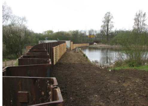
(b) Newly finished dam, formed from steel sheet piles, behind the existing concrete dam
