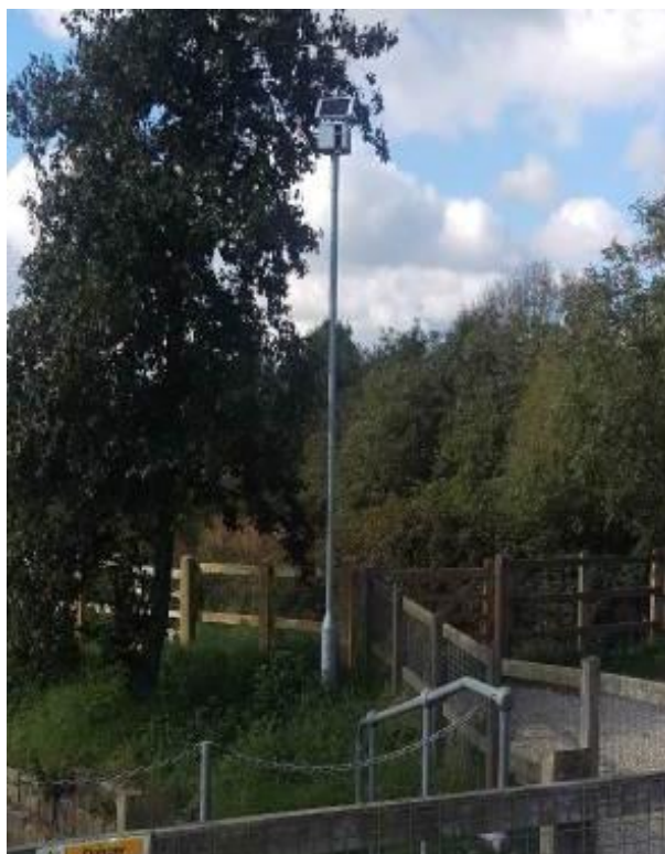
Figure 3.19 Solar panel operated CCTV at Swanage flood storage reservoir taking still images
