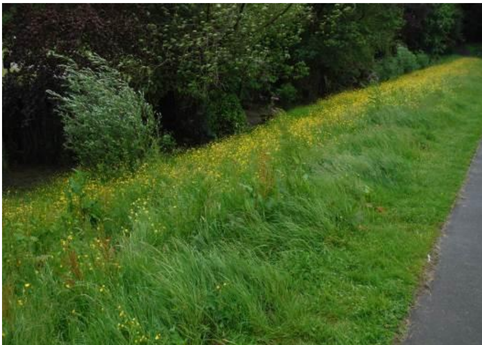
Figure 3.8 Long grass on the downstream embankment face and trees/shrubs at the toe area prevent effective surveillance of the embankment performance
