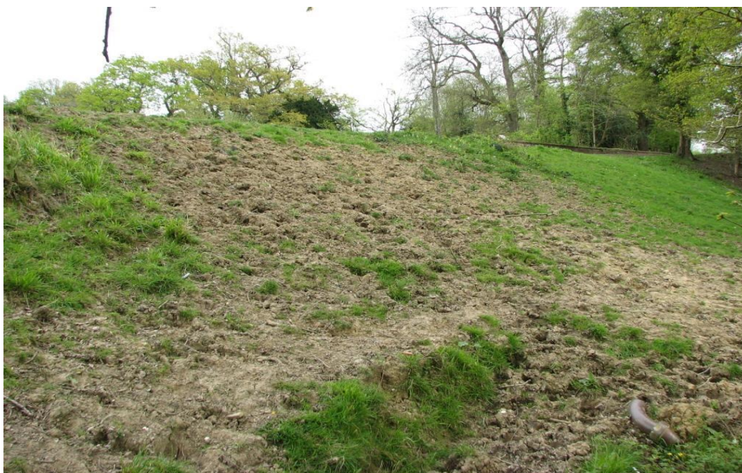
Figure 3.16 Serious cattle poaching on the downstream face of a flood storage embankment
