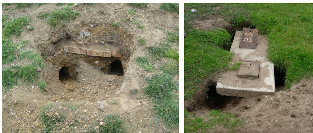
Figure 3.17 Rabbit burrow damage (left), Badger damage (right)
