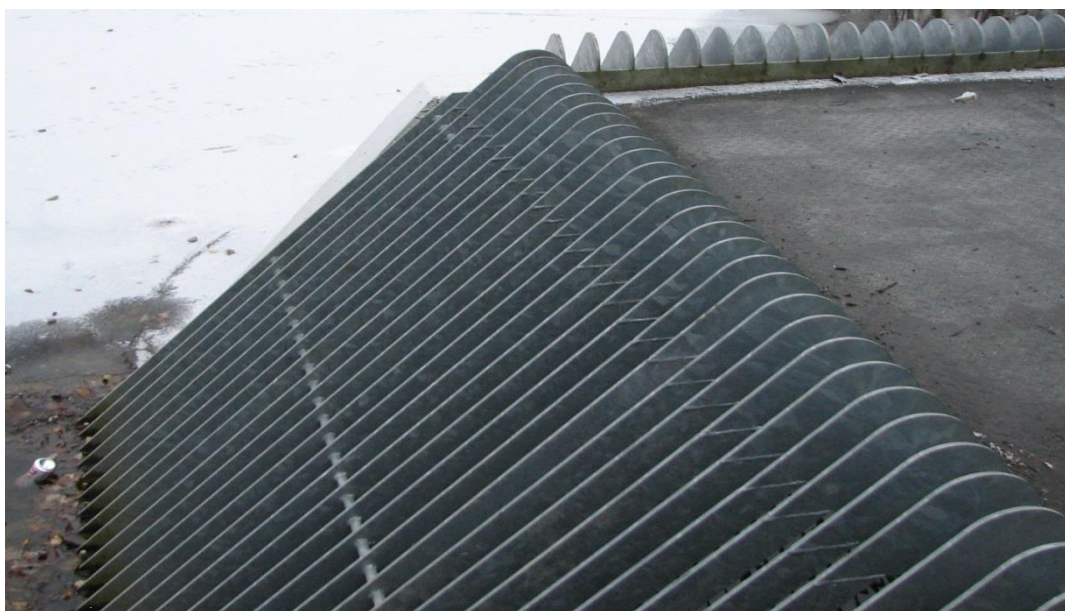
Figure 3.14 The intermediate horizontal support bar of this screen is insufficiently recessed to allow efficient manual raking over the screen's full height
