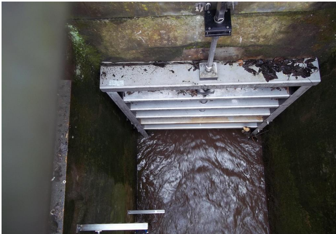
Figure 4.3 Online vertical penstock control
