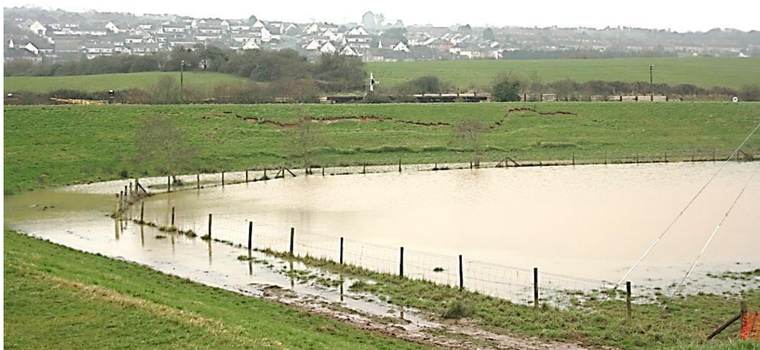
Figure 3.2 Shallow slope failure at Swanage flood storage reservoir following impoundment in October 2013
