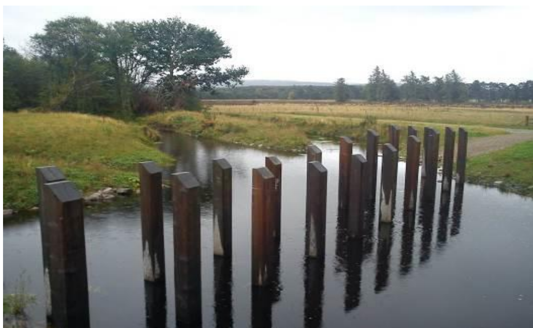
Figure 3.11 Tree catcher for the Moray Council flood storage reservoir
