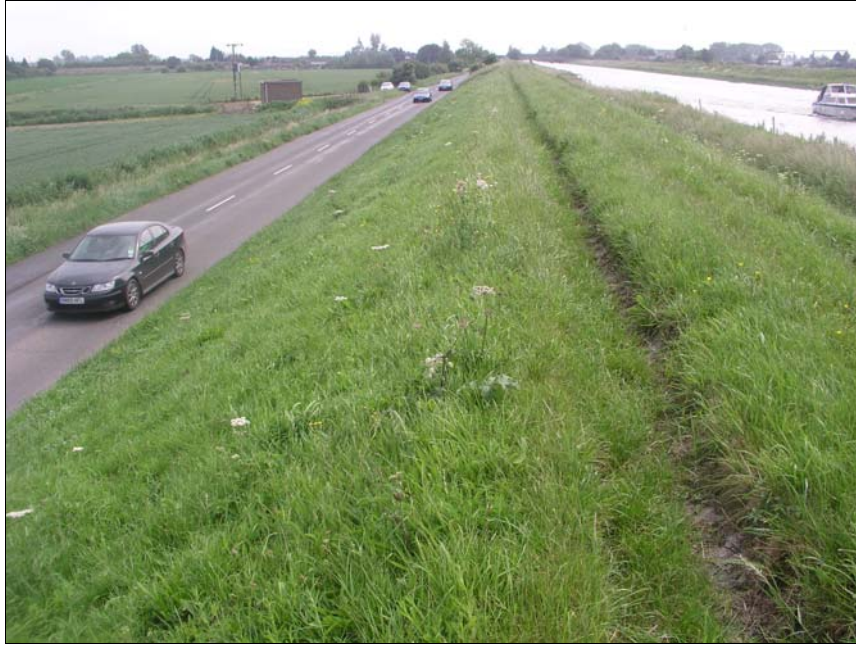
Figure 4.141 Ely Ouse Community A photographed on the landward face of Treatment 1 in June 2007.
