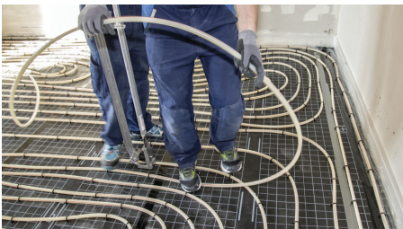
Under floor heating rather than radiators or kick/plinth heaters
