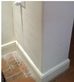
Walls - hydraulic lime plaster (with salt resistant additive) on steel mesh supported by wooden battens (to create air gap).
