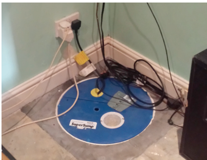
Sump and pump sited in corner of lounge, carpet tiles over concrete floor are easily removable
