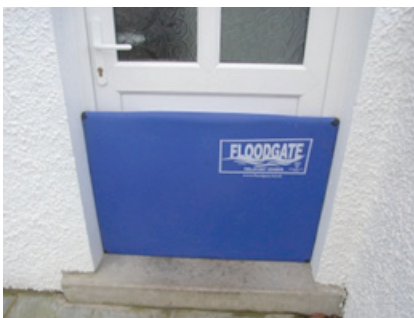
Might not be possible to keep water out entirely but water exclusion / minimisation strategy employed
