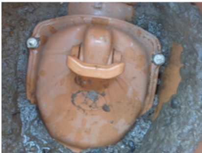
Non return valves to prevent back up and minimise clean up
