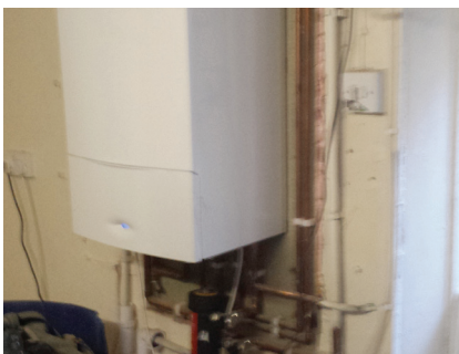
Boiler (and electrics) mounted above expected flood level
