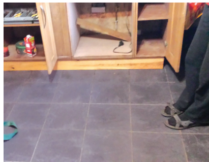
Marine ply kitchen units, with solid oak doors – can be hosed down and disinfected (picture taken 10 days after flood).
