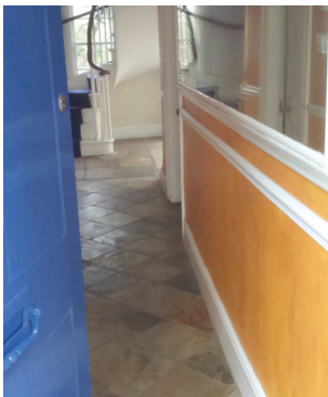
Walls finished with lime plaster and 'old-fashioned' paint; dado to mark where post-flood decoration needs to go up to.
