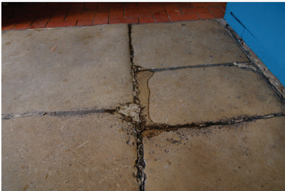
Water comes up through the floor but tiled floors are easy to mop up after a flood.
