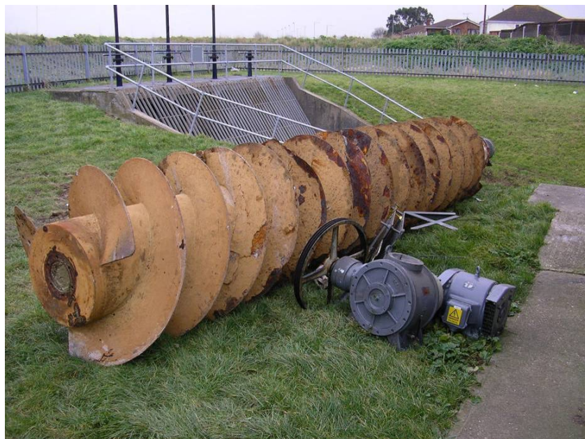
Figure 3.5: Typical three-flight screw removed for servicing
