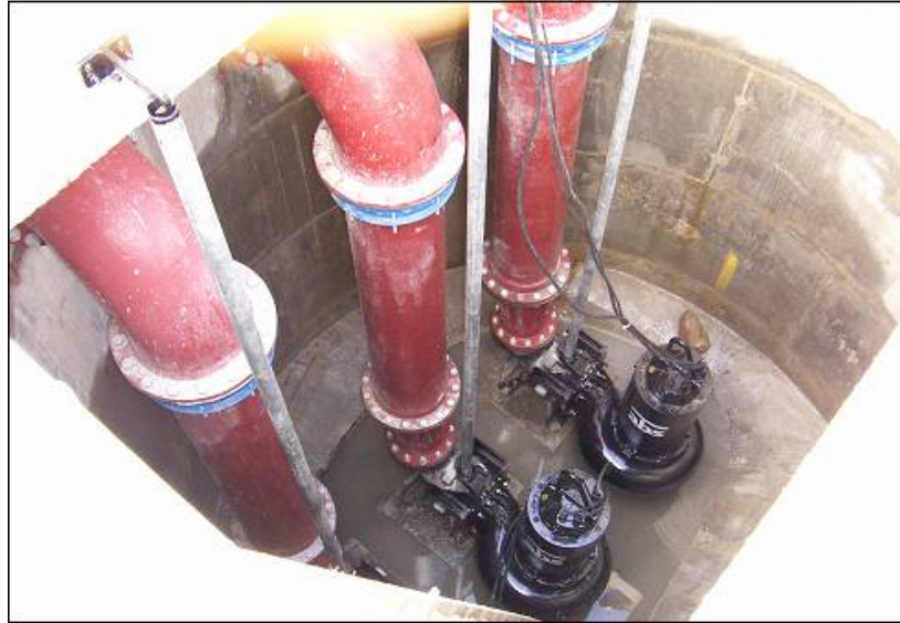
Figure 3.11: Typical submersible transfer pump installation (top cover removed)
