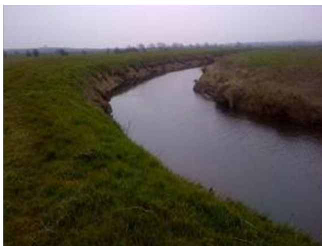
Figure 3.1 This semi natural channel looks clear of obstructions, but siltation which has become vegetated on the bank shoulders has reduced the channel capacity over the past 15 years. Siltation below water level could not be assessed in this turbid water.
