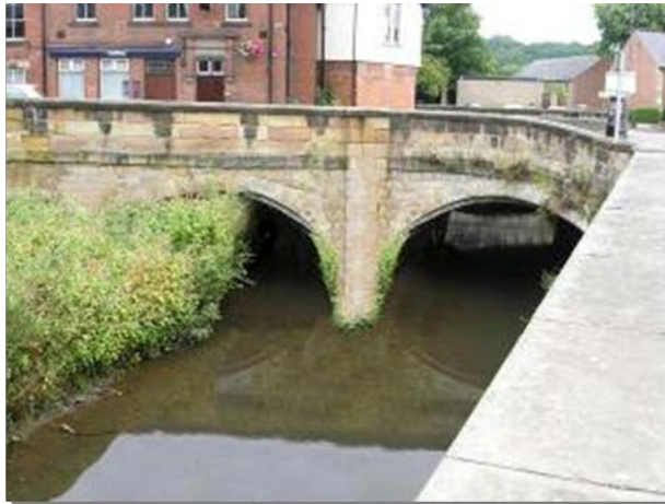
Figure 3.11 An edited photograph to show the level of blockage where a first alert should be raised – an ‘amber’ alert.
