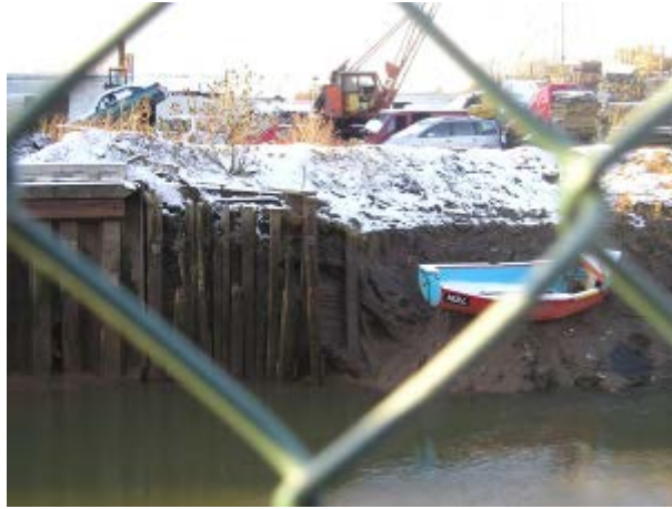
Figure A.2.7 This is clearly not a new issue and riparian responsibilities may be important in deciding whether action should be taken. However, the obvious problems at this transition should be recorded through a red alert. This is also likely to be reflected in the condition grade of the 'defence – high ground'.
