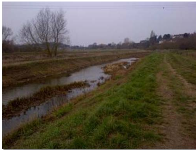
Figure 3.3 Open channel – natural and defence – embankment with no berm to relieve flood flows. There is moderate accumulation of weed in channel and vegetated shoaling, which could affect channel conveyance.
