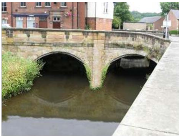
Figure 3.12 An edited photograph showing an acceptable channel with no alerts required – the ‘green’ condition.
