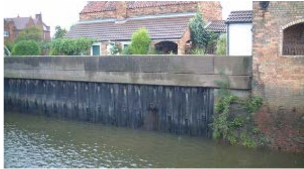
Figure A.2.2 A smooth transition between materials lining a channel. Although vegetation growth may cause an issue in the future, on this evidence there is no need to raise either a red or amber alert for the transition.
