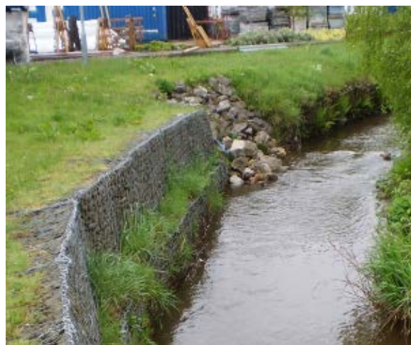
Figure A.2.6 A failure of a bank at the transition with an upstream gabion wall. The tipped stone may have already been placed to stabilise this and it also may not be clear whose responsibility this is. The collapse does not itself increase flood risk. An amber alert may be appropriate to ensure the wider asset management team is aware of the issue.
