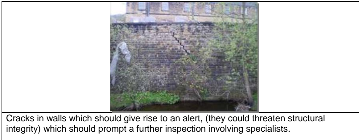
Figure A.11.1 Typical evidence of cracking or fissuring
