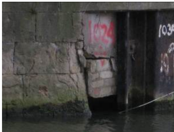
Figure A.2.8 This transition between sheet piles and a masonry wall has the potential for backfill washout close to the current water line when subjected to high fluvial flows. An amber alert is appropriate to raise awareness and to ensure the transition is monitored for any further movement or loss of integrity.
