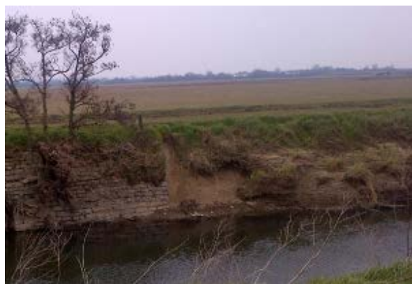
Figure A.2.3 A typical transition between stone work channel side and a natural bank where erosion can occur. On this evidence there is no need to raise either an amber or red alert, particularly bearing in mind the low consequences of failure in this rural location.
