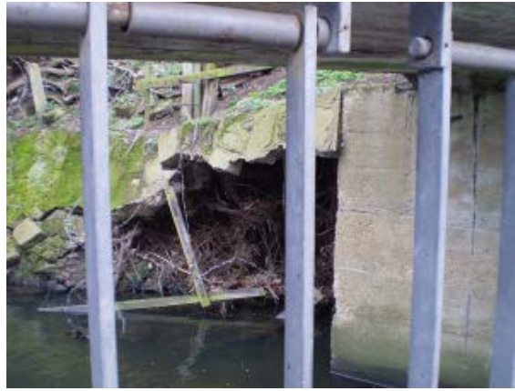
Figure A.2.5 A problem at a transition between a revetted bank and a bridge abutment. This should be highlighted as a red alert as there is a risk of progressive erosion of the downstream bank.
