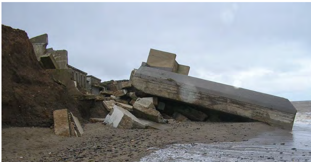
Figure 5.3 Undermining of wartime coastal structures at Kilnsey, Holderness (courtesy of ENBE)
