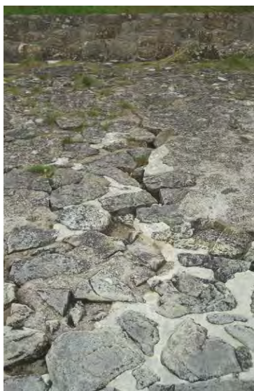
Figure 2.4 Extensive crack in masonry toe (courtesy HR Wallingford)
