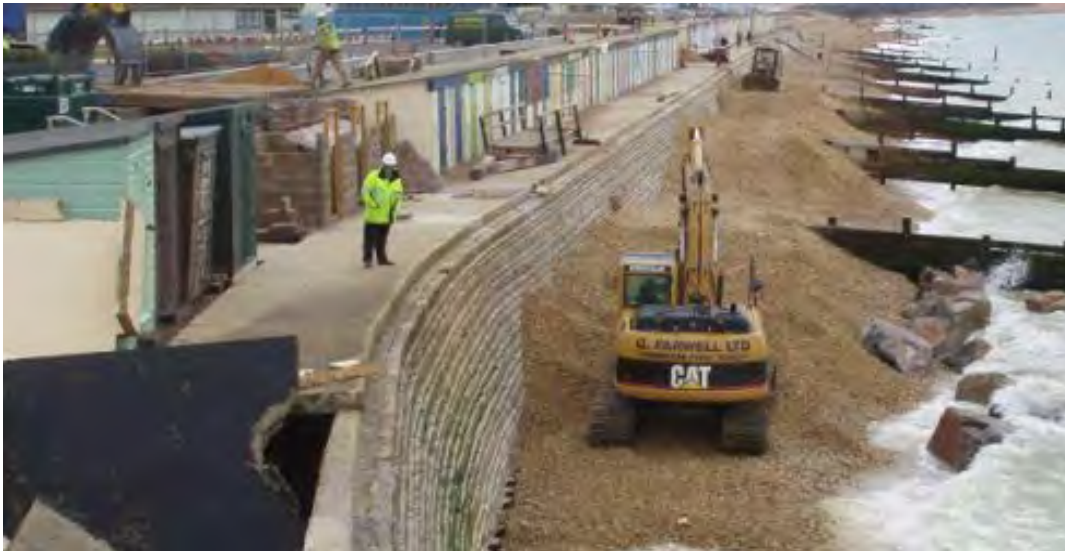
Figure 4.5 Temporary access road constructed from local beach material (courtesy New Forest District Council)
