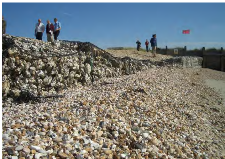
Figure 4.16 Weathered gabions at East Head, Chichester Harbour, West Sussex (courtesy HR Wallingford)
