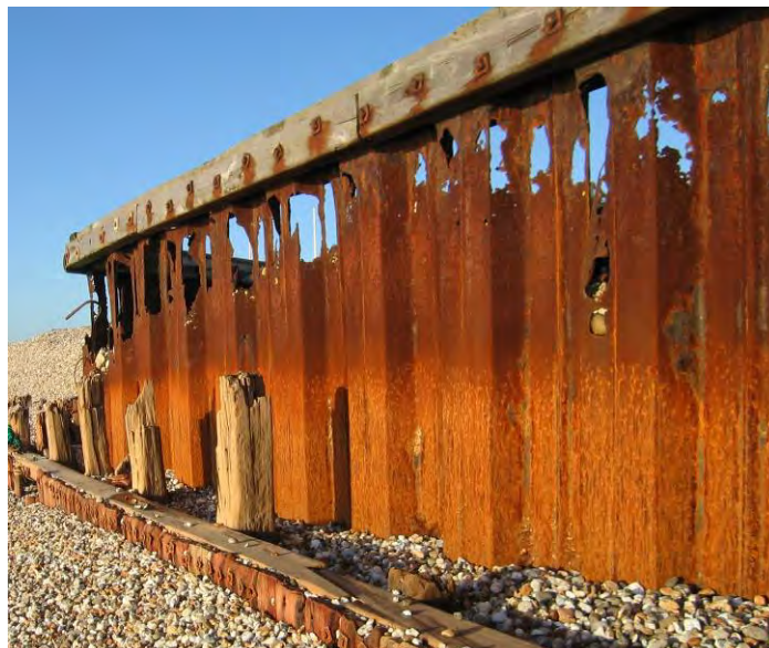
Figure 4.22 Deteriorated sheet piles
