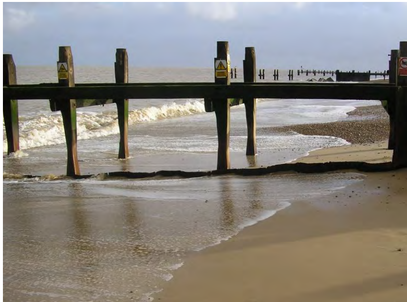
Figure 2.22 Necking in derelict timber piles (courtesy ENBE)
