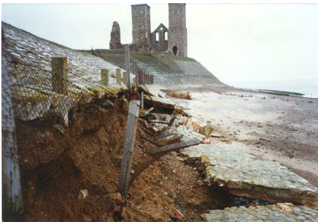
Figure 5.1 Toe failure example
