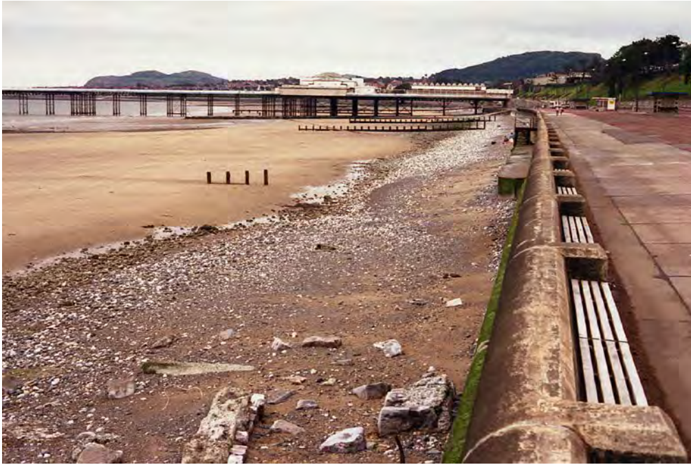
Figure C12.2 Beach lowering in front of vertical seawall, Colwyn Bay
