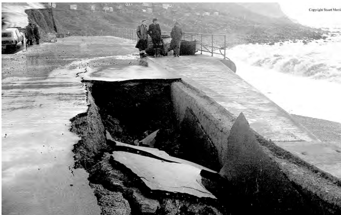
Figure 4.12 Typical collapse of promenade decking following undermining of backfilled mass concrete wall and washout of fine core (Chesil Cove 1962) © Stuart Morris
