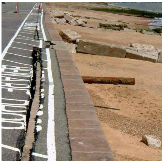
Figure 3.4 A seawall in the process of overturning (courtesy of Black & Veatch)
