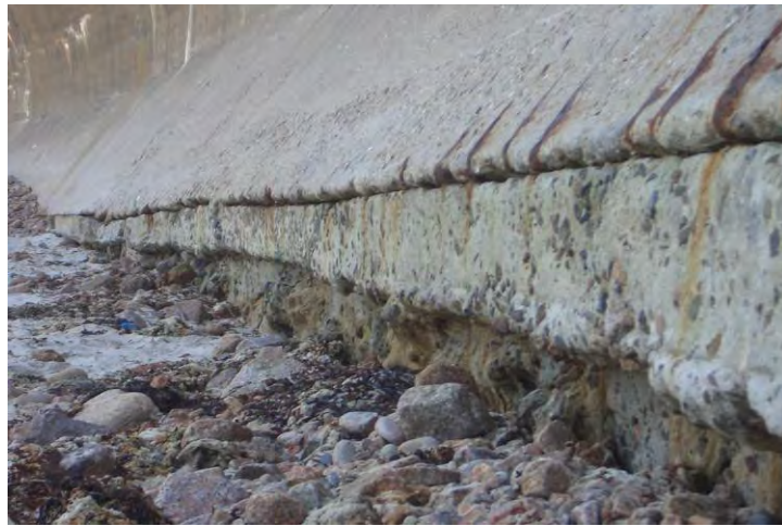
Figure 3.28 Abraded concrete toe and onset of undermining (courtesy of HR Wallingford)
