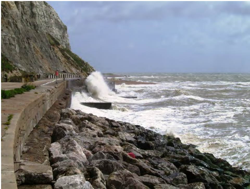
Figure 4.13 Contrast between concrete toe and modified rock armour toe Folkestone Warren (courtesy Bryan Curtis)
