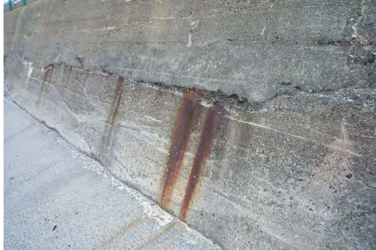
Figure 2.15 Reinforcement rebar corrosion and spalling of concrete (courtesy of HR Wallingford)
