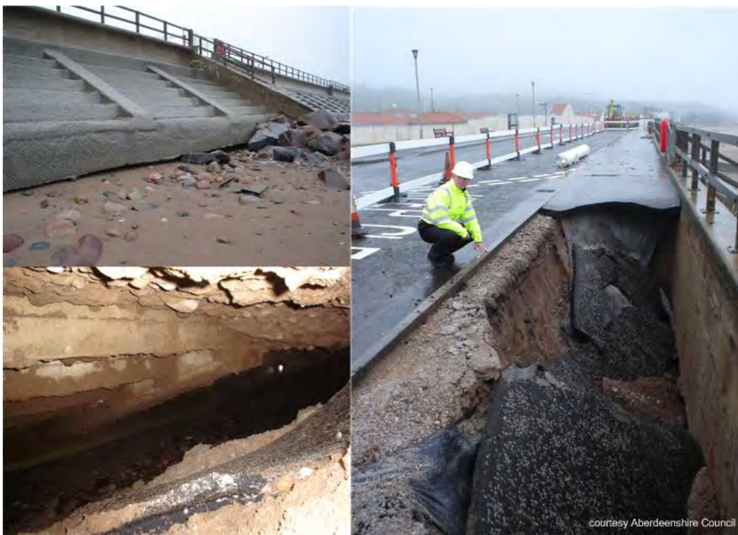
Figure 3.32 Undermining and fill washout of stepped revetment and wave return wall
