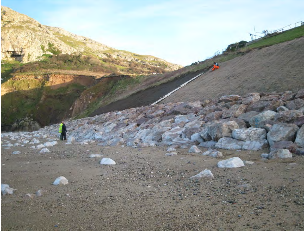
Figure C1.6 Regraded cliff face
