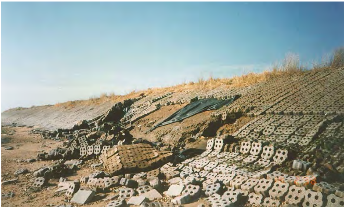
Figure C6.3 Failed flexible armoured revetment
