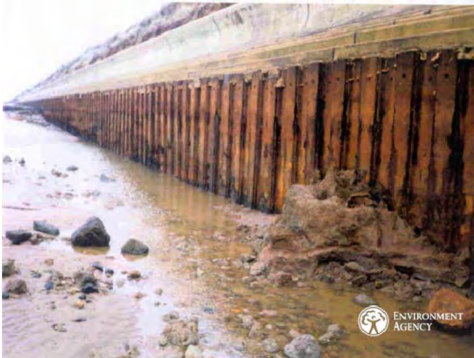
Figure A.19 Erosion of a cohesive shore platform at the toe of a seawall
