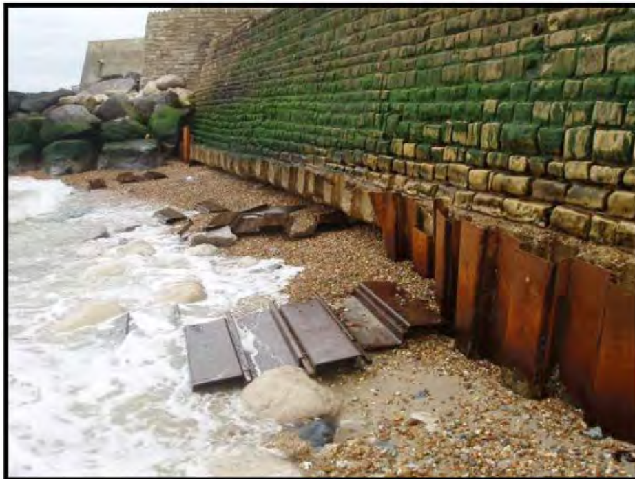
Figure A.9 Example of structural damage to a seawall at Milford-on-Sea (courtesy Andrew Bradbury, New Forest District Council)
