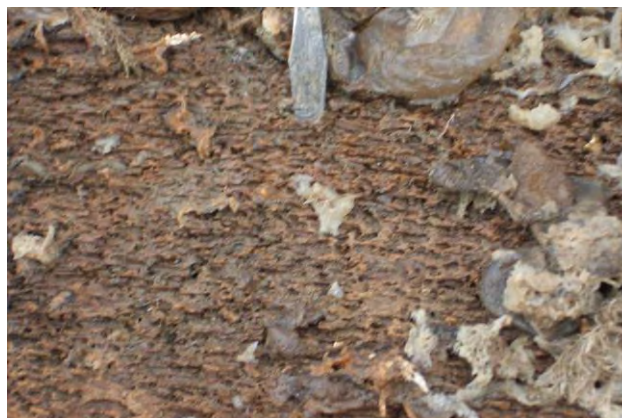
Figure 2.20 Close up of gribble damage to timber (courtesy of HR Wallingford)
