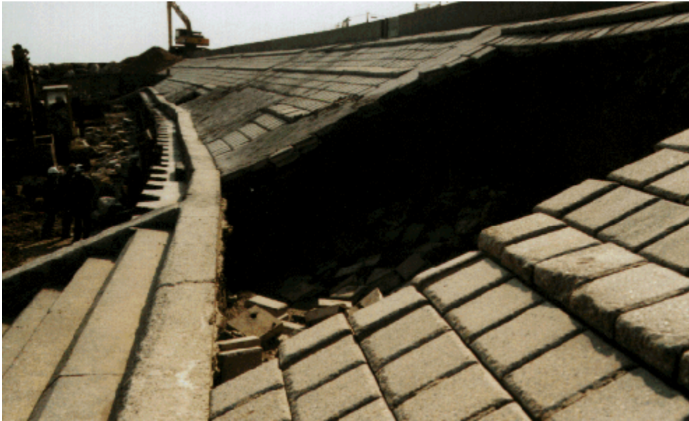
Figure 4.21 Washout and collapse of block revetment following block removal (courtesy Canterbury City Council)
