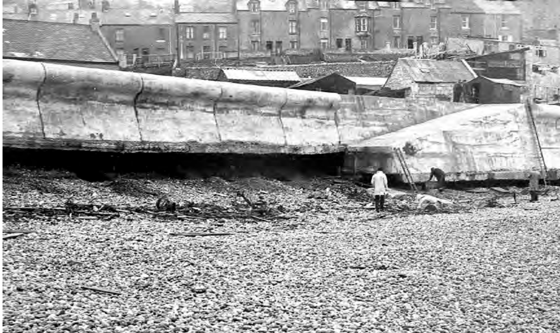
Figure 4.9 Unsupported section of reinforced mass concrete seawall following major undermining (Chesil Cove 1962) © Stuart Morris
