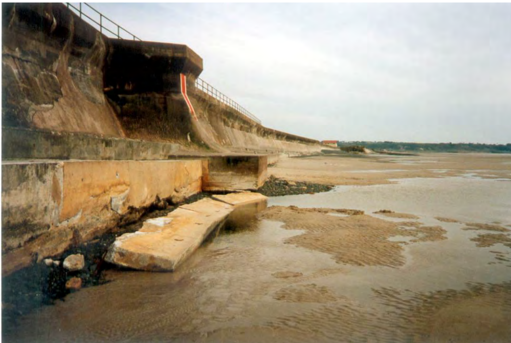
Figure 2.17 Failure of a concrete toe beam at St Ouens Bay, Jersey (courtesy HR Wallingford)
