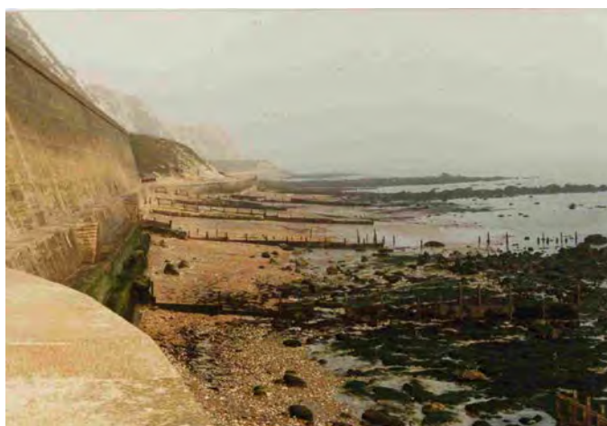
Figure 3.26 An extreme example of beach depletion, foreshore erosion and down-cutting – note the level of the base of the access steps in relation to the level of the beach (courtesy HR Wallingford)
