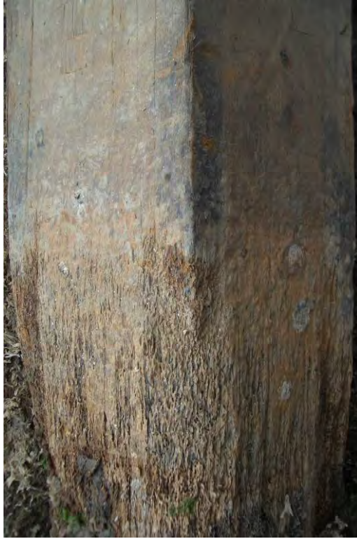
Figure 2.19 Gribble attack on Timber pile at the sediment line (courtesy of HR Wallingford)
