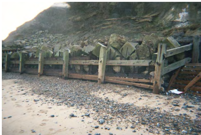
Figure 2.3 Cribwork and concrete block fill, Norfolk (courtesy of North Norfolk District Council)
