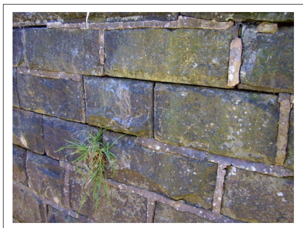
Figure 2.18 An example of poor pointing and missing mortar beds in a spillway wall
