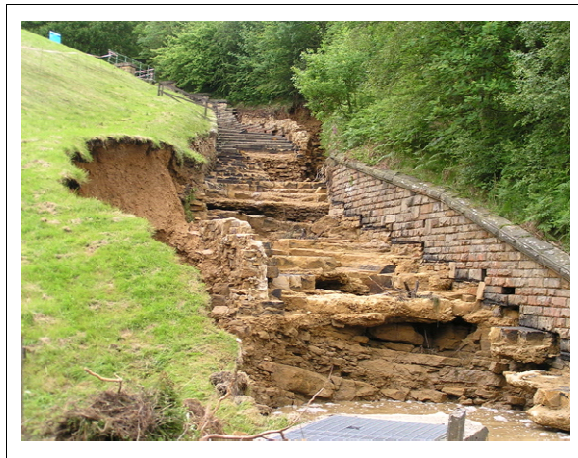
Figure 2.16 An example of a widespread failure of a stepped masonry spillway
