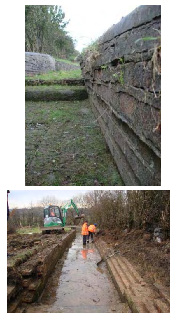
Figure 5.8 Side wall with a definite lean – before and after local demolition. Wall will be rebuilt.
