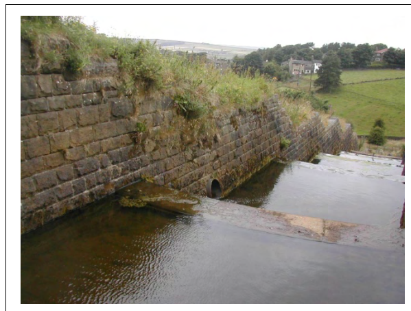
Figure 5.20 Replacement of horizontal invert (impact) masonry slabs of steps with concrete slabs
