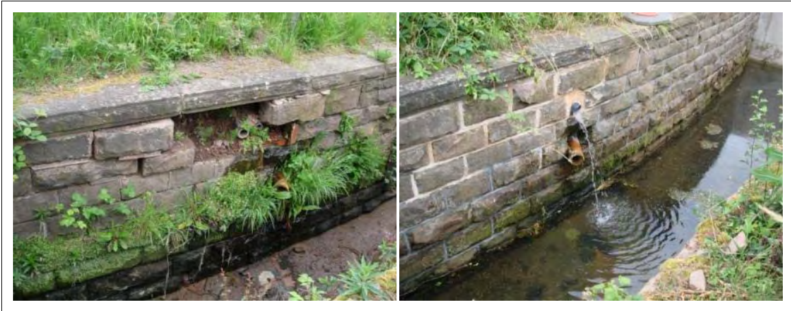
Figure 5.12 Damage to masonry wall repaired by replacement of missing blocks, repointing and fixing of leaky pipe
