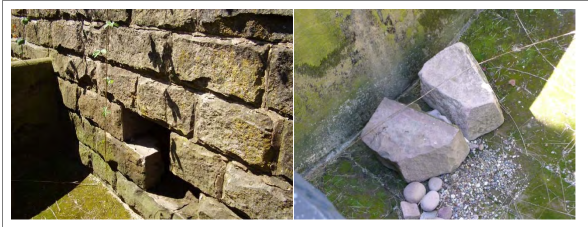
Figure 2.15 Examples of localised loss of masonry blocks
