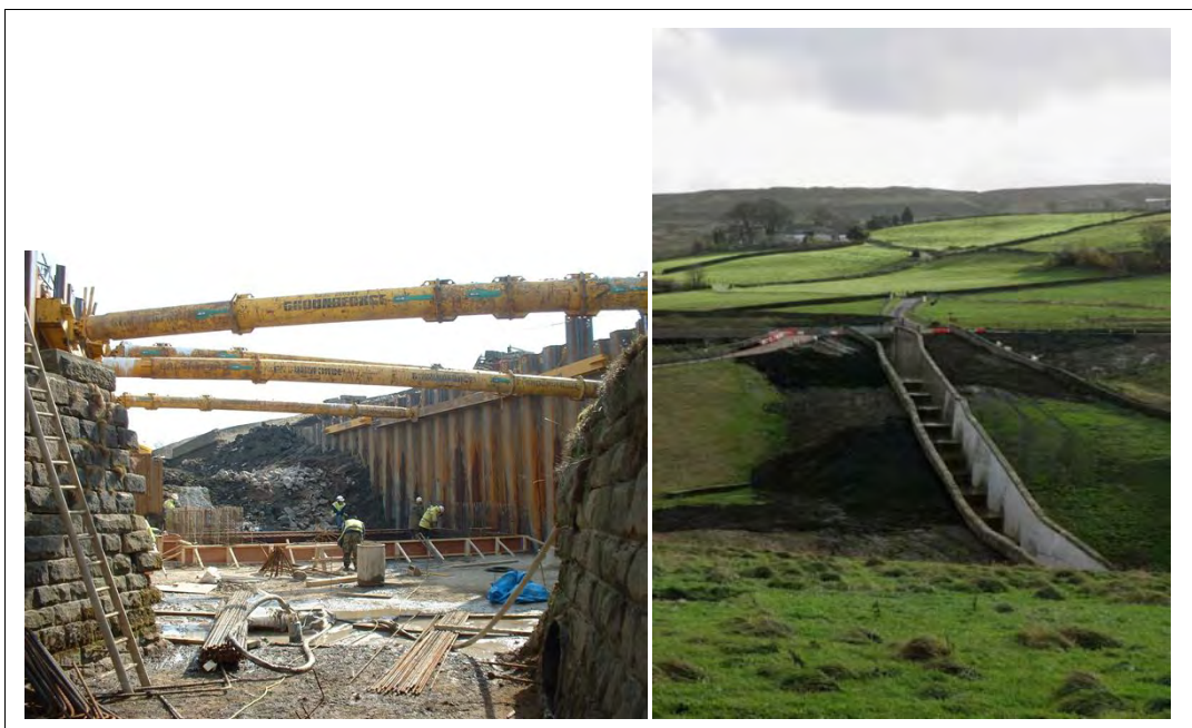
Figure 5.22 Replacement of masonry stepped spillway with new stepped spillway constructed along same line in reinforced concrete
