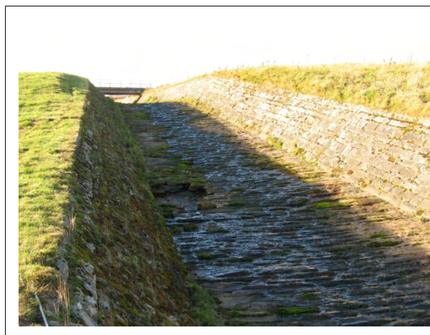
Figure 2.2 An example of a sloping bed in a masonry spillway, with the wall masonry laid parallel to the bed.
