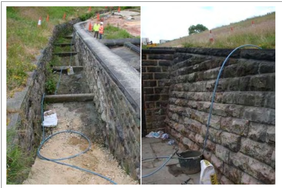
Figure 5.10 Lines along a spillway channel to pressure point both sides of the wall on the right hand side of the spillway
