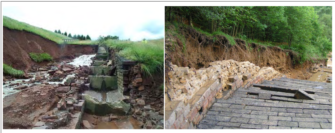
Figure 2.4 Examples of failures of masonry spillways. The spillway wall on the left has random rubble masonry backing, whilst the spillway wall on the right has mass concrete hearting between the random rubble backing and the dressed face.
