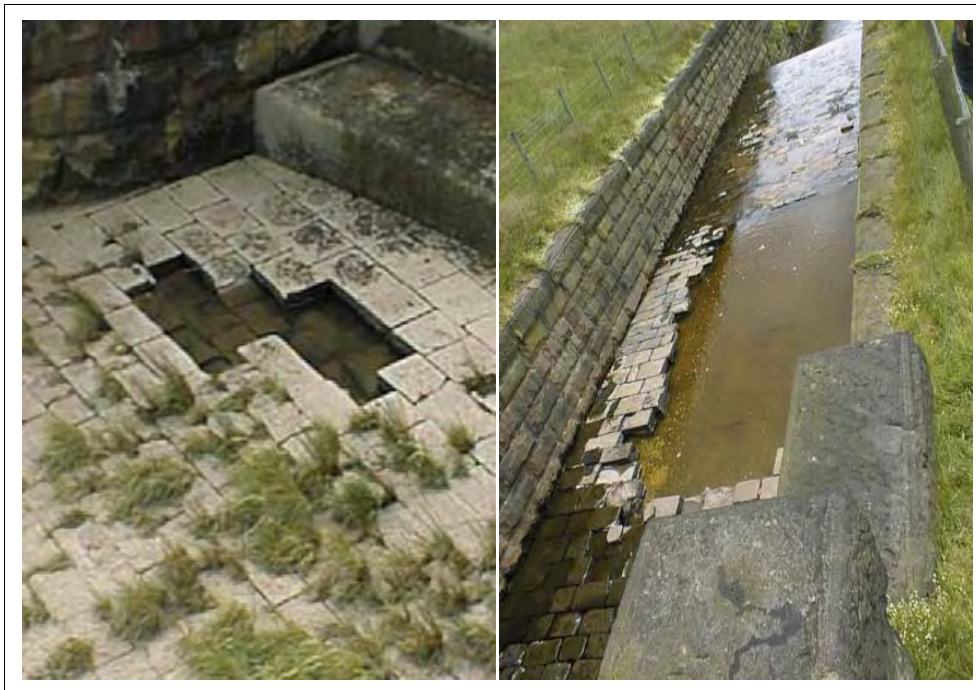
Figure 2.17 Examples of invert failures of stepped masonry spillways
