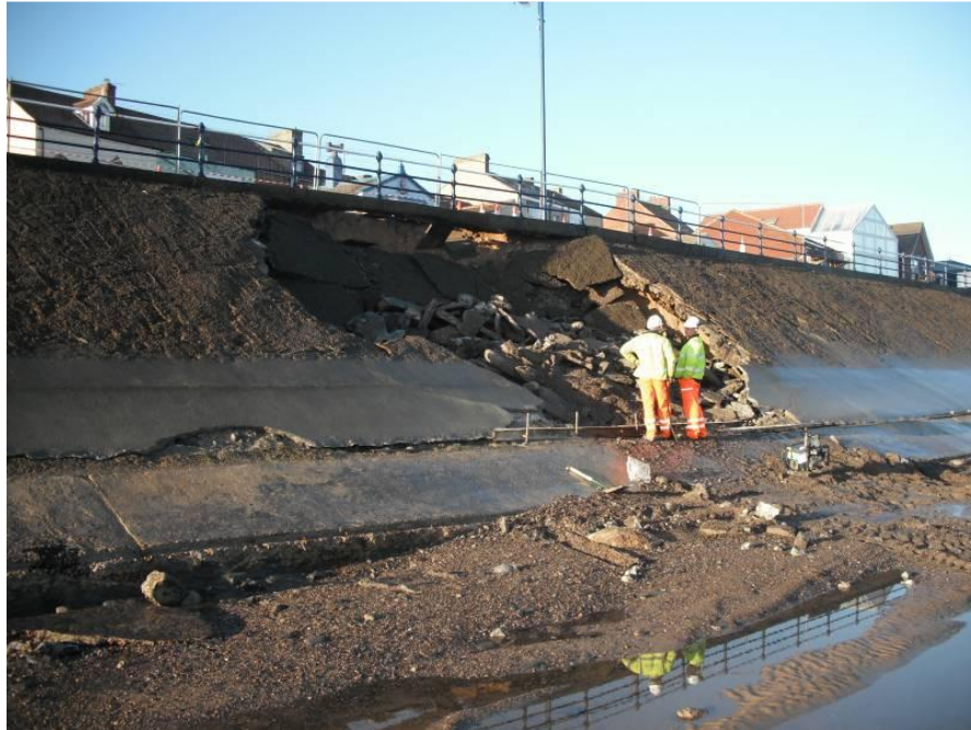
Figure 3. Defence Failure at Redcar. Photograph courtesy of Redcar and Cleveland Borough Council
