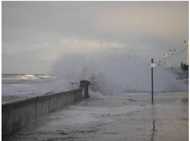
Figure 1. Overtopping at Esplanade on 1 March 2006. Photograph courtesy of Dave Cocks, RNLI Redcar
