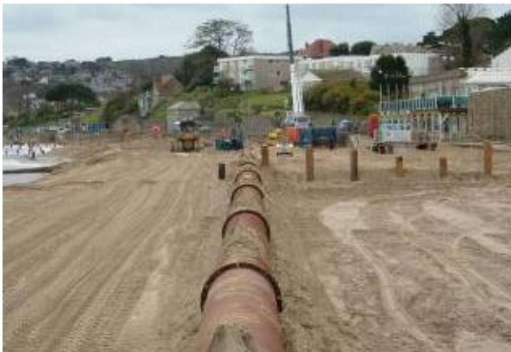
Figure 3. – Beach replenishment and groyne construction at Swanage. Source: David Robson, Borough of Poole Council, 2010
