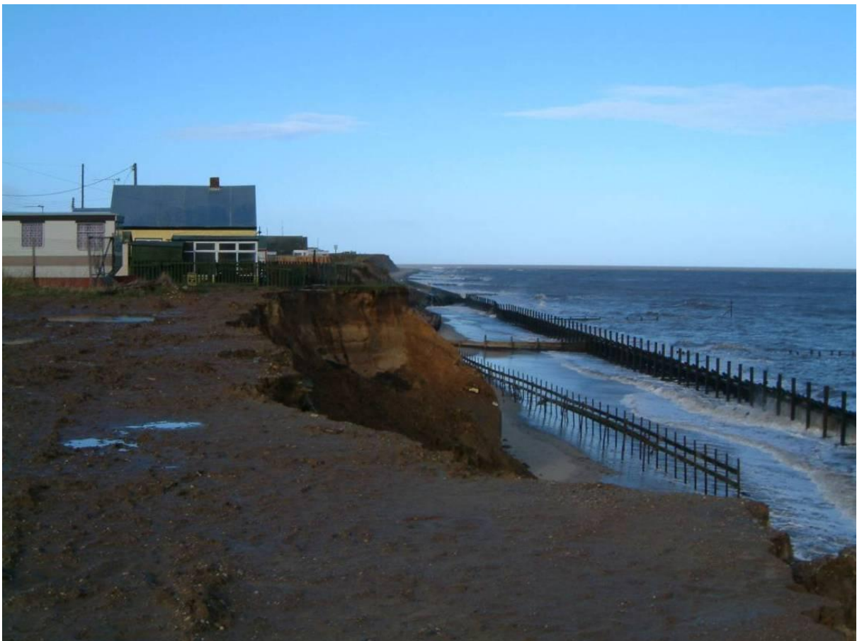
Figure 4. February 2002 - Eroding sandy cliffs behind failing defences. Photography courtesy of North Norfolk District Council
