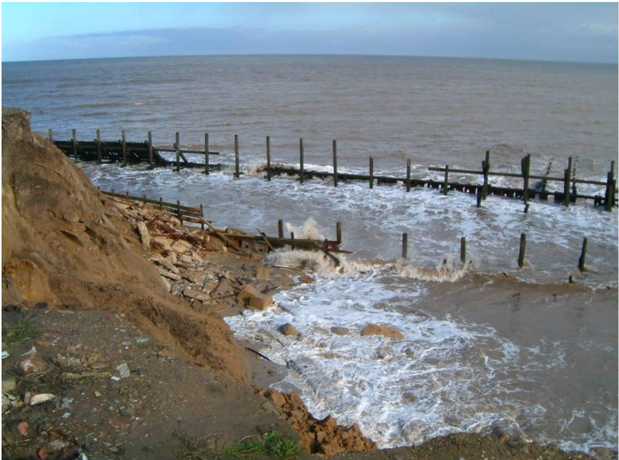
Figure 3. February 2002 - failed revetment. Photography courtesy of North Norfolk District Council
