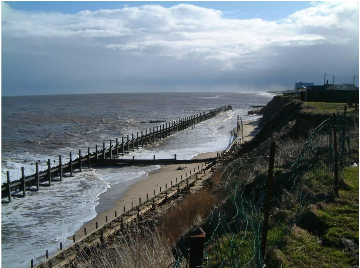
Figure 5. View of deteriorating defences prior to first placement of rock (February 2002). Photography courtesy of North Norfolk District Council
