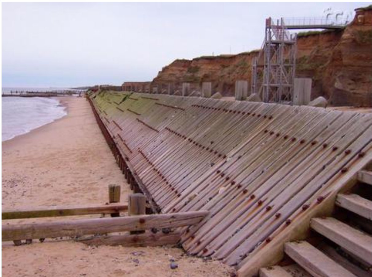
Figure 1. Timber revetment in fair condition. Photography courtesy of North Norfolk District Council
