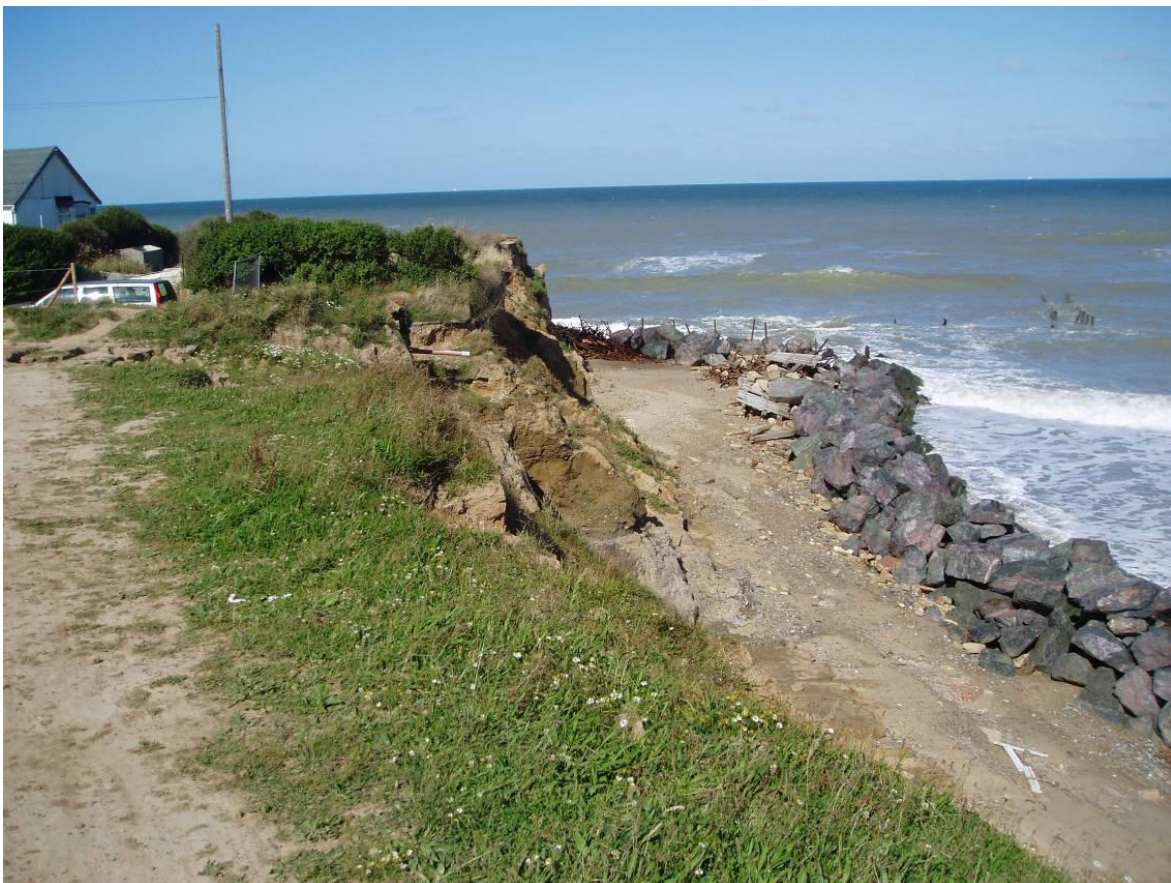
Figure 8. Rock revetment in place at southern end (2007). Photography courtesy of North Norfolk District Council
