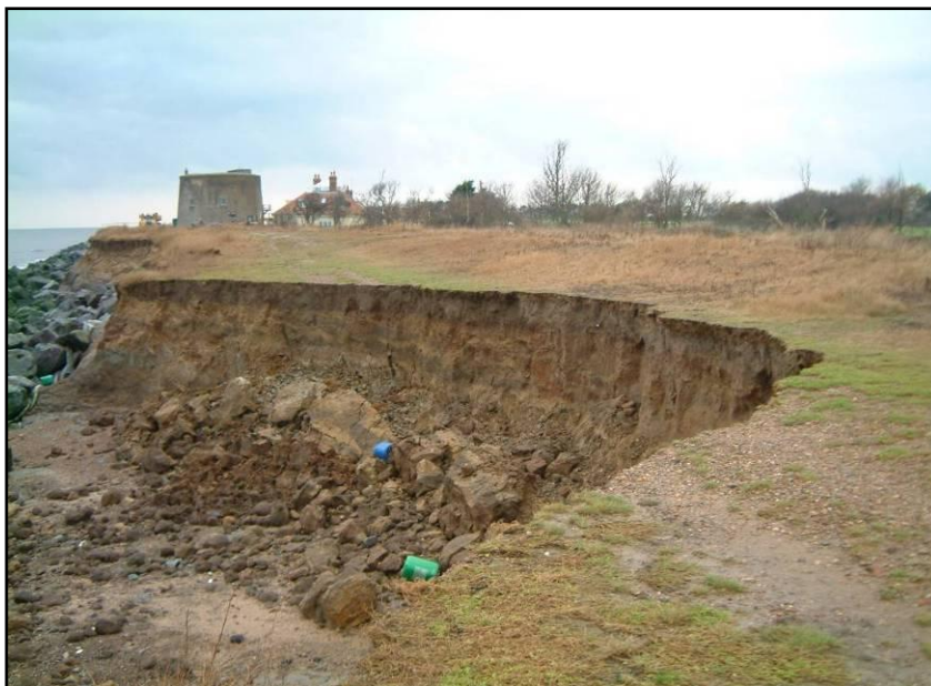
Figure 4. Erosion of Environment Agency flood defence embankment (Nov 2004). Source: Terry Oakes Associates Ltd
