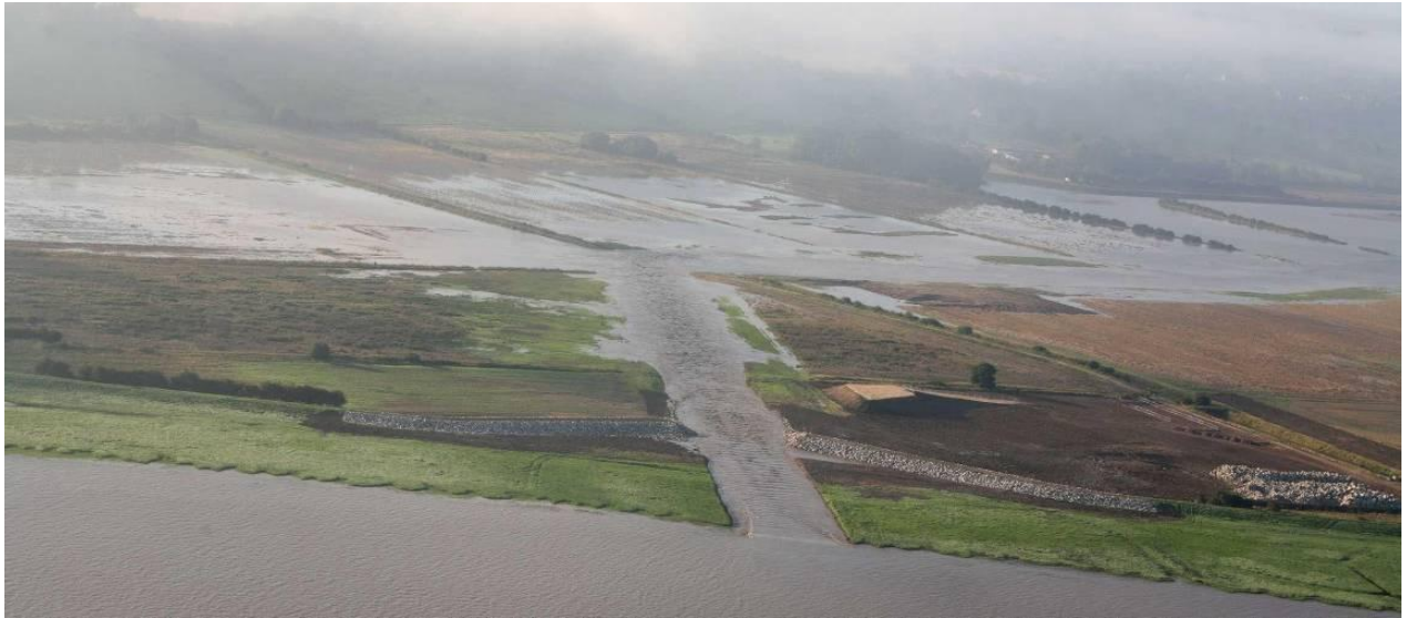
Figure 4. Site breach, Copyright: Environment Agency
