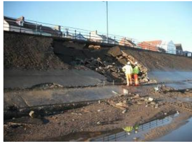
Figure 17. Defence Failure at Redcar.
