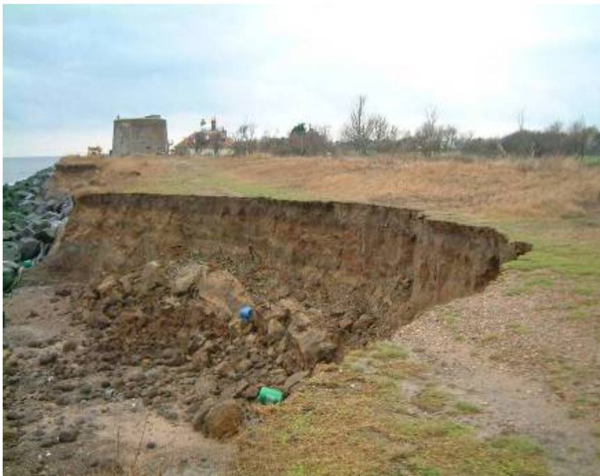
Figure 5. Erosion of Environment Agency flood defence embankment (Nov 2004).
