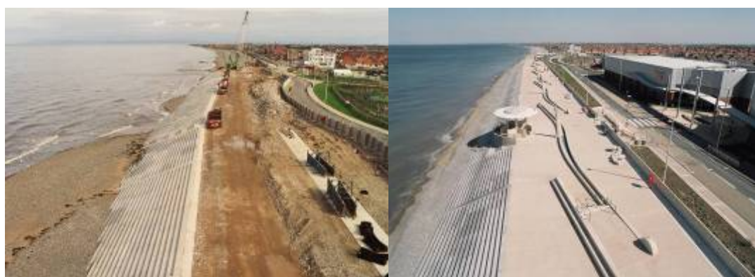
Figure 3. During (left) and after (right) construction of part of the Cleveleys scheme.
