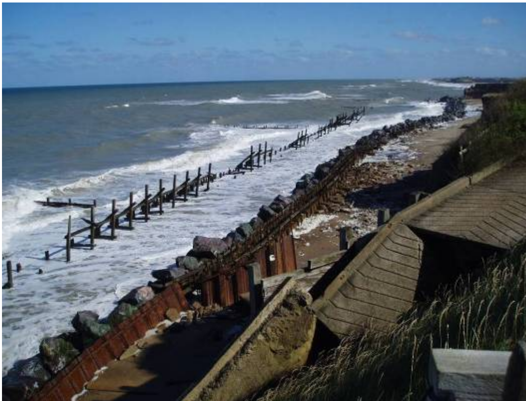
Figure 7. View of dilapidated defences, post construction of rock revetment (2007)
