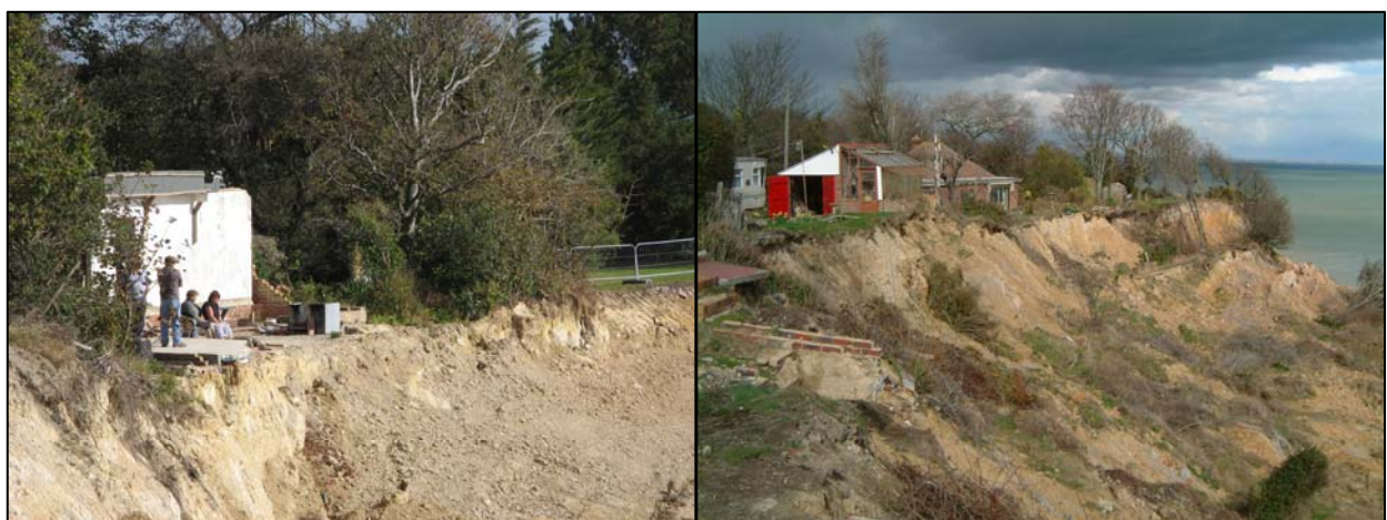
Coastal erosion at Fairlight Cove an example of a no active intervention scenario. Source: Terry Oakes Associates
