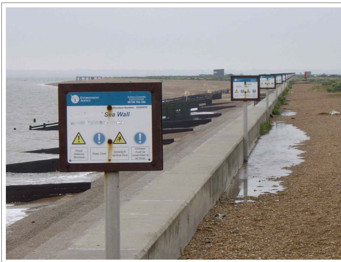
Photograph 6.1 Sea wall out of town but along a tourist coastline and near to an advertised tourist site.
