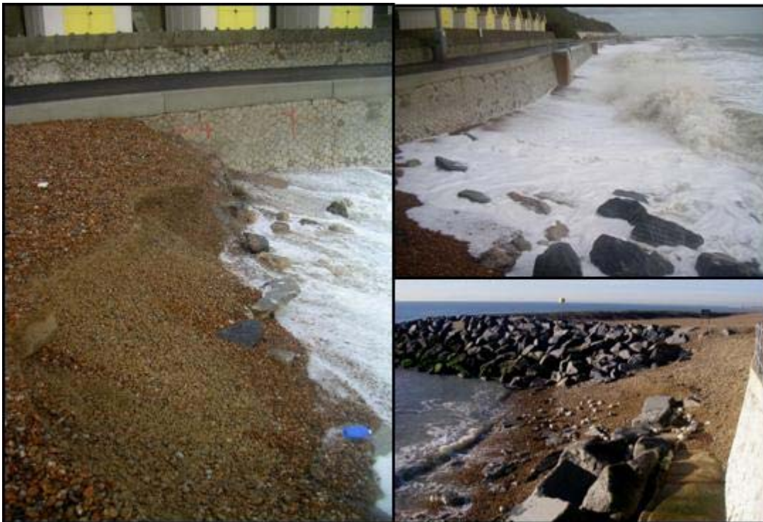
Figure 39 Photographs showing the dramatic storms and subsequent erosion east of groyne B (cell 5).
