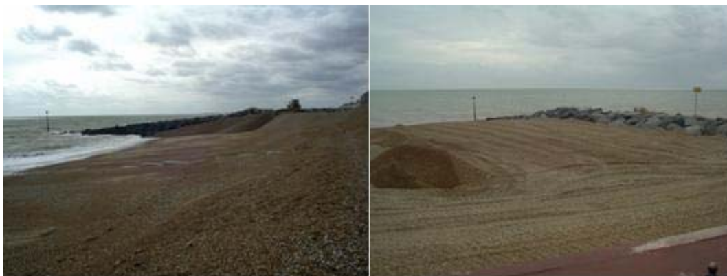
Figure 36 Stockpile being placed at Stade Street, in the shelter of groyne A
