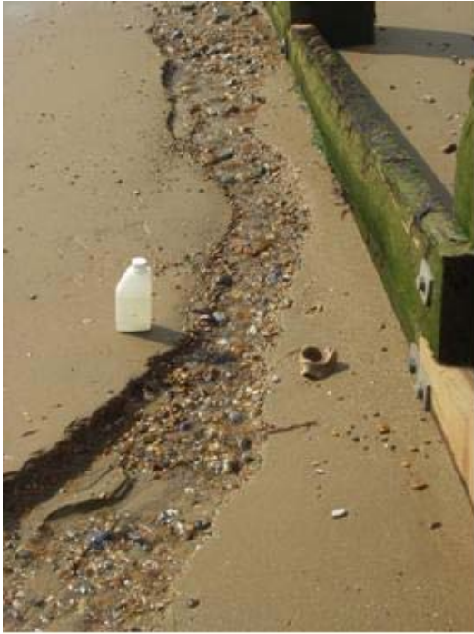
Figure 18 Exfiltrating water following high tide
