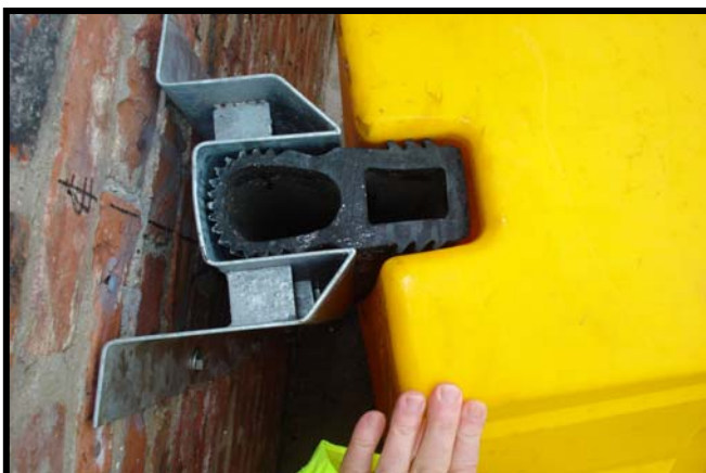
Figure 6: One of the bespoke steel channels used to attach AquabARRIER units to walls at Clementhorpe
