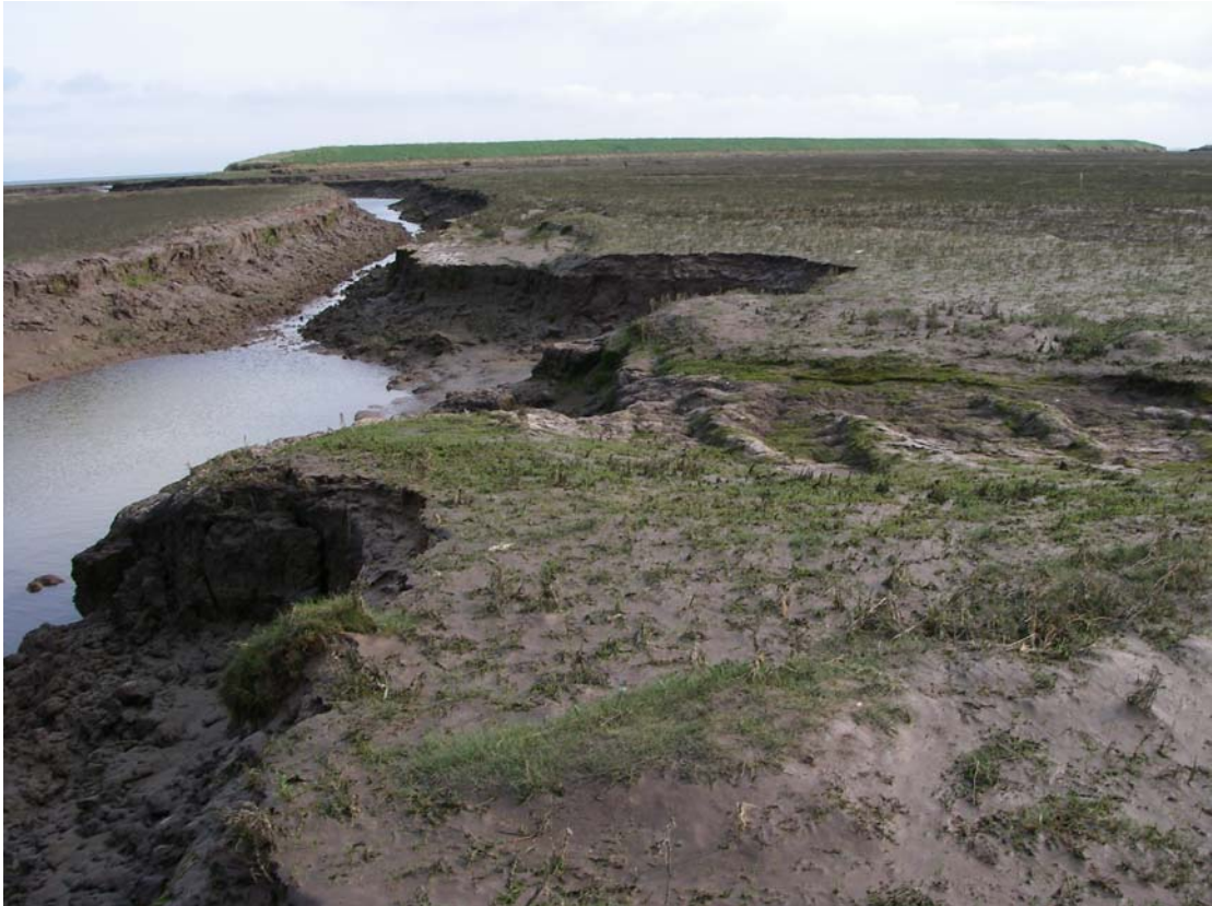
Photo 9.5 Creek side erosion of excavated creek inside MR, looking towards central breach. Photo: Sue Brown, April 2007
