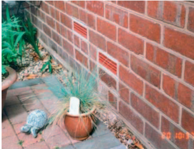
Figure 6.11 Periscopic air vent (courtesy Severn Trent Water)
