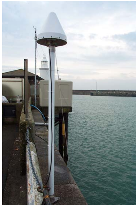
Figure 2.5 Photograph of a GPS antenna and monument: the photograph shows the equipment installed at the Dover tide gauge.
