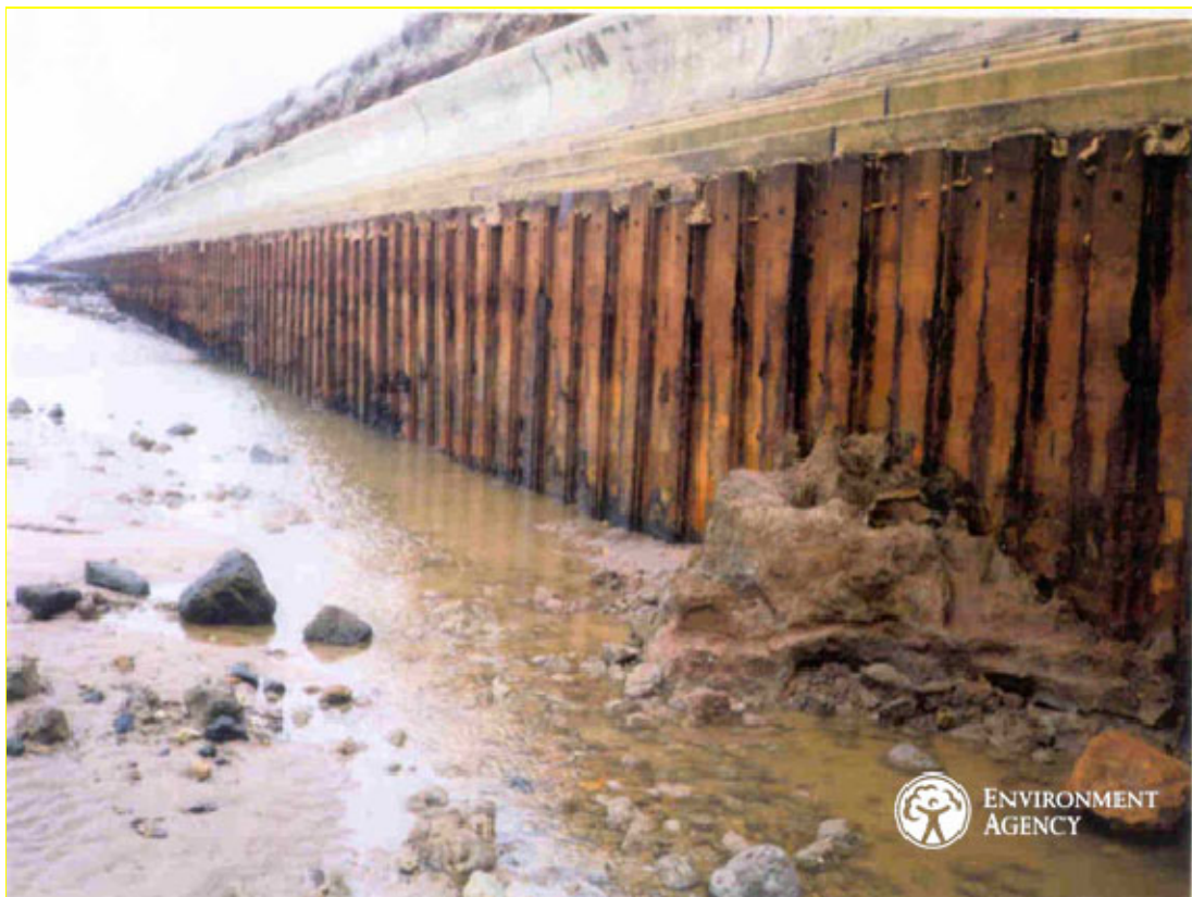
Figure 5.1 Exposure of Sheet Piling at the Toe of a Seawall
