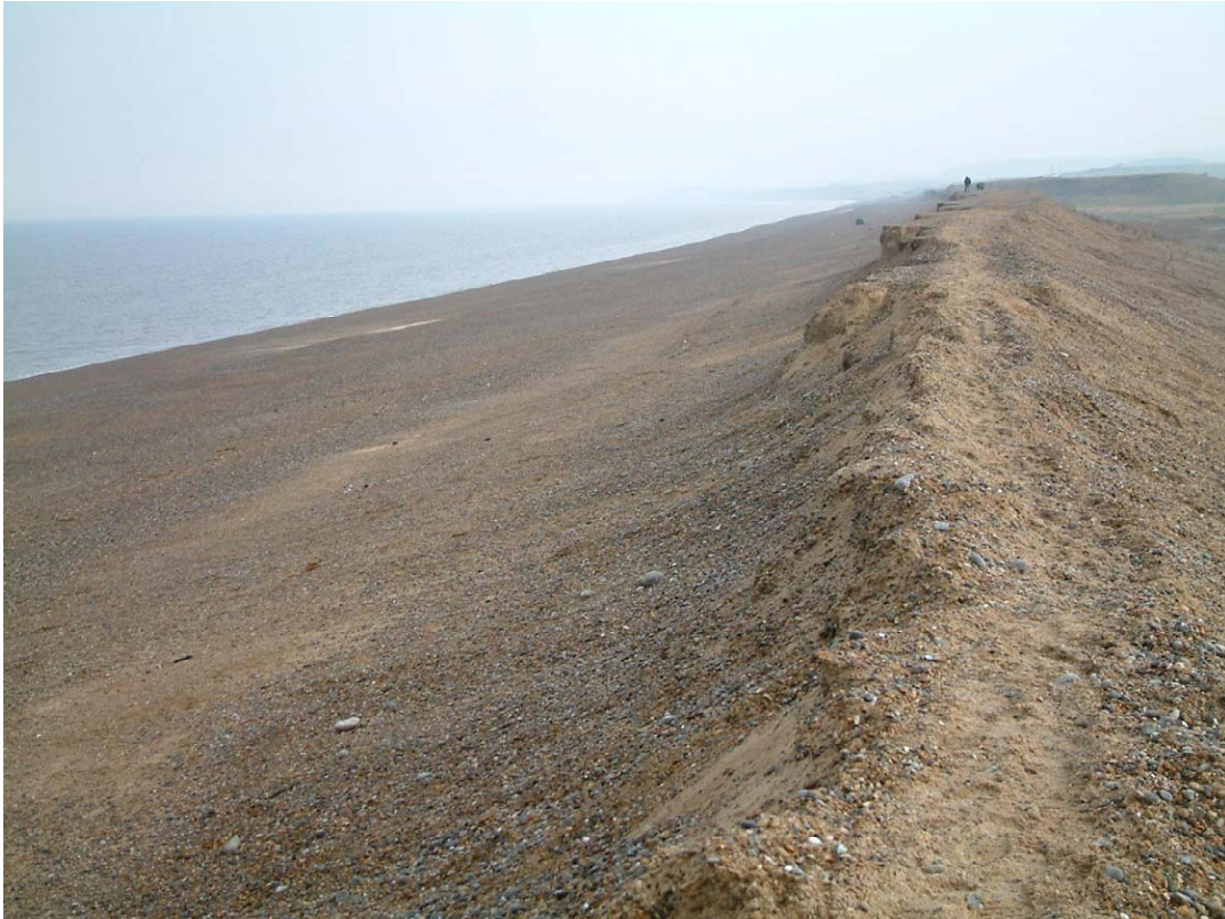
Plate 6.3 Brittle cross shore profile developed as result of re-grading with mechanical plant (Bradbury)
