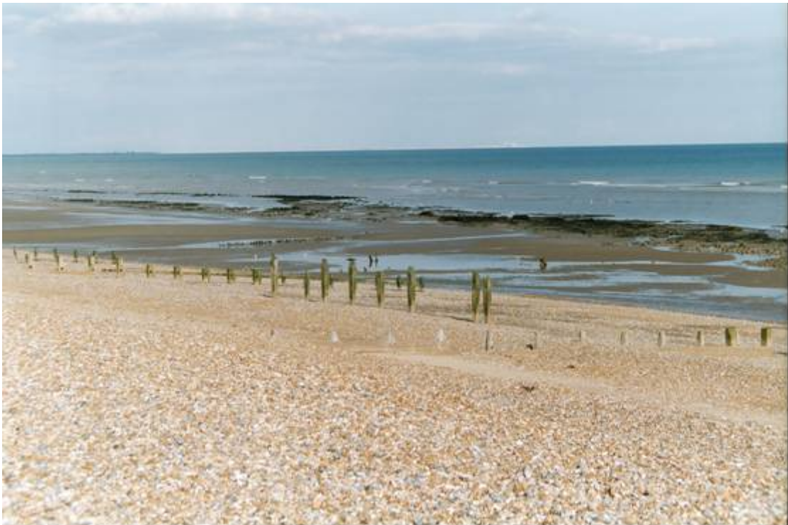
Plate 5.37 Erosion of the lower foreshore
