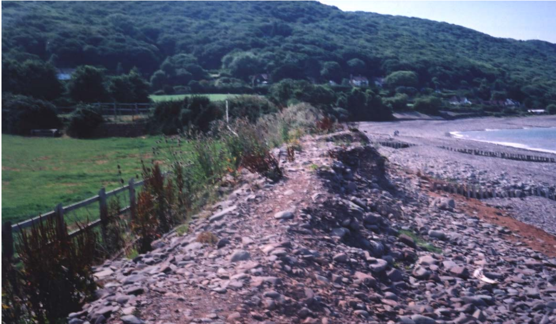
Plate 2.1 Porlock barrier, Somerset. A vulnerable section that experienced crest cut-back, 3 rd September 2001 (Cope, 2004)
