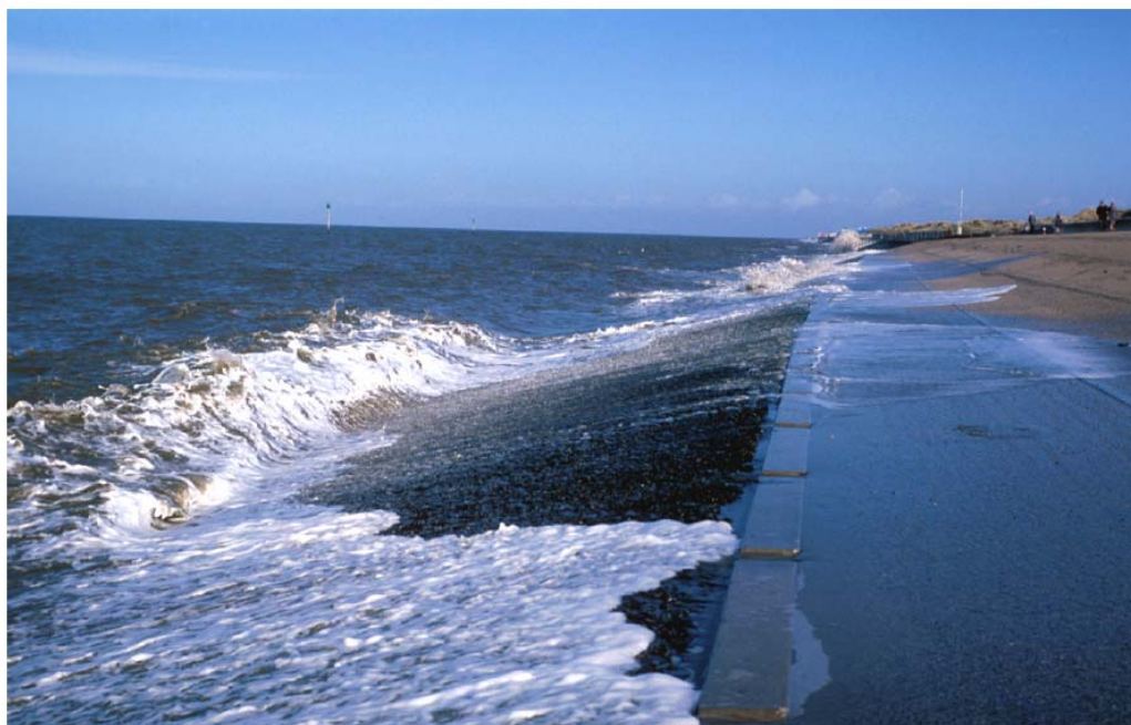
Plate 3.2 Wave run-up and overtopping of a sloping seawall, Prestatyn (Dodd et al. , 2000)
