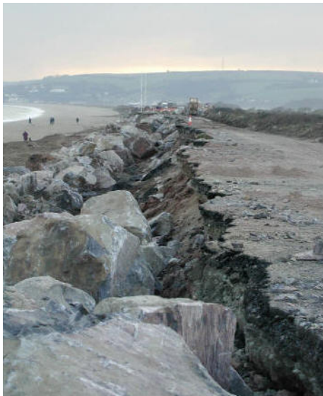
Plate 4 Erosion of Slapton coast road - 1999 (Peter Wagstaff)
