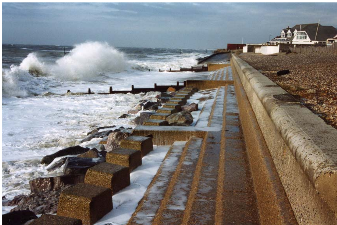
Plate 9 Concrete unit and rock fillet, Selsey Bill, West Sussex, 2006
