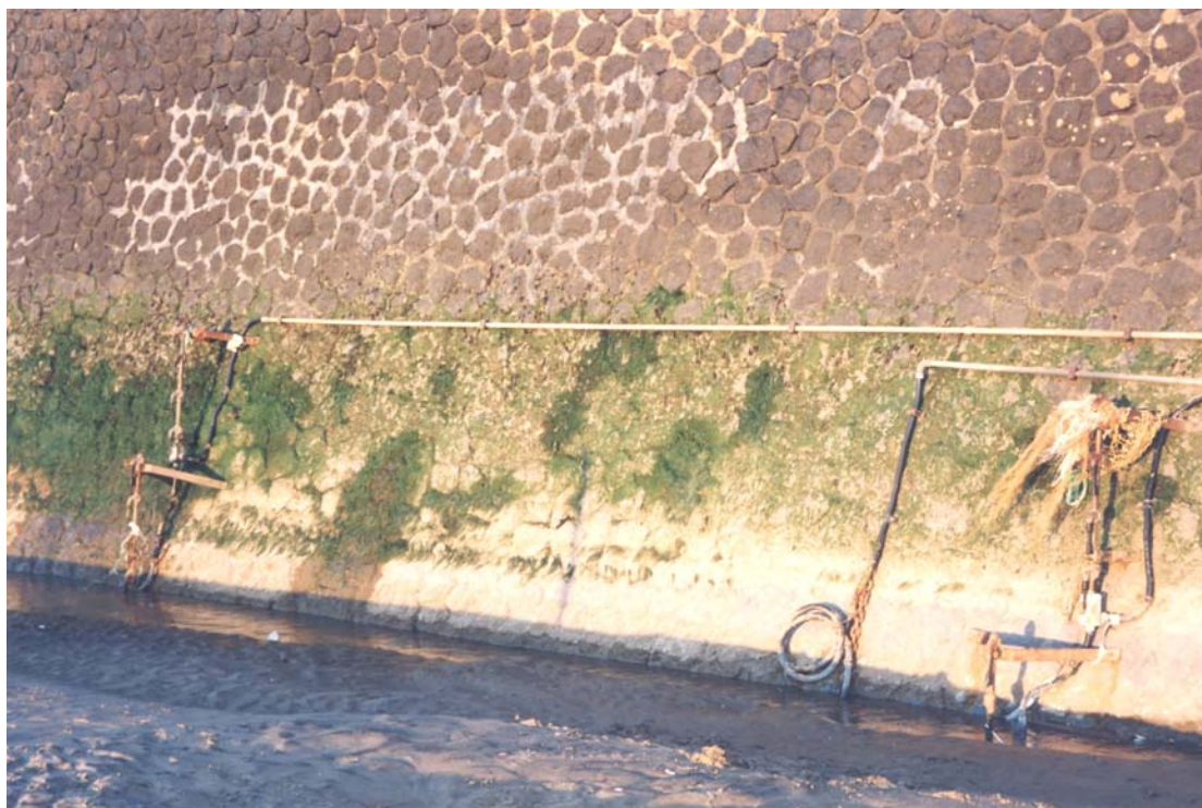
Plate 5 Scour monitors B, on left, and A, on right, with cable to offshore monitor C in the centre
