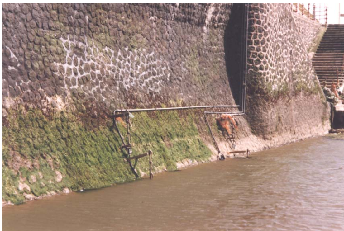
Plate 6 Scour monitors B and A on seawall showing position relative to steps
