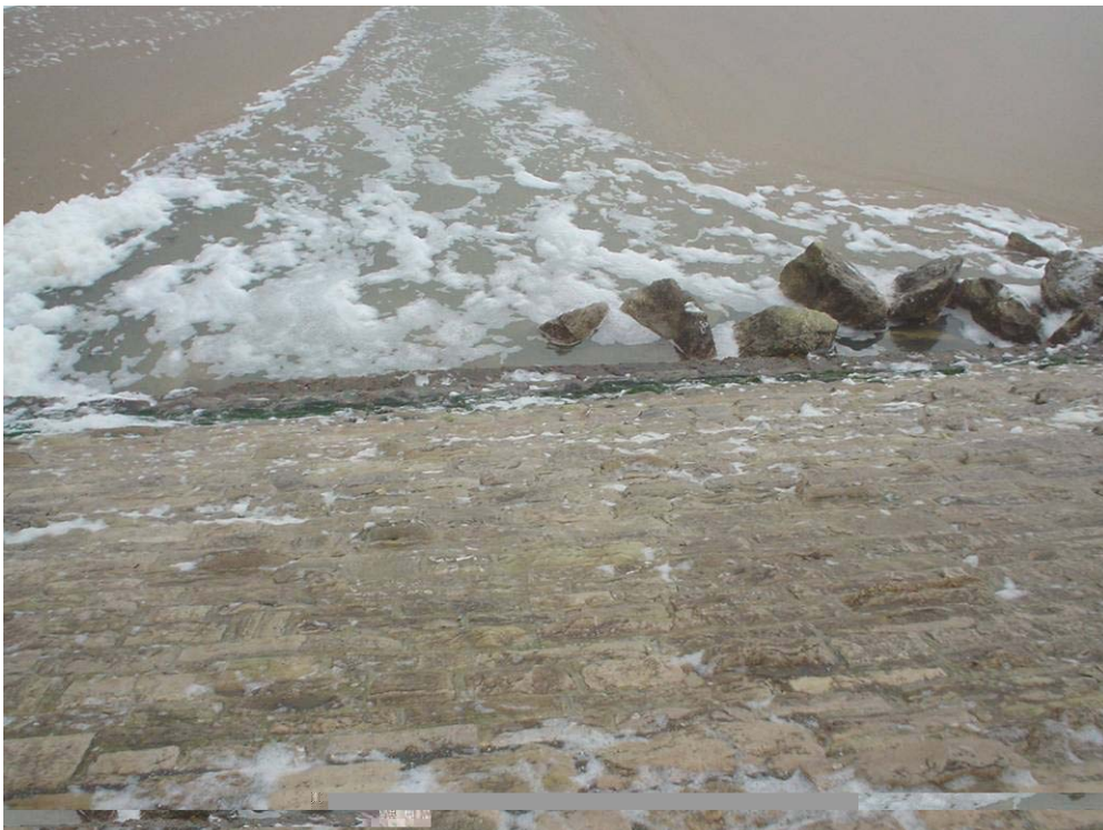
Plate 16 Fisherman's Walk on 11 January 2005. Low beach level revealed rocks at toe at approximately 0mODN elevation at toe of wall.
