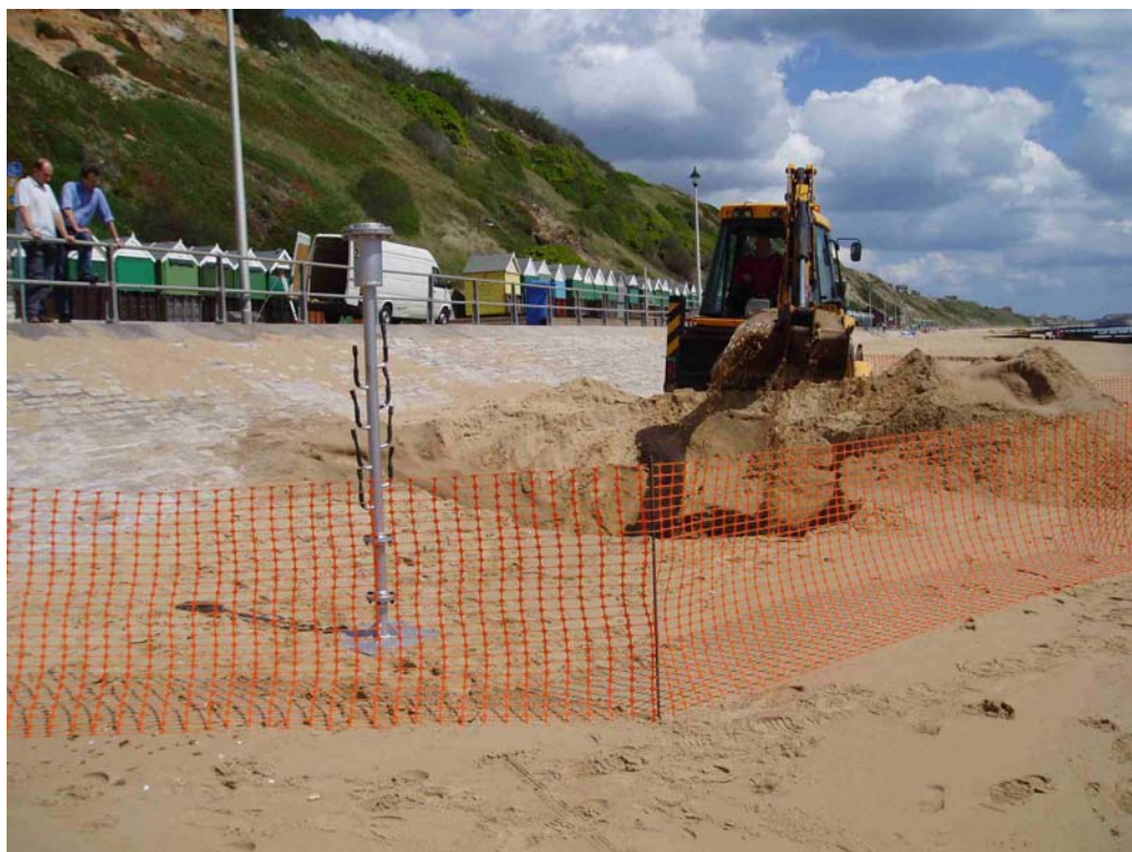
Plate 22 Scour monitor about to be deployed vertically at toe of sloping seawall by JCB on 9 May 2005.
