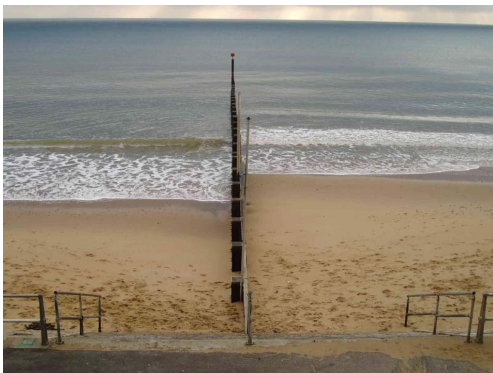
Plate 9 Groyne G32, showing wider beach on right (western) side (21 December 2004). CCO profile 5f00410 and Bournemouth Borough Council profile A8 marked by yellow paint to left of steps.
