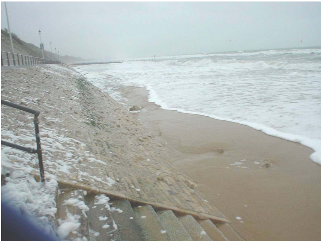
Plate 18 Beach lowering at toe of seawall at Fisherman's Walk on 11 January 2005.
