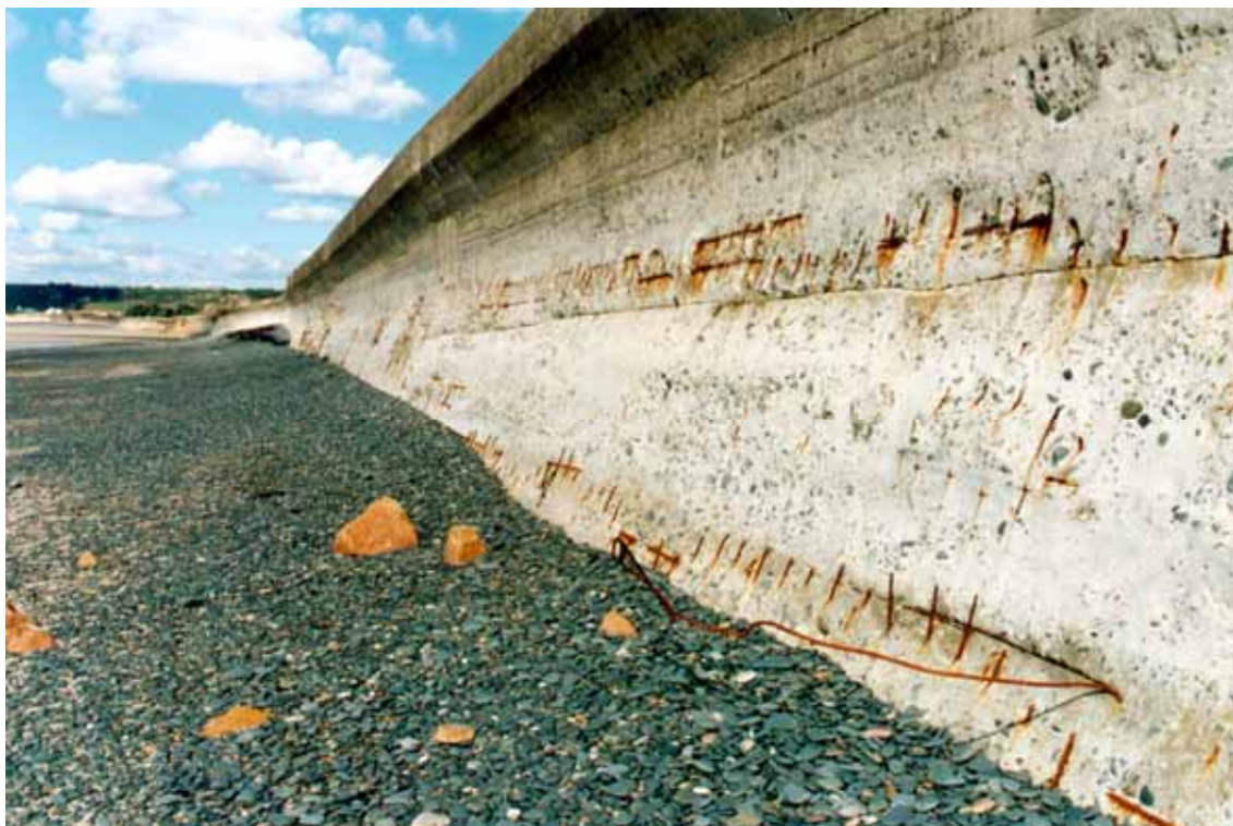
Figure 3.2 An example of hydrodynamic abrasion exposing steel reinforcement in a concrete seawall
