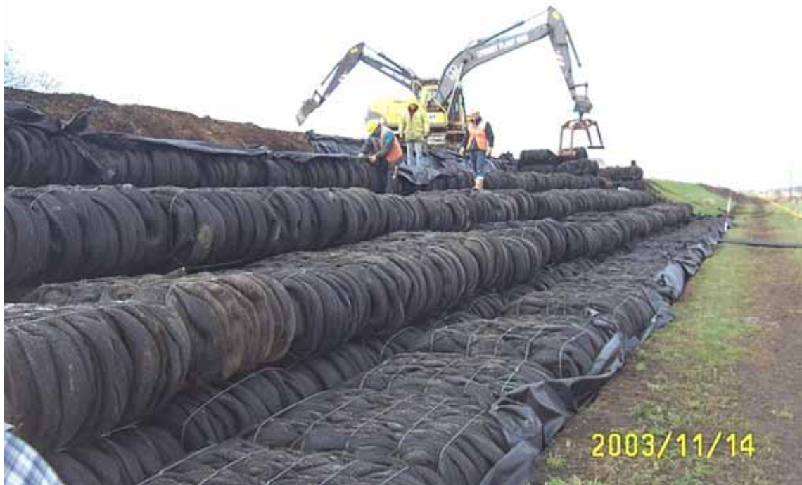
Figure 5.32 Construction of the River Witham Flood Embankment, near Lincoln (courtesy Environment Agency)
