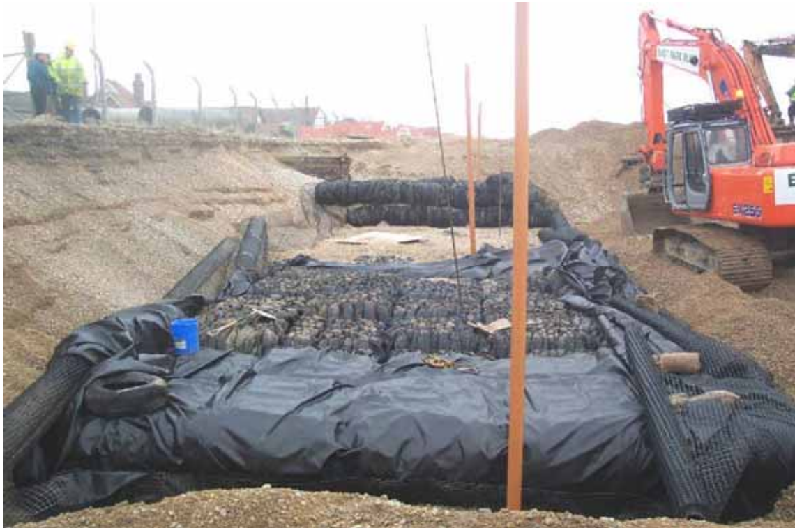
Figure 5.30 Pevensey Bay project near completion with sampling pipes in situ. (courtesy PCDL)
