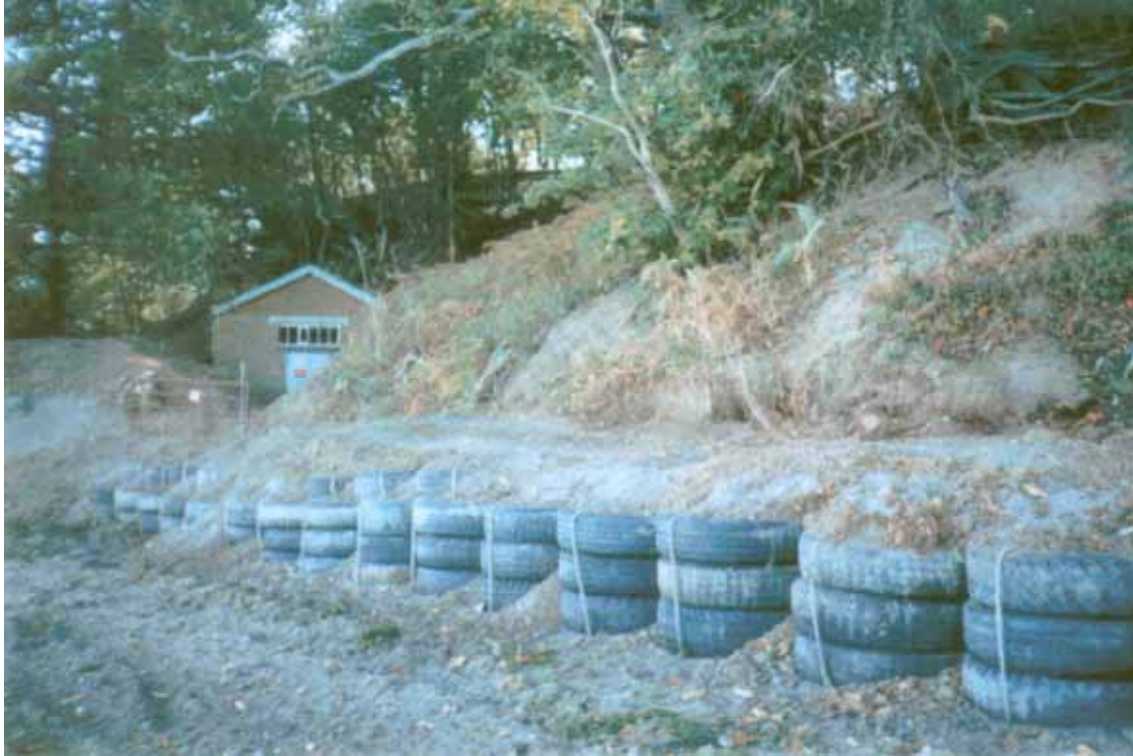
Figure 5.7 The Copperas Wood defence soon after construction (courtesy of Sorrell Flood Protection)
