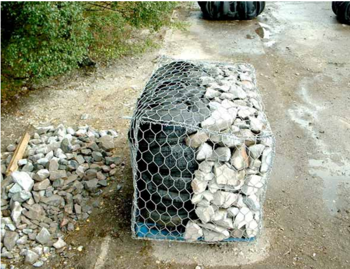
Figure 5.39 Tyre bale as rear fill for gabion box (courtesy Northern Tyre Recycling)
