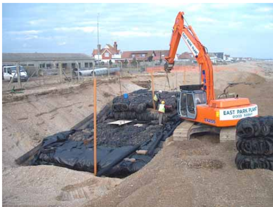
Figure A8.12 Construction of the tyre bale block in Pevensey Beach (Courtesy of PCDL)
