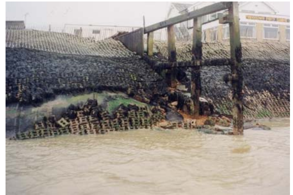
Figure 2 Failure of the toe of the channel lead to collapse of this revetment
