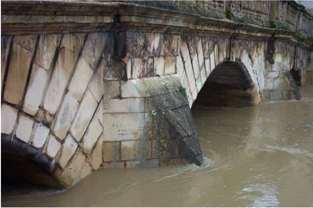
Plate 5 – Flood flows at arch bridge – River Cam
