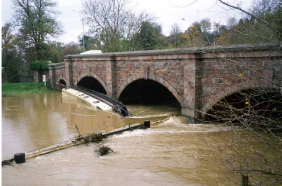
Plate 3 Bridge blockage by boat – River Soar
