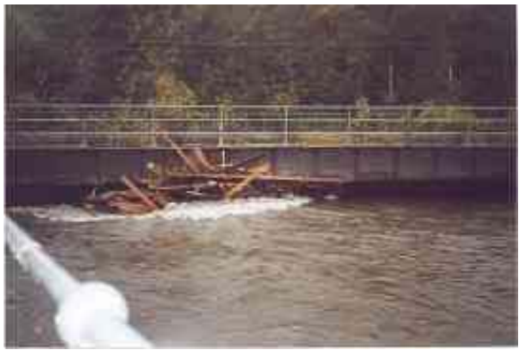
Collection of floating debris at a bridge soffit during flood.
