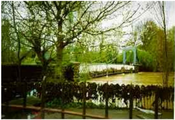
Partial blockage of the railings of a footbridge.
