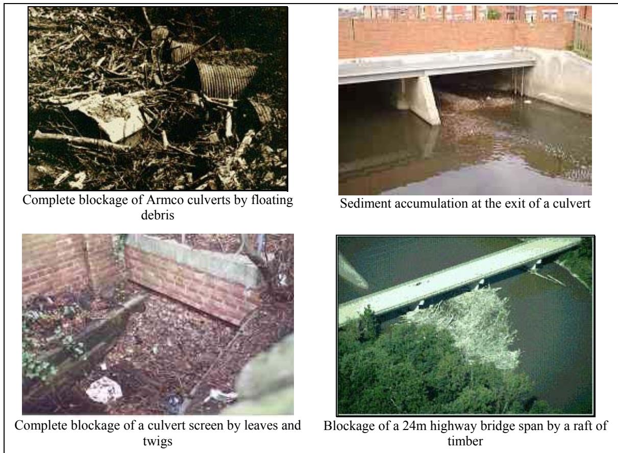
Figure 3.6: Examples of blockage
