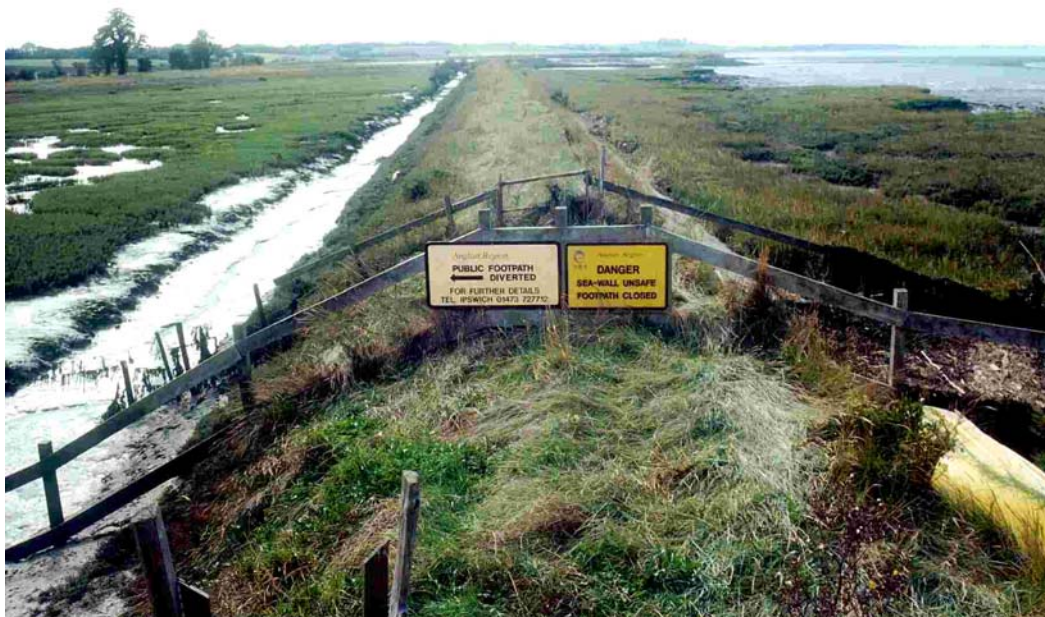
Figure D.14 Orplands sea wall post breach; looking westwards along seawall from eastern end of site, showing badly eroding saltmarsh outside of the breached sea wall (to the right) and retreat site to the left of the picture (source: Environment Agency)
