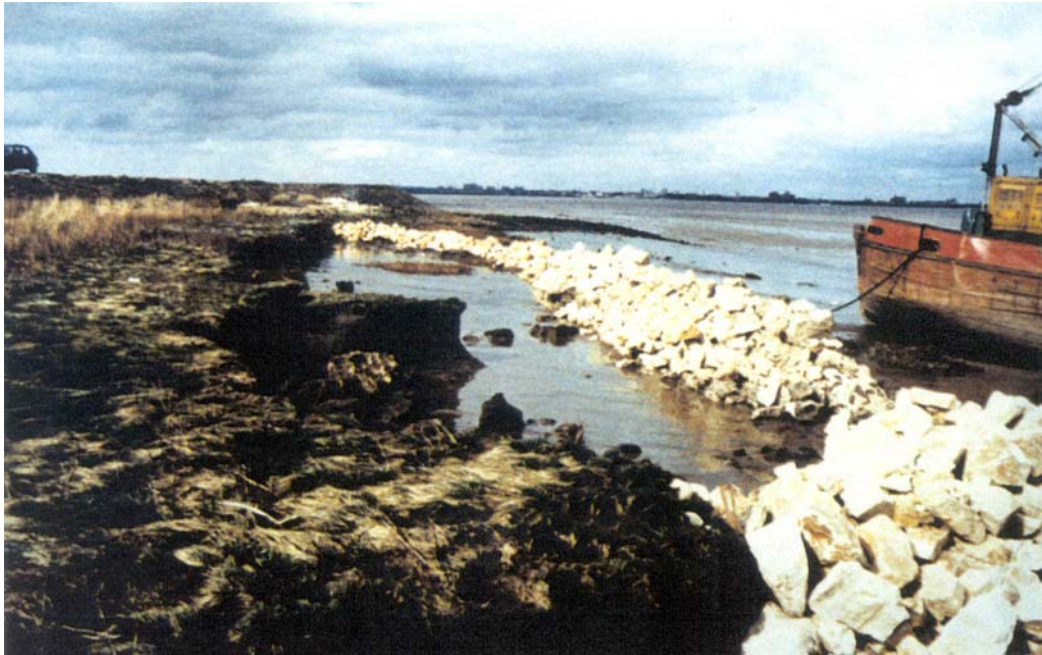
Figure D.11 Construction of the rock beach sill, Goxhill on the Humber (from Toft et al., 1995)
