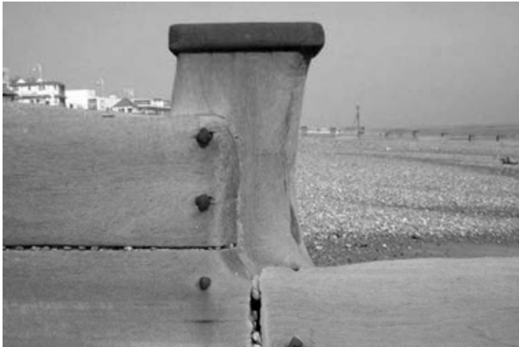
Figure 8.4a. Abraded timber groyne pile (courtesy HR Wallingford)
