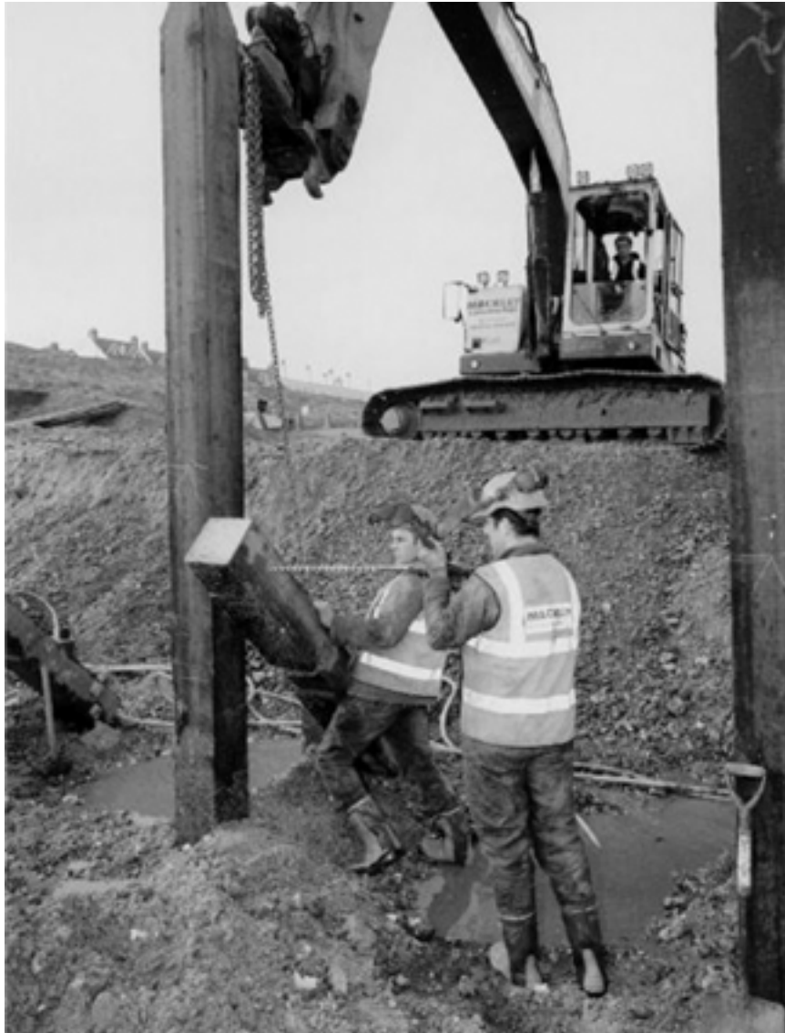
Figure 7.10. Fitting ties to a pile for a timber groyne (courtesy Mackley Construction)
