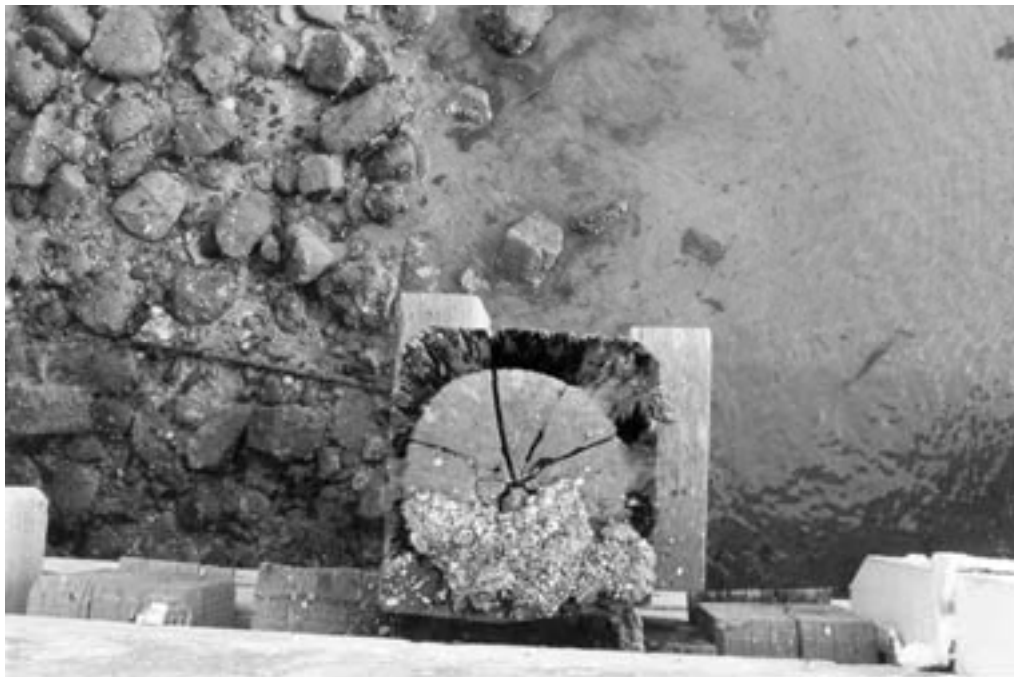
Figure 7.8. Plan view of a greenheart pile approximately 100 years old. The outer perishable sapwood has eroded, leaving the cylindrical durable heartwood clearly visible (courtesy TRADA Technology)
