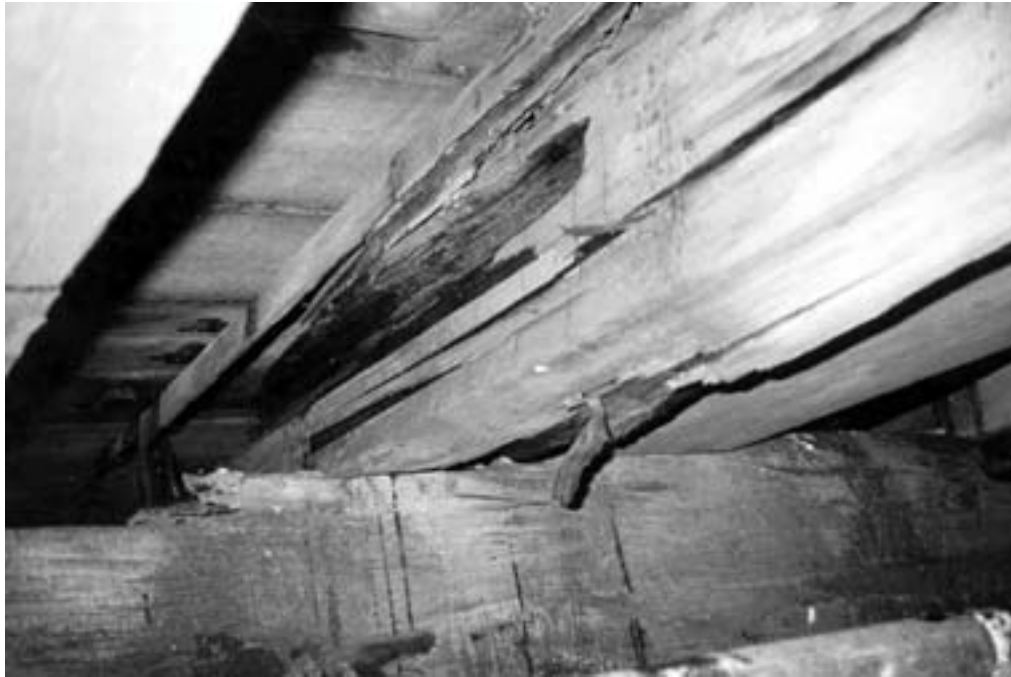
Figure 9.1. Advanced fungal decay in primary and secondary beams (courtesy John Williams)
