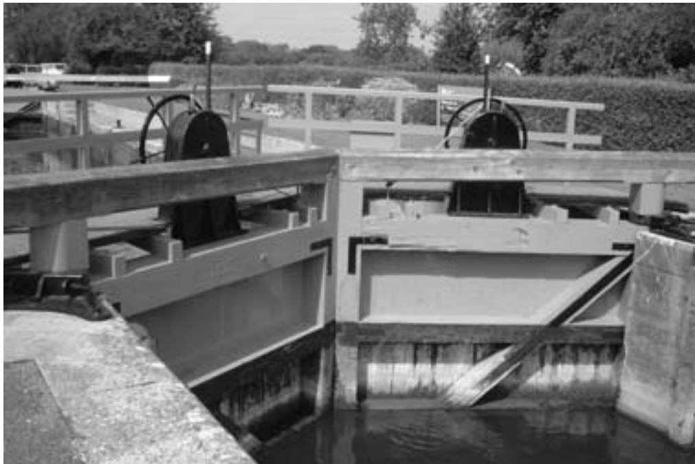
Figure 8.25. Timber lock gates on an upper reach of the River Thames (courtesy HR Wallingford)
