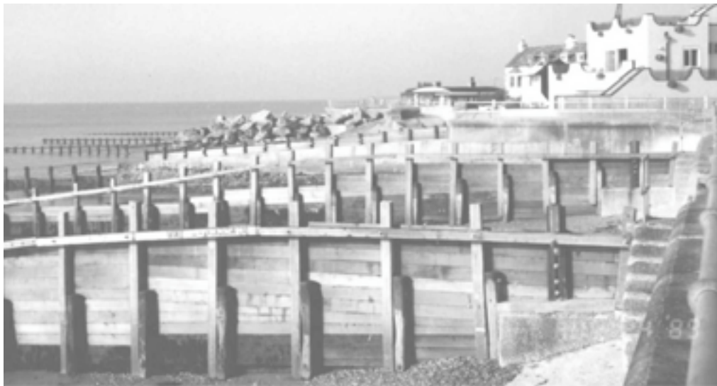
Figure 8.5. Pile extensions to facilitate reprofiling of a groyne field (courtesy Arun District Council)
