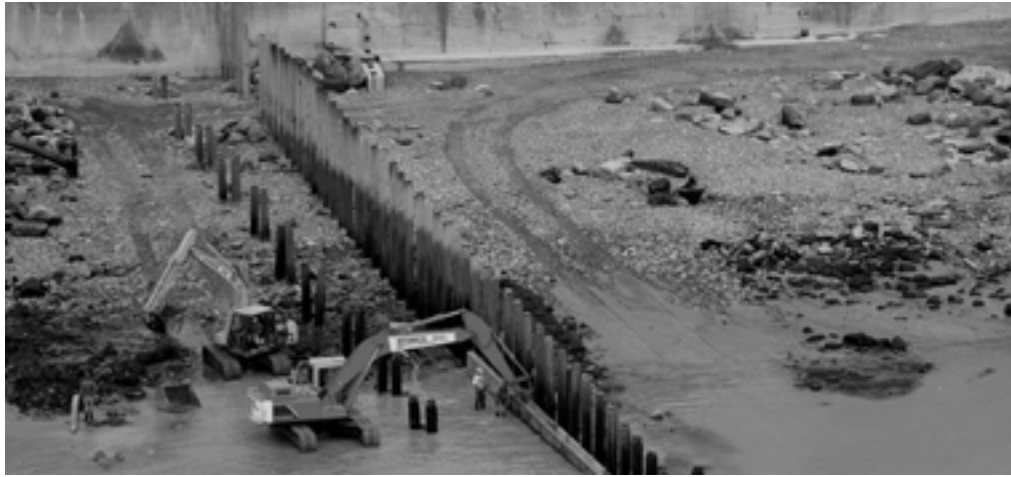
Figure 7.2. Groyne construction work at Eastbourne, working up the beach with the rising tide (courtesy Mackley Construction)
