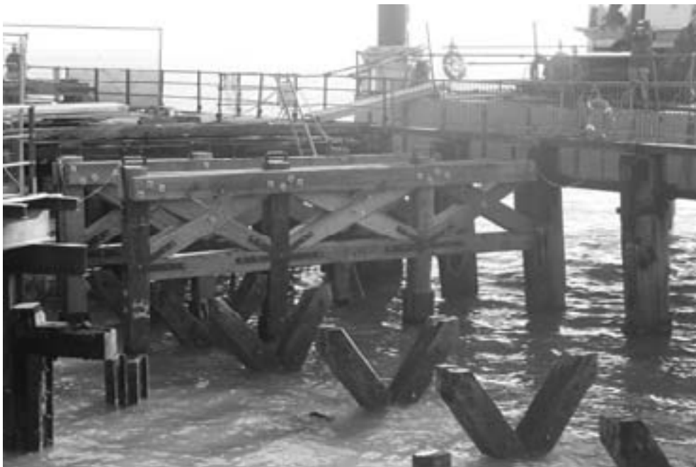
Figure 10.1. New timber fixed onto old as part of refurbishment of fire damaged Southend Pier (courtesy Southend Borough Council) – see also Section 9.1.6
