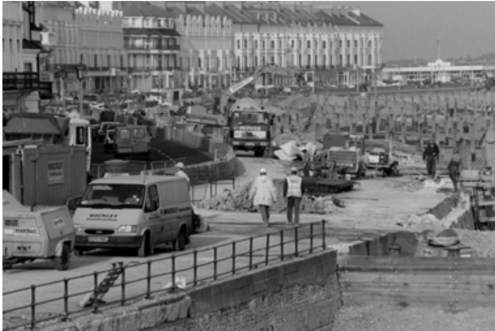
Figure 7.1. Access and interface with the public during reconstruction of timber groynes at Eastbourne, East Sussex (courtesy Mackley Construction)
