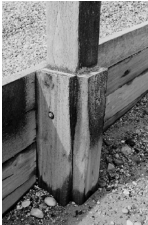
Figure 8.4b. Rubbing pieces protecting the pile on a timber groyne (courtesy HR Wallingford)
