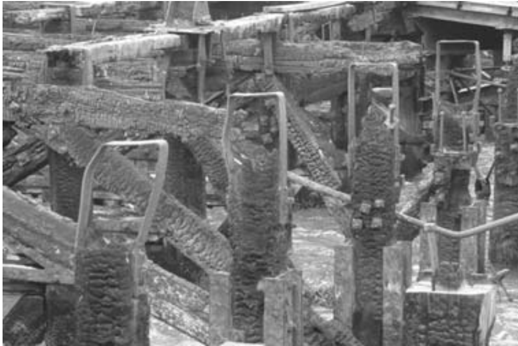
Figure 9.2. Fire damage down to the water line of Southend Pier (courtesy Ecotimber Ltd.) – see also Section 10.2
