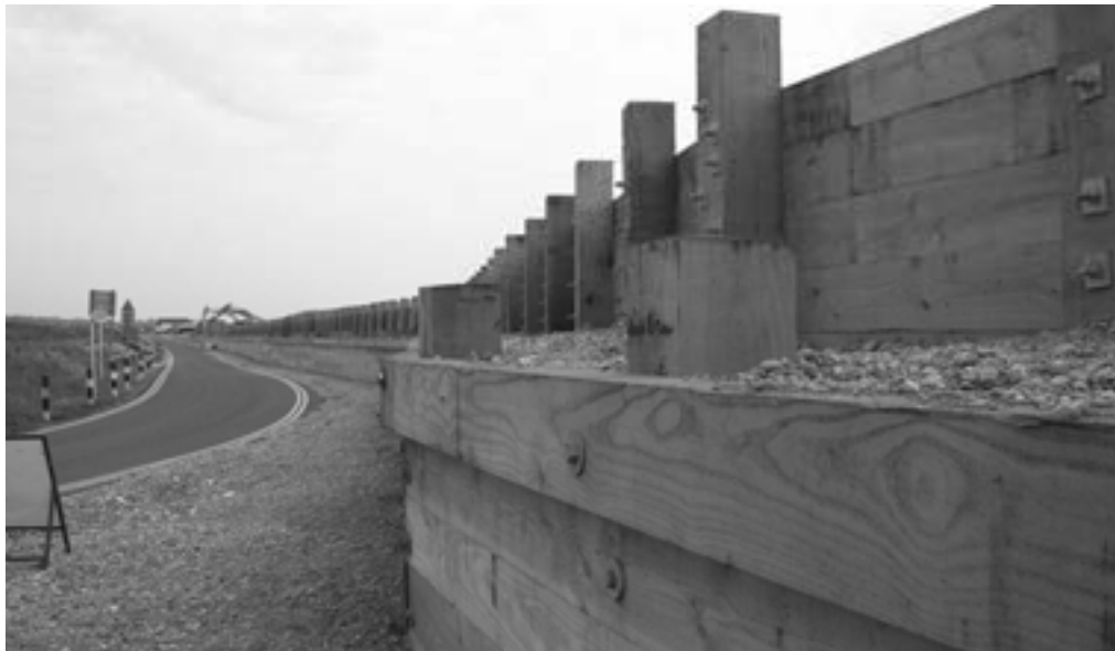
Figure 8.10. Breastwork at Pevensey, East Sussex, retaining substantial shingle beach, to right of photo (courtesy Aitken & Howard Ltd.)
