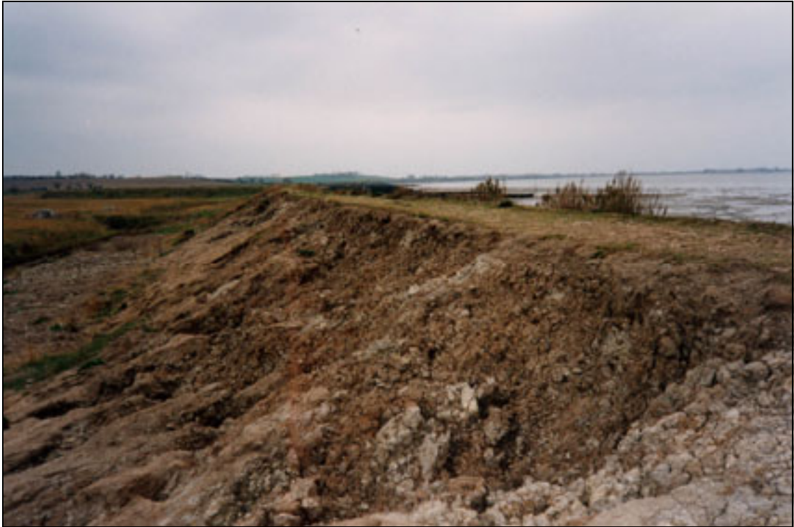
Plate B3.14 Erosion of outward face due to overtopping
