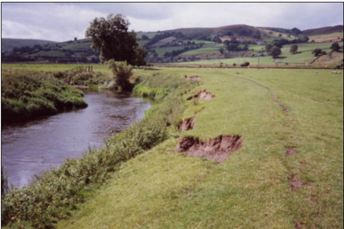
Plate B3.10 Inward face instability (due to undercutting of embankment toe)
