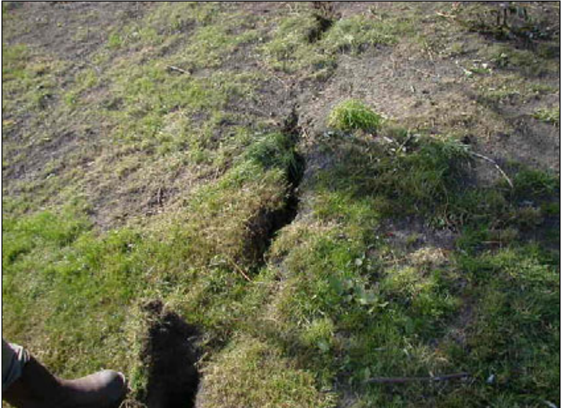
Plate B3.5 Cracking through embankment crest due to rotational failure
