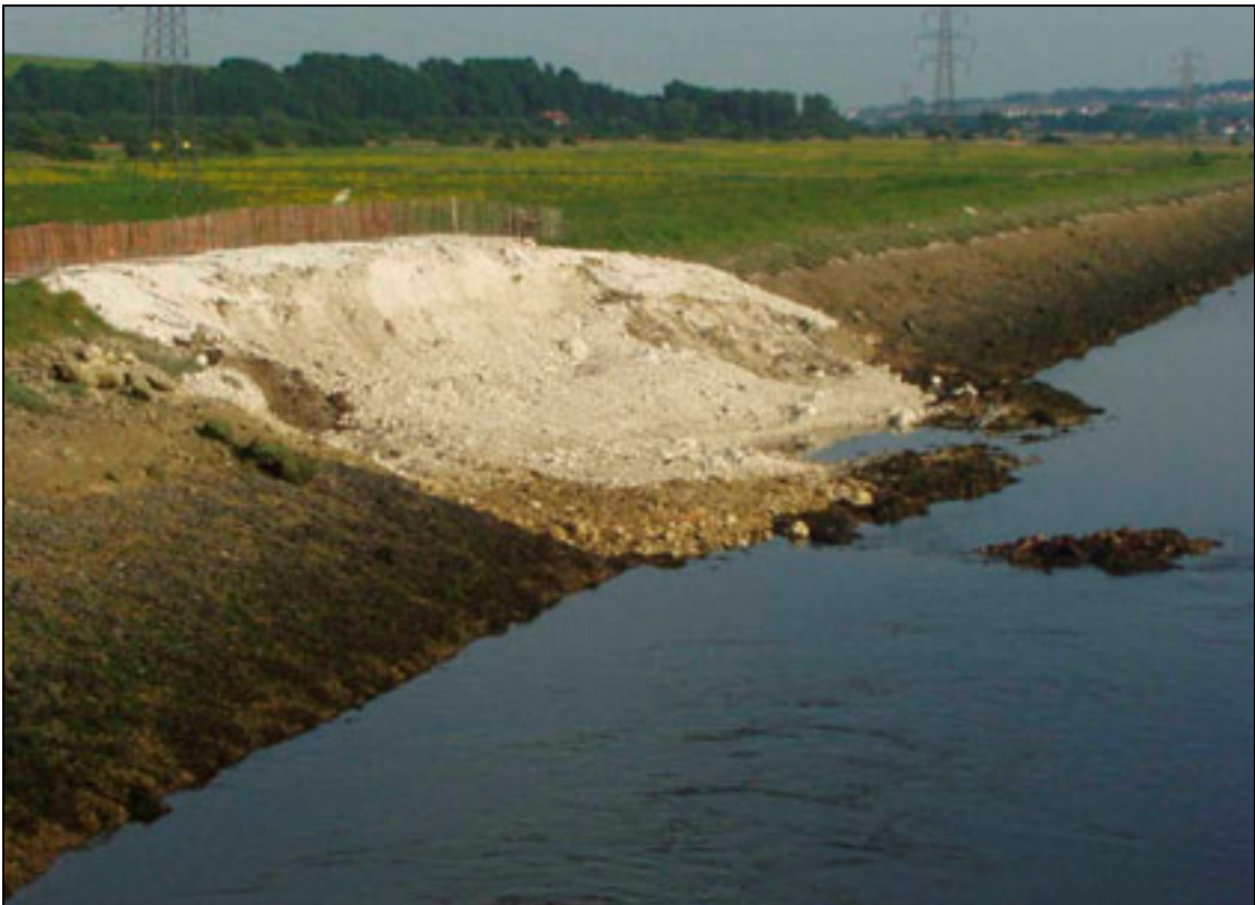
Plate B3.4 Rotational failure through inward face of embankment
