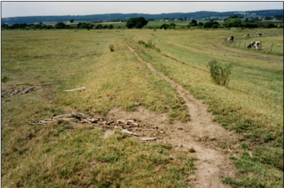
Plate A2.20 Sheep tracks across embankment erode surface protection (grass) and create low spot in defence
