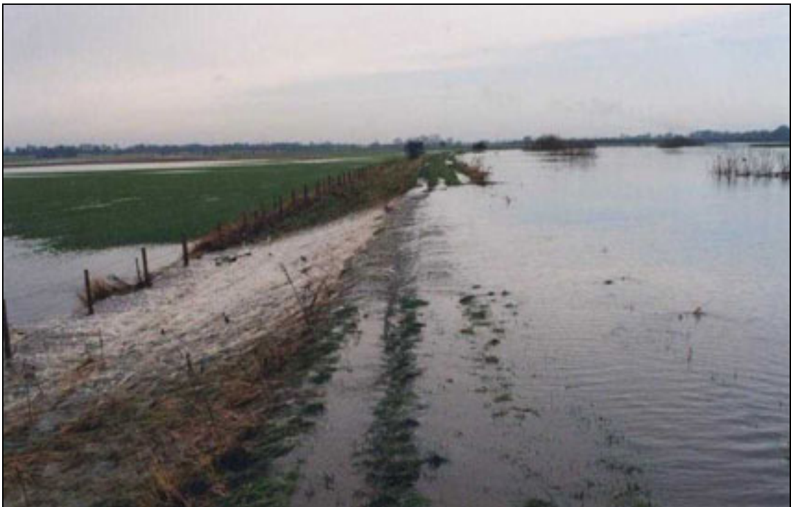
Plate B3.2 Localised overtopping showing dip in embankment crest level
