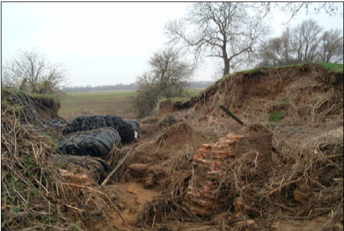
Plate A2.27 Failed culvert running through embankment
