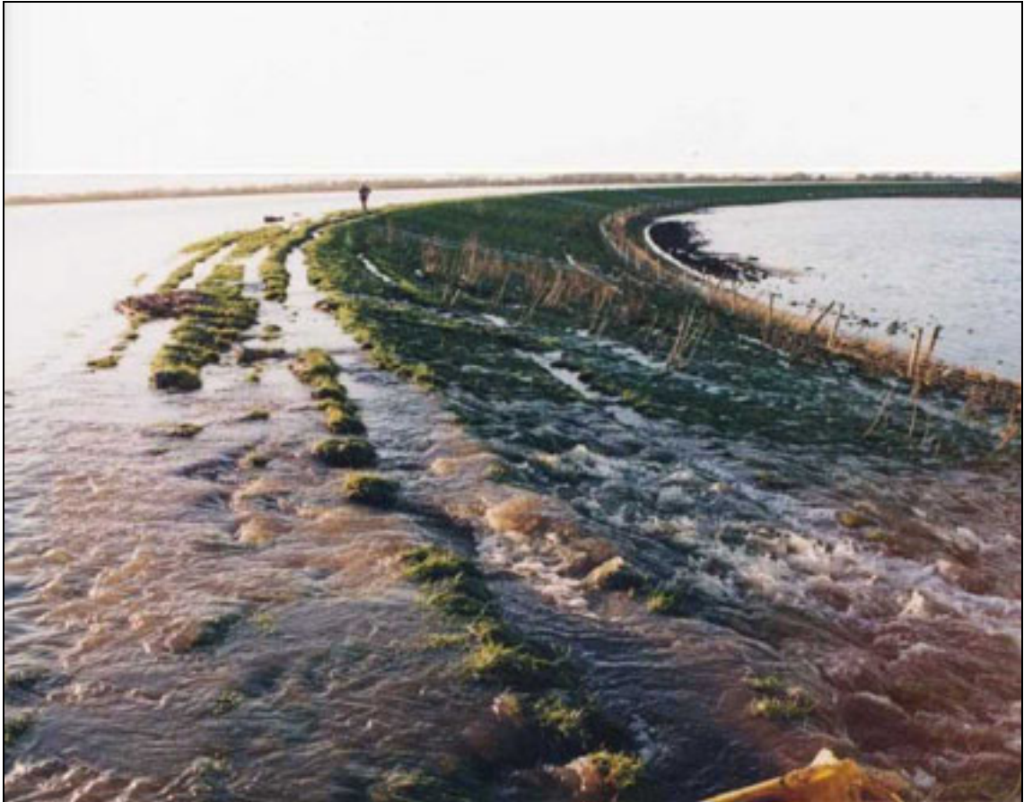
Plate B3.1 Localised overtopping showing dip in embankment crest level
