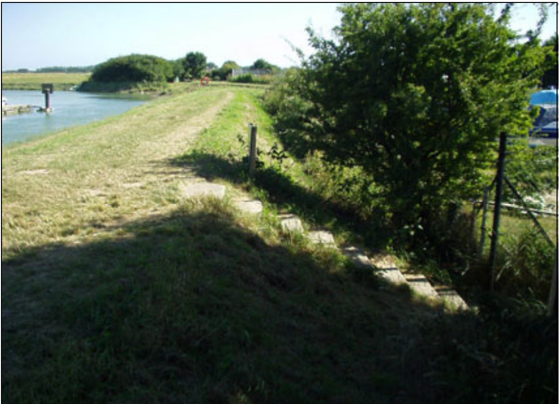
Plate A2.47 Stepped access on outward face of embankment (note erosion of bank adjacent to steps)
