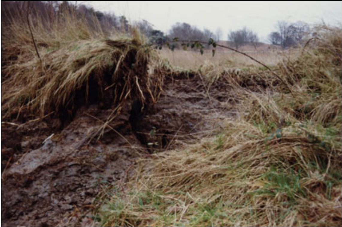
Plate B3.9 Breached embankment on the River Alde (remains of pipe can be seen in centre)
