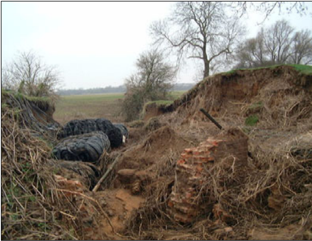
Plate B2.1 Root action contributing towards failure of a culvert through embankment
