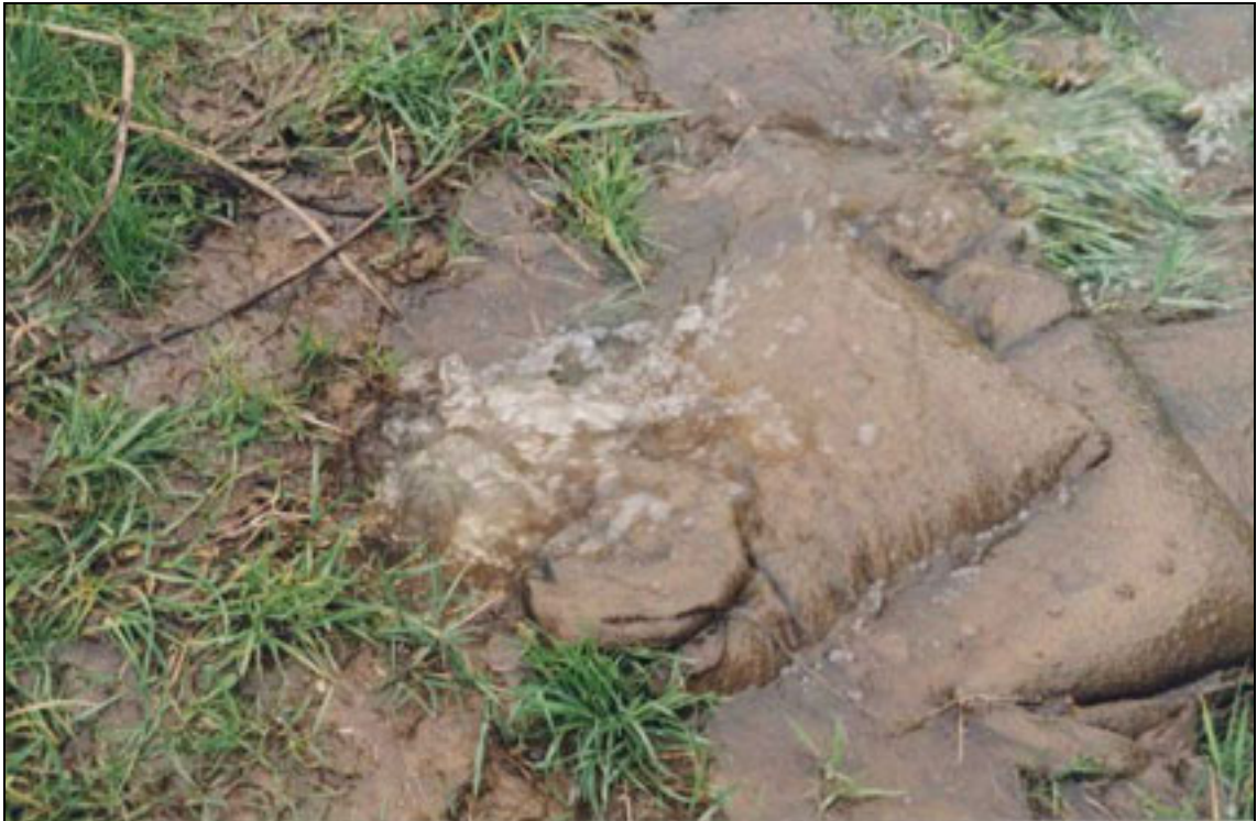
Plate B3.7 Seepage through embankment
