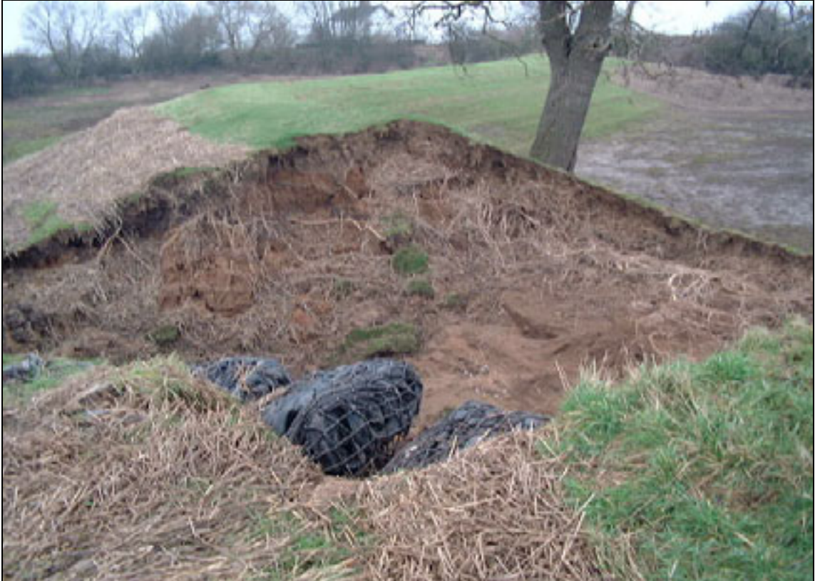
Plate B2.2 Root action contributing towards failure of culvert through embankment
