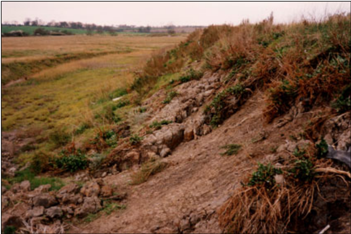
Plate B3.13 Erosion of outward face due to overtopping
