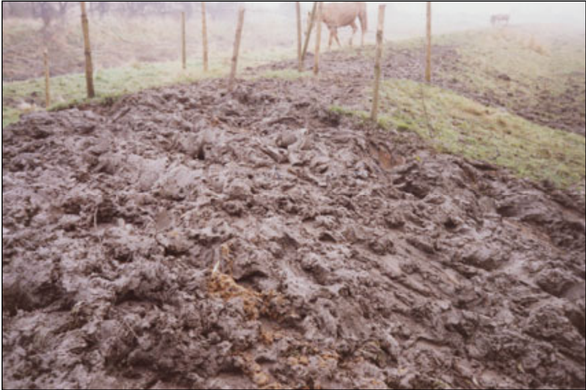
Plate A2.21 Severe surface erosion and soil damage caused by livestock on the embankment during wet conditions
