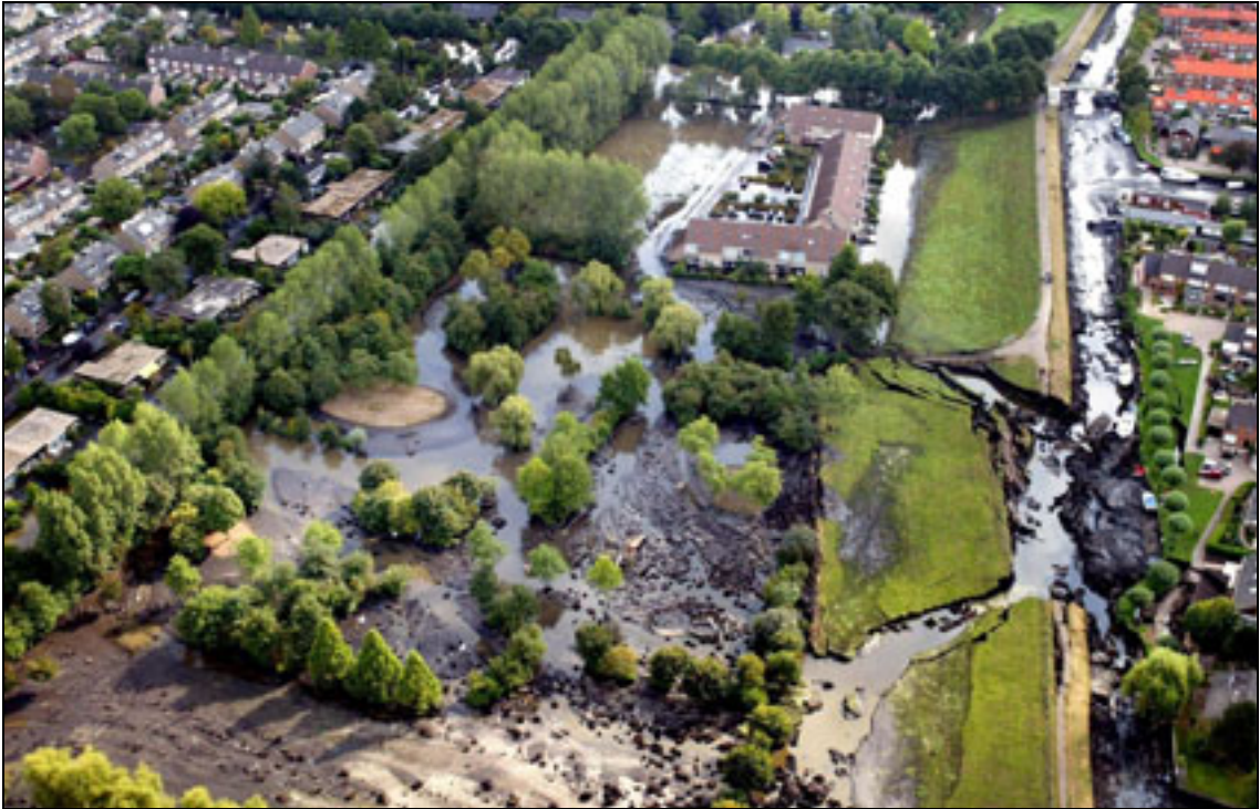
Plate B3.18 Translational block failure of embankment
