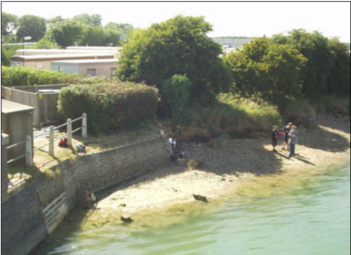
Plate A2.59 Interface between embankment and bridge abutment (note embankment erosion)
