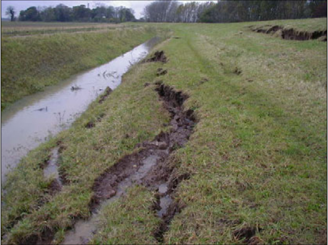
Plate B3.3 Rotational failure through inward face of embankment
