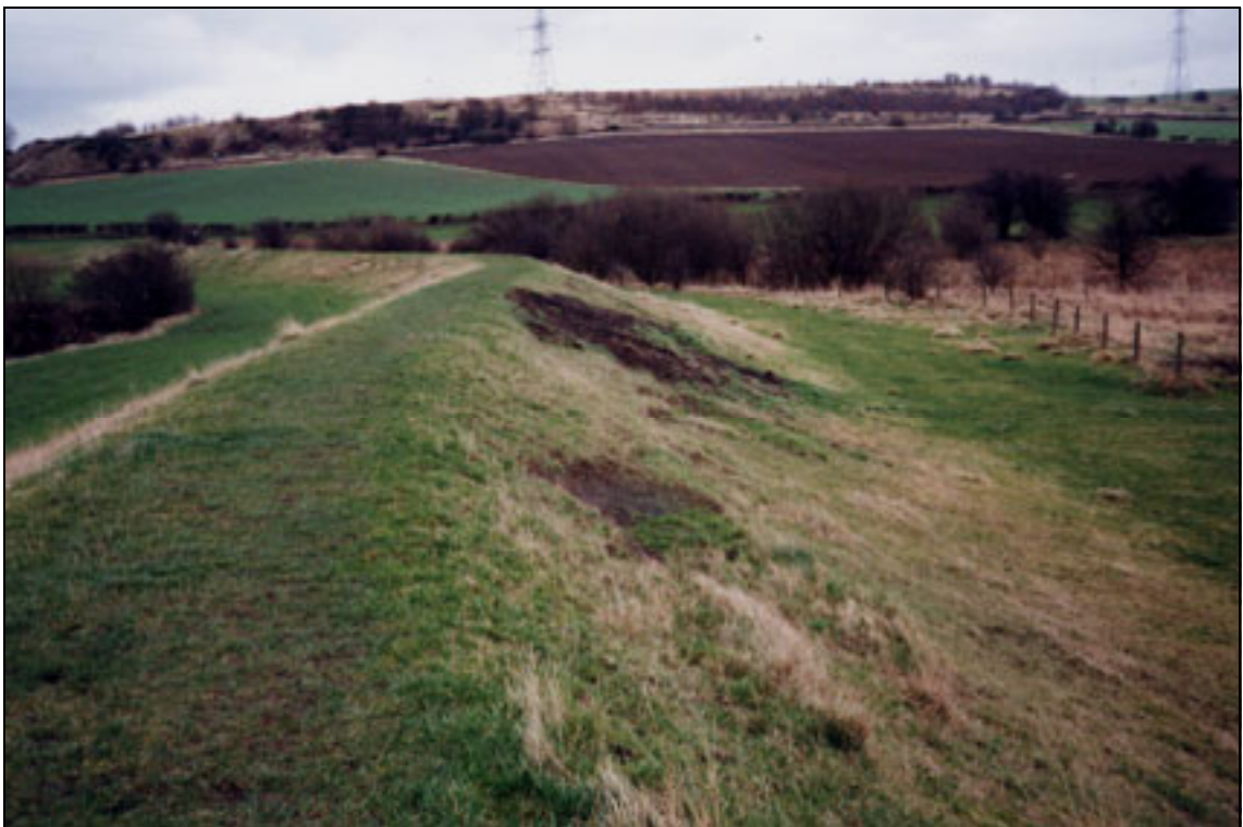
Plate B3.17 Erosion of face due to animal activity / surface instability
