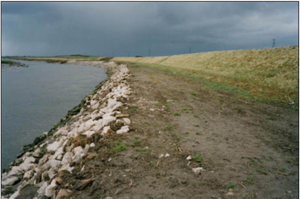
Plate B1.3 Toe and inward face protection using stone / rock rip rap
