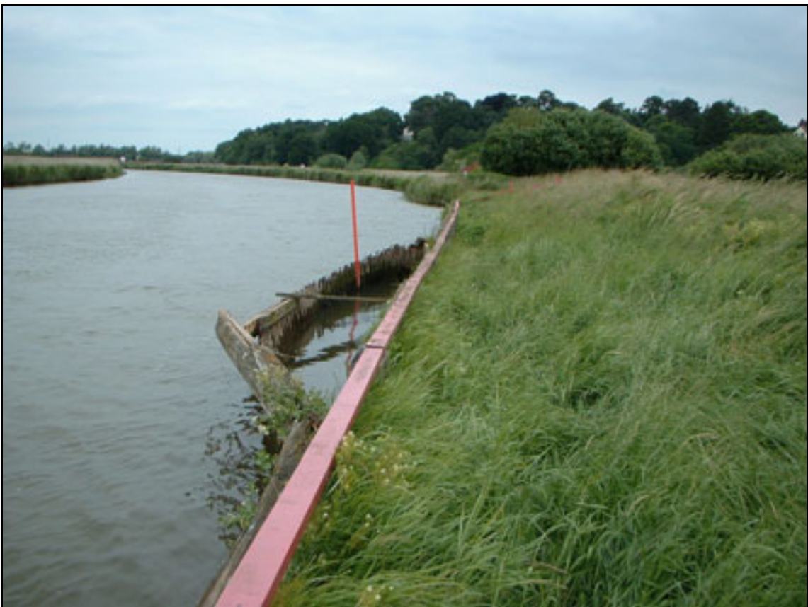
Plate B1.2 Failure of anchor in sheet piling protection
