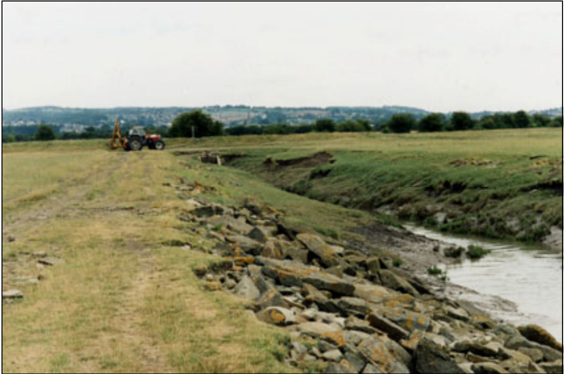
Plate A2.12 Bank instability in estuary area with high tidal range (stone placed as protection; cut off constructed to prevent progression)
