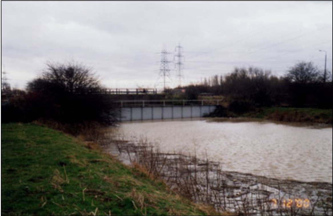
Plate A2.58 Interface between embankment and bridge abutment (low soffit railway bridge)
