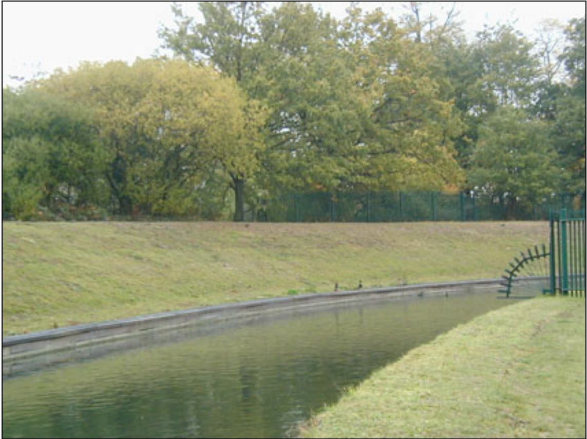
Plate B1.9 Toe and inward face protection using sheet piling (timber clad)
