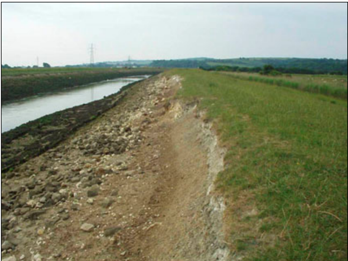
Plate B3.15 Erosion of inward face by river flow
