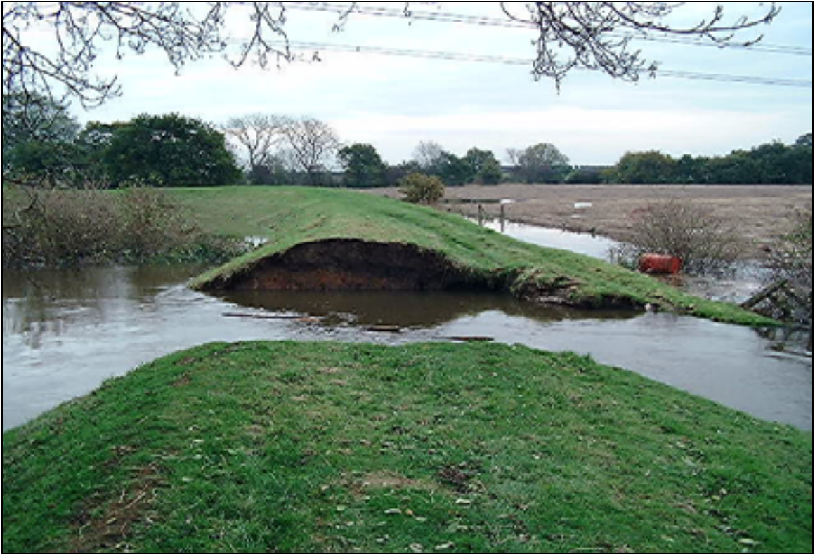
Plate A2.28 Failed culvert running through embankment
