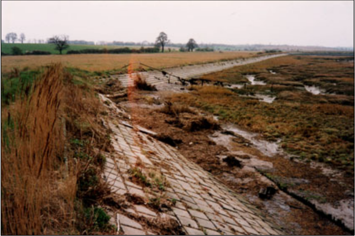
Plate B1.5 Toe and face protection using concrete blocks (stable in distance failing in foreground)
