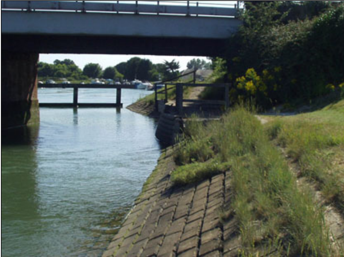
Plate A2.60 Typical 'mixed' construction at transition between embankment and bridge abutment
