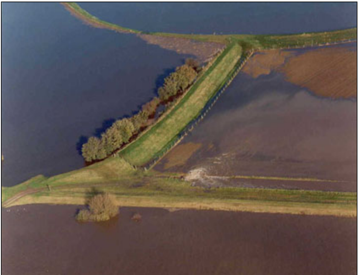
Plate B3.8 Piping through embankment
