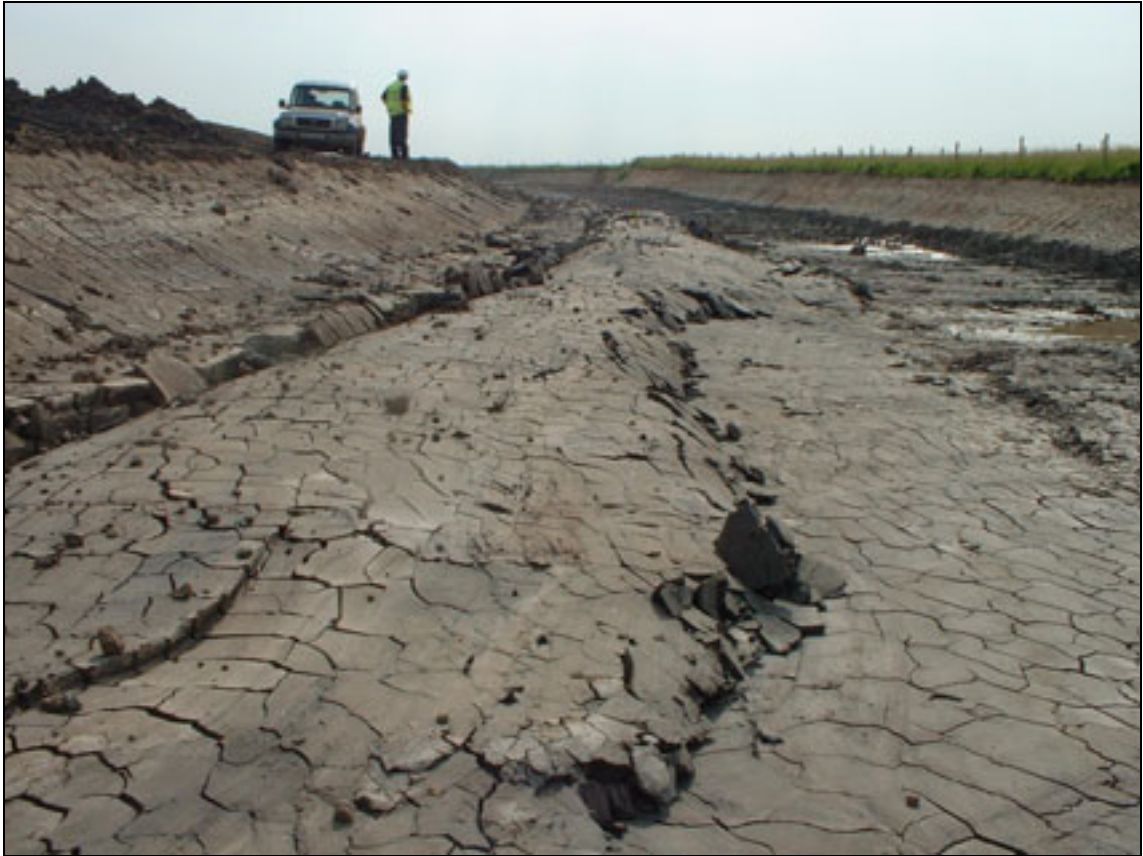
Plate A4.2 Embankment slip failure following drainage of soke ditch
