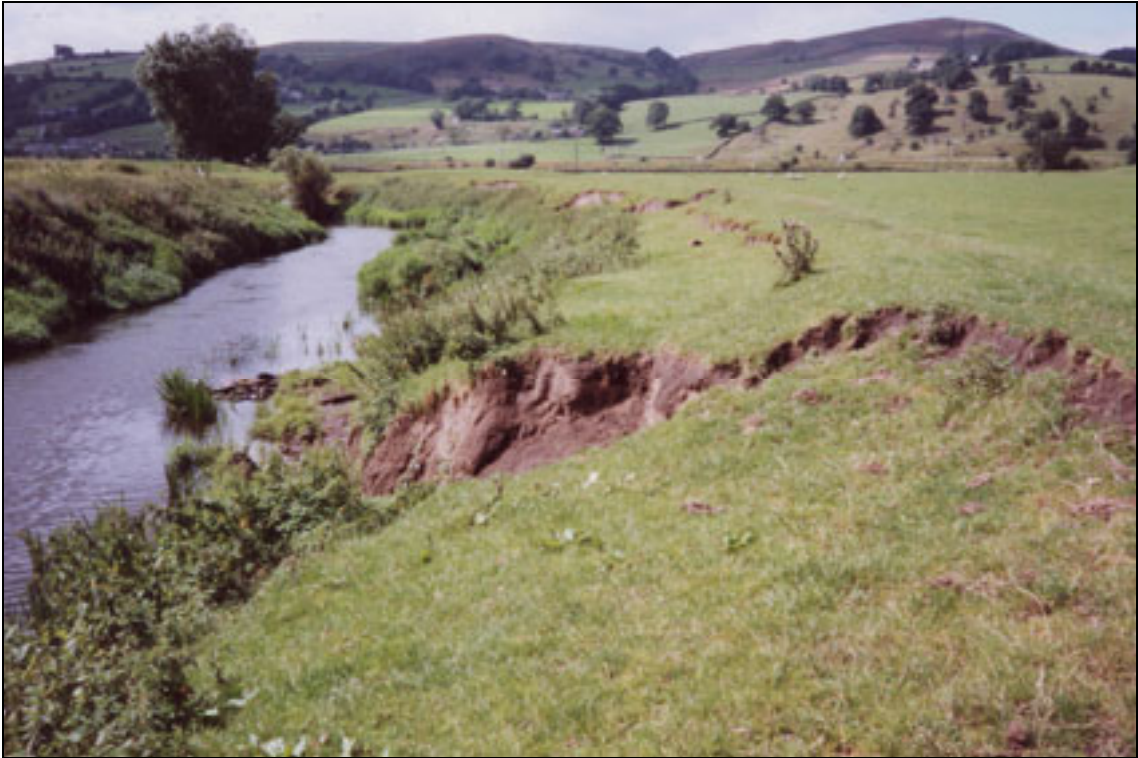
Plate B3.11 Inward face instability due to undercutting and surface failure
