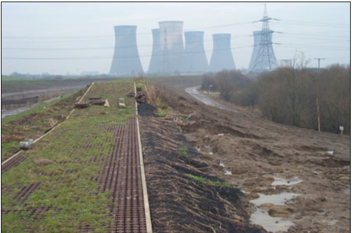
Plate A2.37 Partially completed works after overtopping incident
