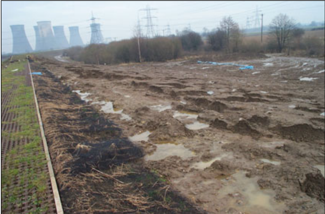
Plate A2.38 Damage to outward slope of embankment
