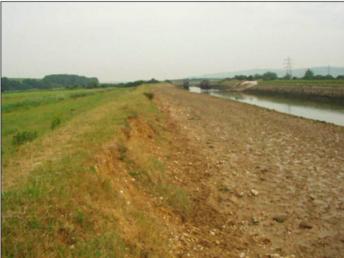
Plate B3.12 Inward face instability due to undercutting and surface failure
