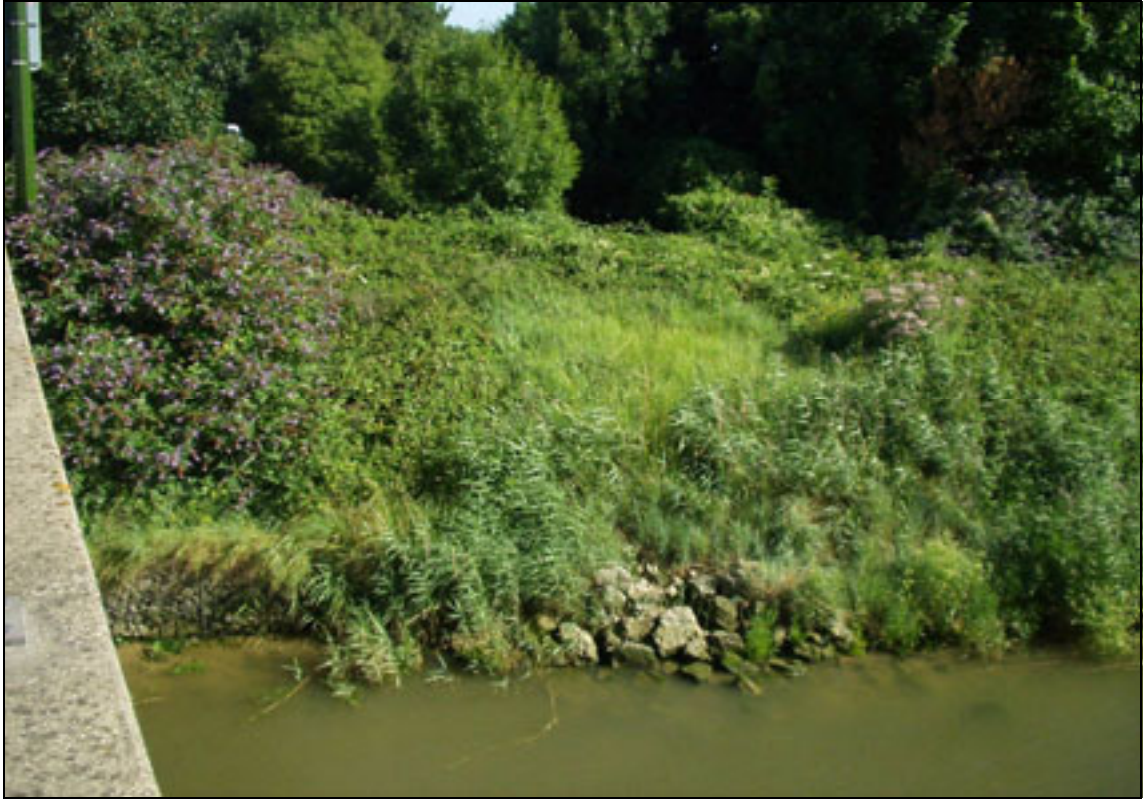
Plate A2.25 Poor vegetation management (plus indications of bank erosion at interface with bridge abutment)
