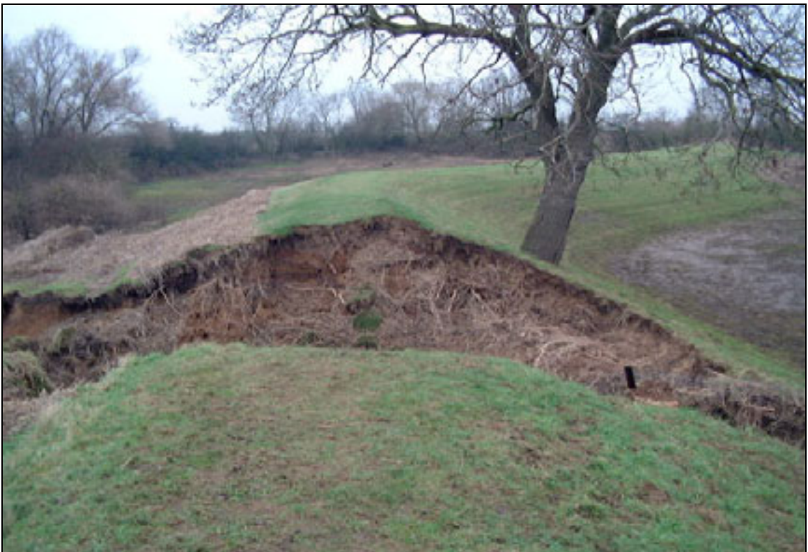
Plate A2.29 Failed culvert running through embankment
