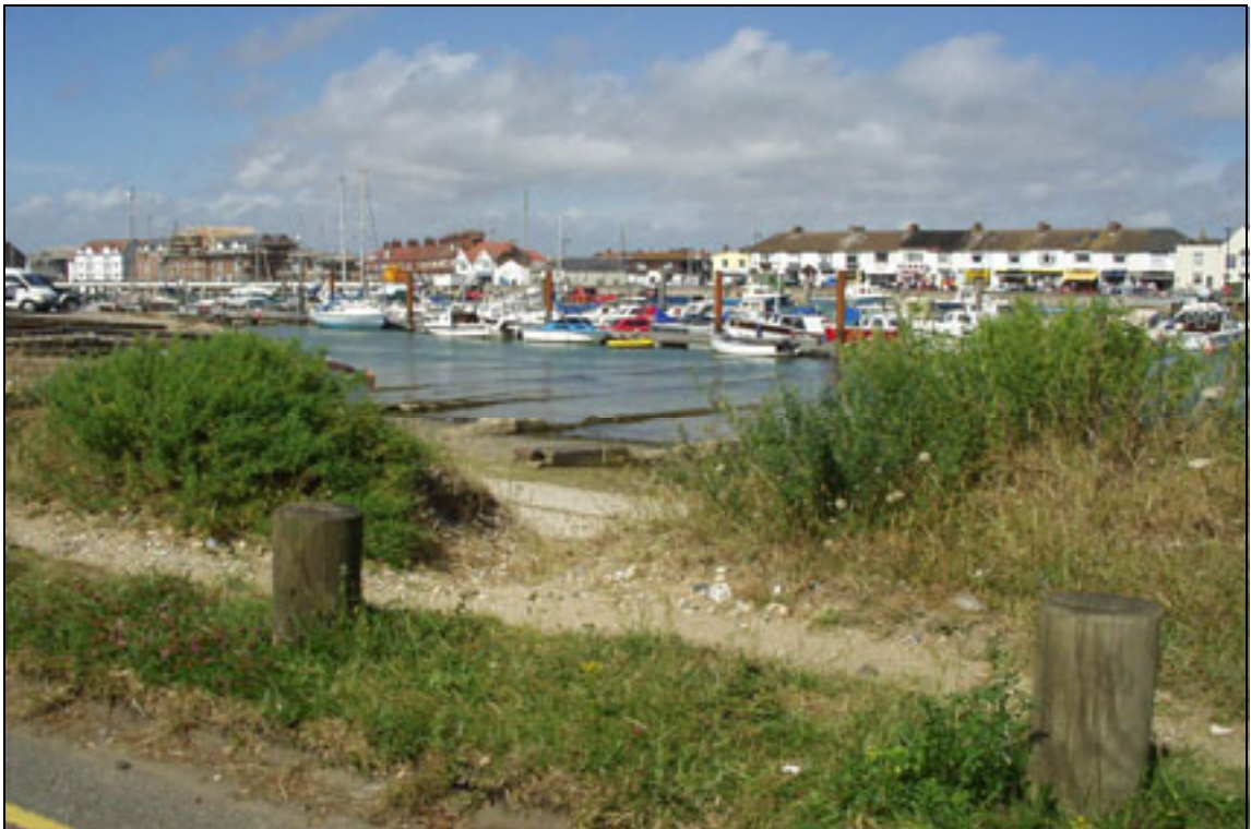
Plate A2.10 Estuary flood embankment (with crest eroded by pedestrian access)
