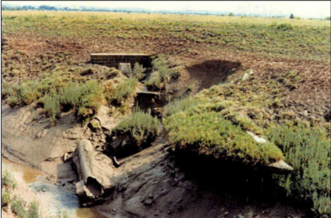
Plate A2.34 Outfall structure undercut by bank erosion
