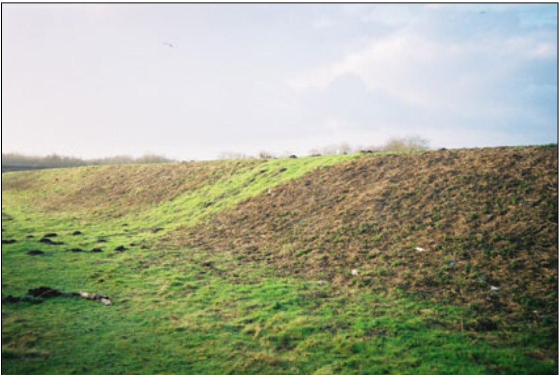
Plate B2.5 Poor vegetation quality on rear face of embankment
