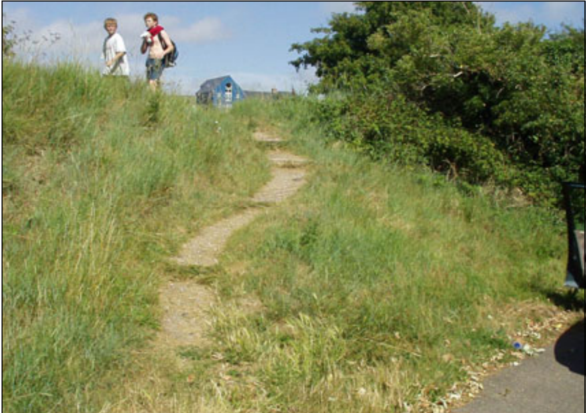
Plate A2.48 Stabilising erosion on inward face of embankment (installation of 5 small steps)
