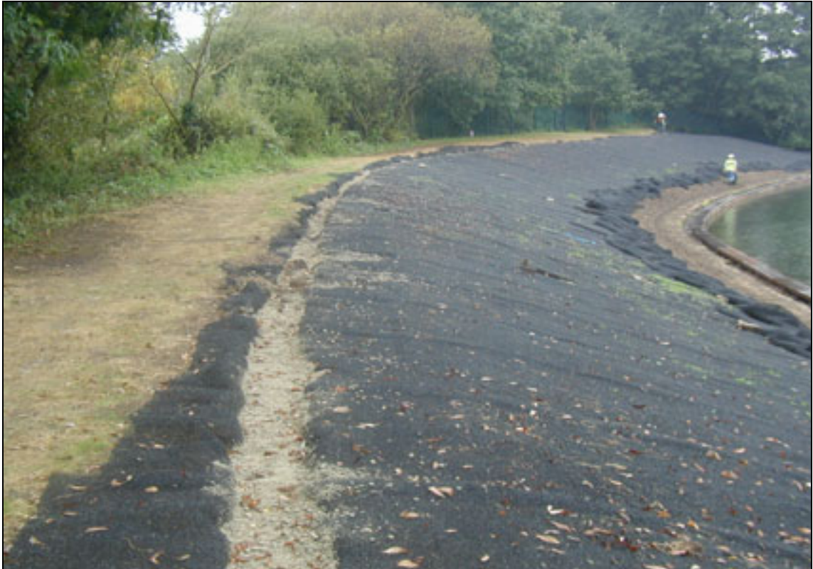
Plate B1.8a Toe and inward face protection using geotextile and vegetation (under construction)
