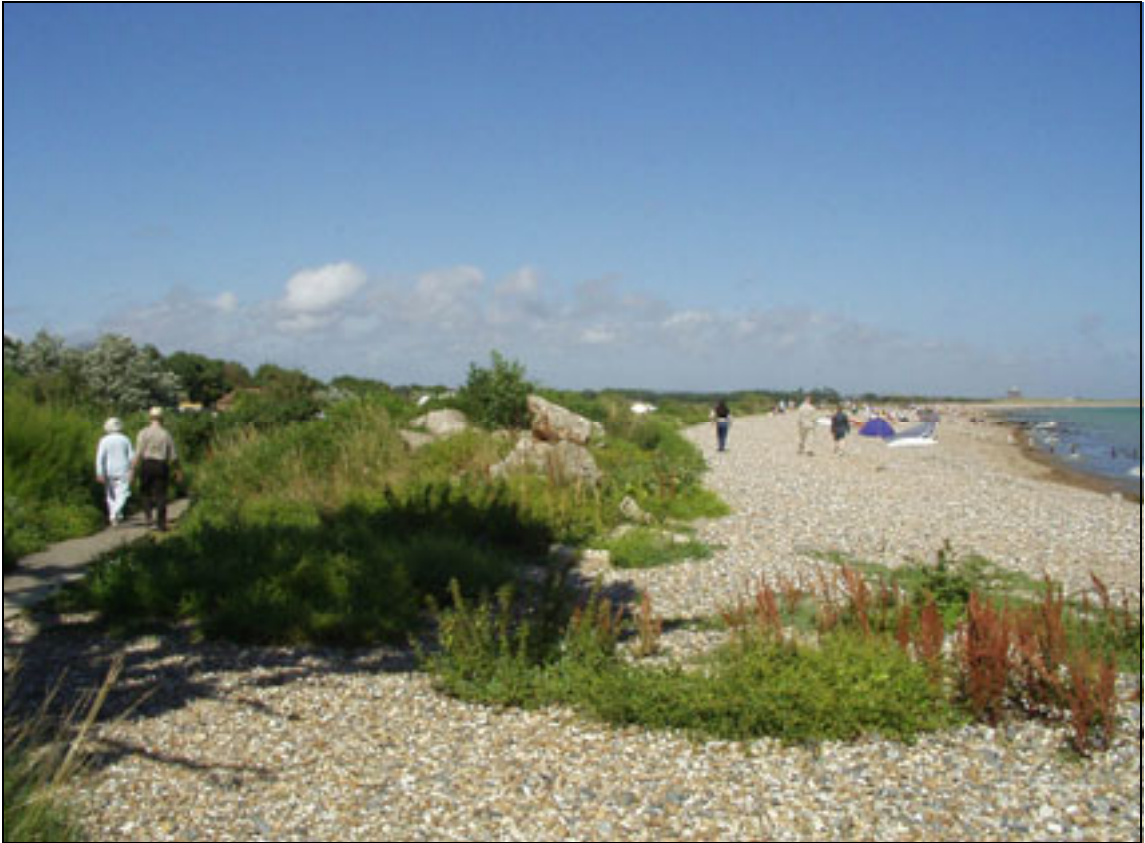
Plate A2.8 Coastal flood embankment (rock protection plus shingle bank on inward face)
