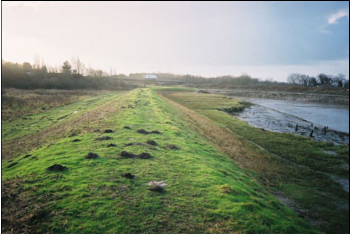
Plate A2.23 Signs of extensive mole activity in crest of embankment
