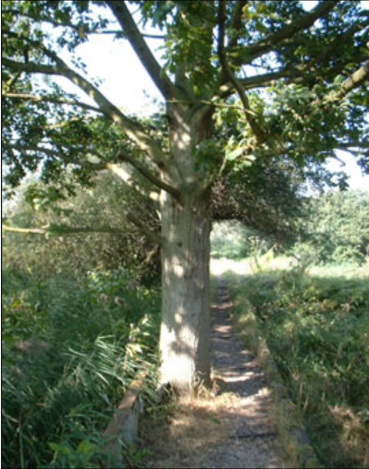
Plate B2.4 Tree growing through embankment
