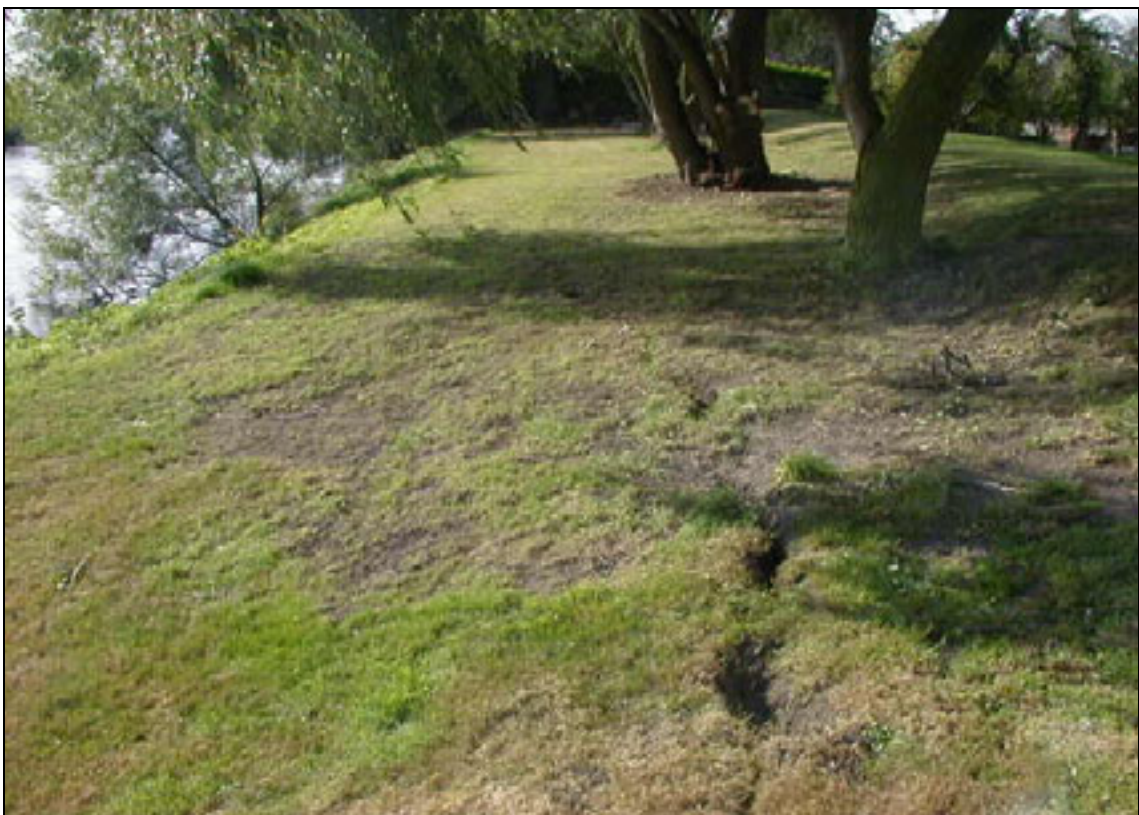
Plate B3.6 Cracking through embankment crest indicating rotational failure
