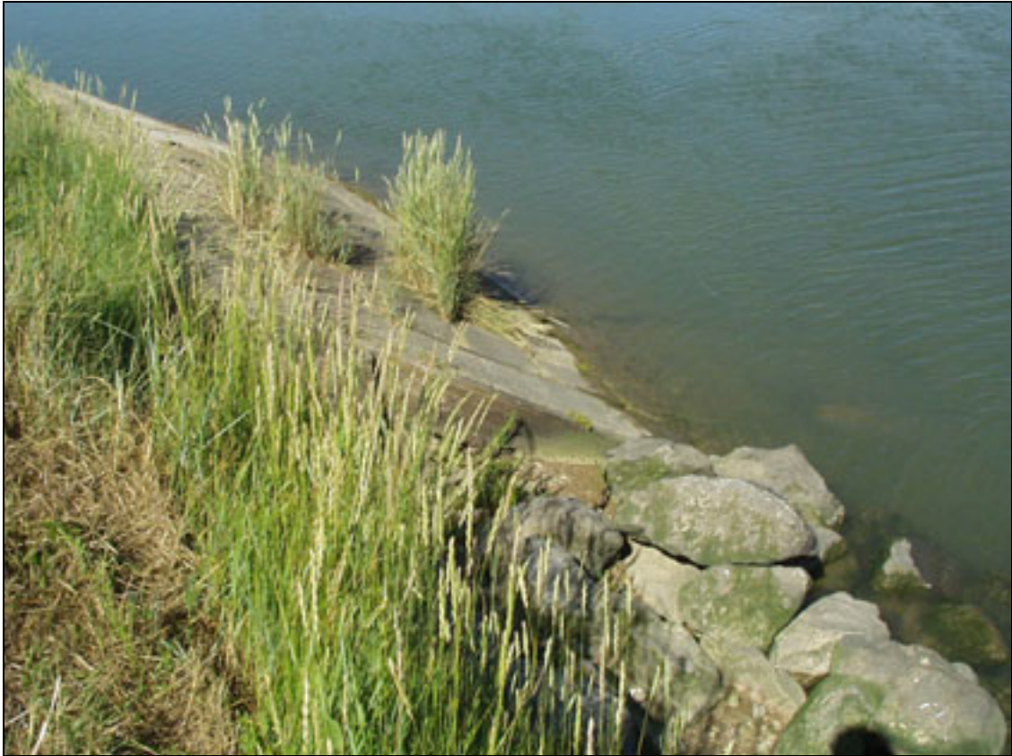
Plate B1.7 Poor detailing at end of slab protection (allowing embankment erosion behind protection)
