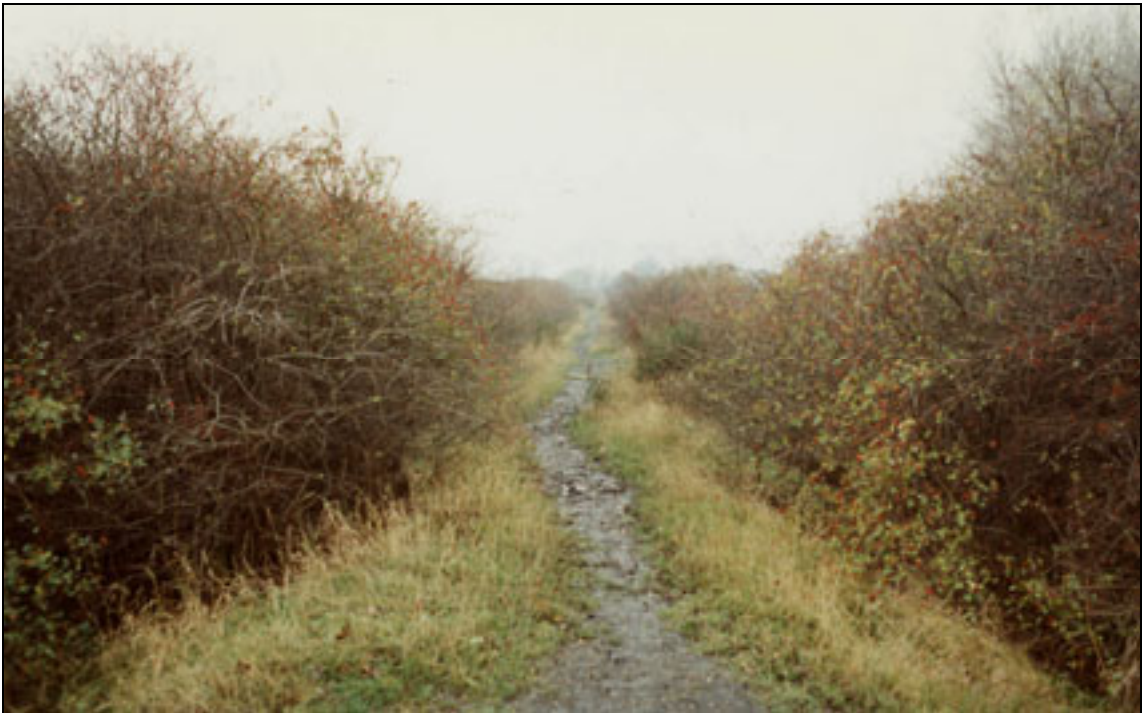
Plate B2.3 Excessive vegetation along embankment
