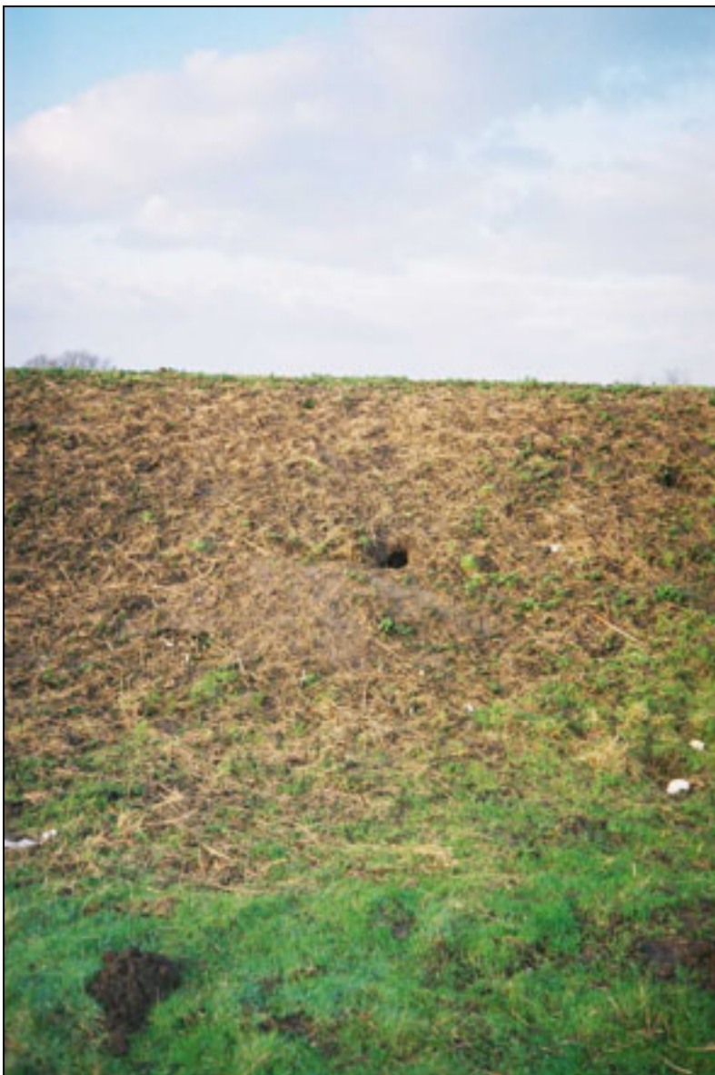
Plate A2.22 Rabbit hole through outward face of embankment
