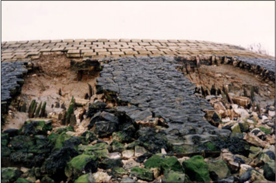
Plate B3.16 Erosion of inward face due to wave action
