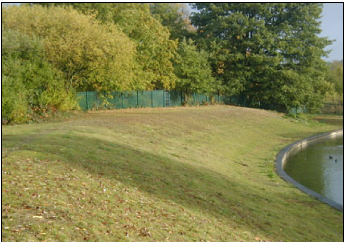
Plate B1.8b Toe and inward face protection using geotextile and vegetation (after vegetation is established)
