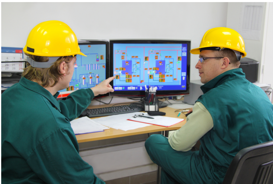
Figure 1: A control room
