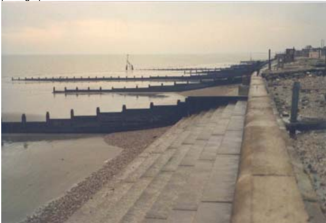
Low beach levels in front of stepped concrete wall, Selsey Bill (1988)
