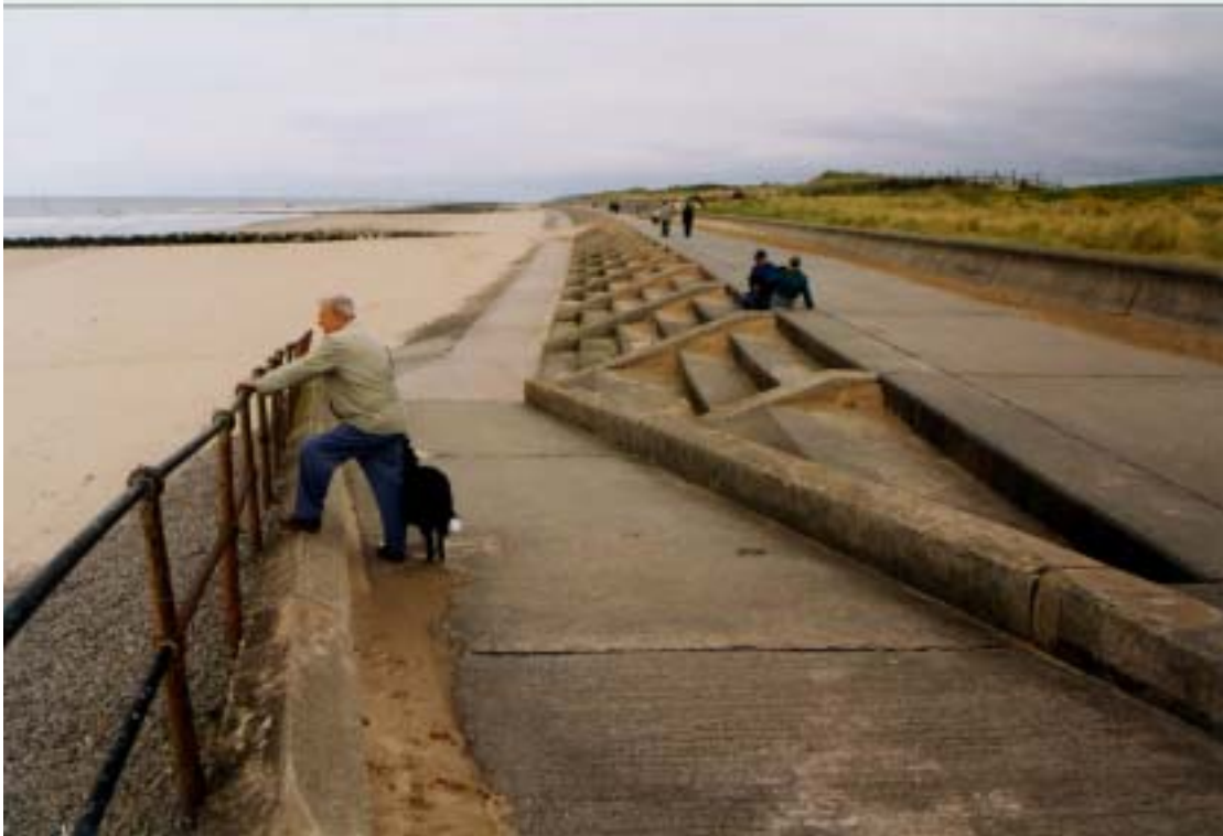
Sloping asphalt apron and rock groynes in front of steeped concrete seawall, Prestatyn
