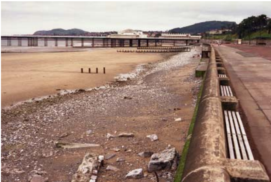
Beach lowering in front of vertical seawall, Colwyn Bay
