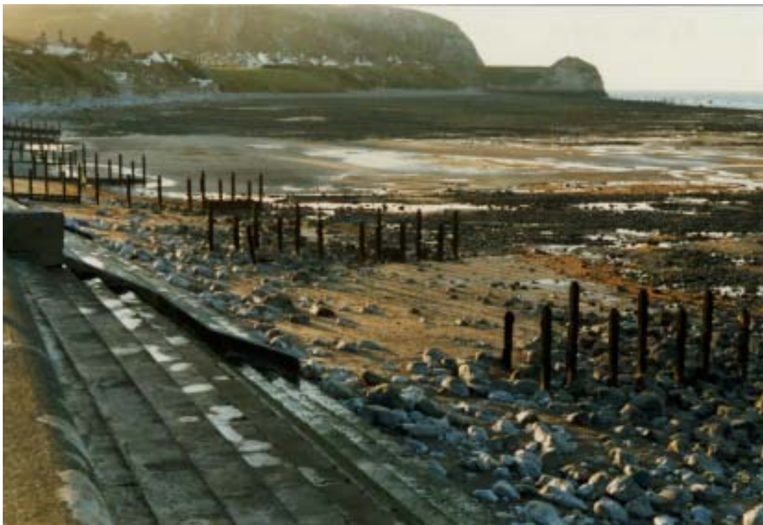
Lowered beach exposing shore platform, Penrhyn Bay
