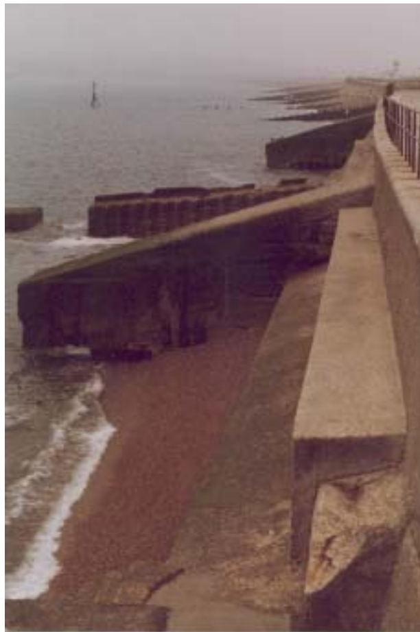
Low beach levels and damaged concrete seawall, Seaford (c1982)
