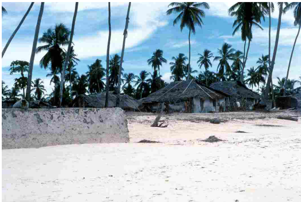
Plate 8 Erosion at downdrift end of seawall, Zanzibar
