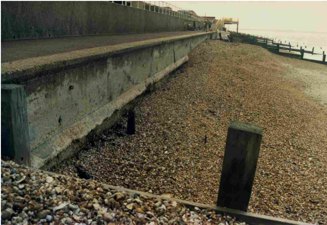
Plate 5 Beach lowering and undermining of seawall, Lee-on Solent
