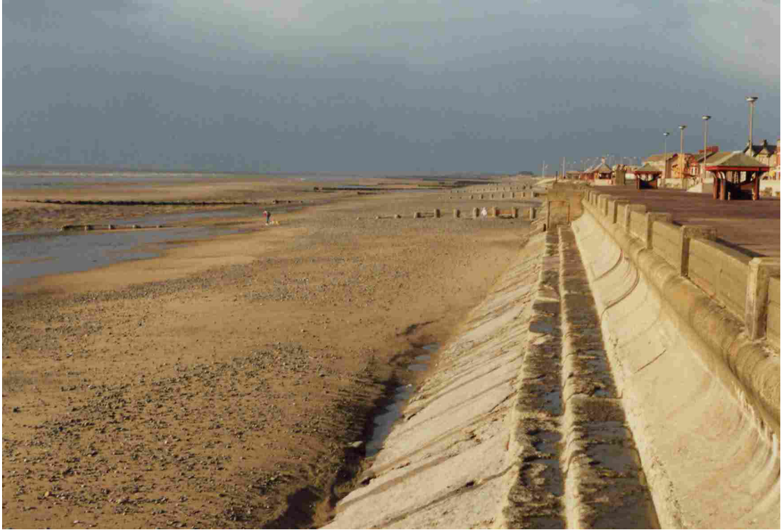
Plate 3 Localised scour runnel at toe of solid seawall, Wyre, Lancashire
