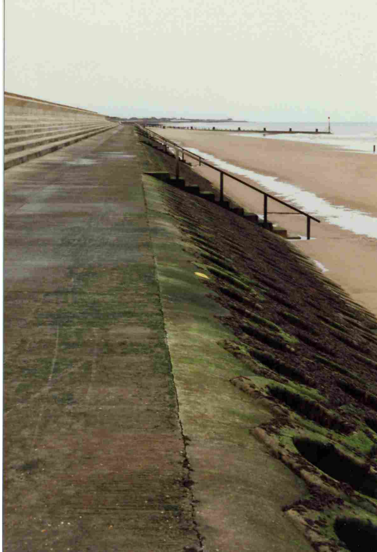
Plate 4 Localised scour runnel at toe of permeable seawall, Lincolnshire
