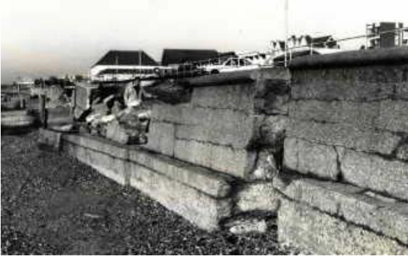
Figure 5.6 Sea wall failure at Lee-on-the-Solent (from Kemp, 1999)
