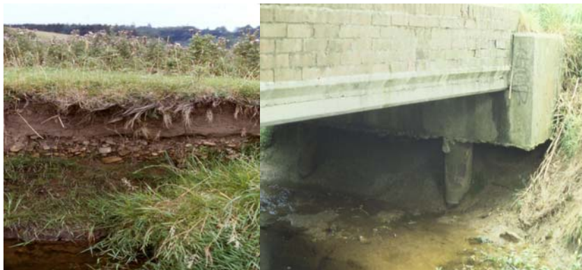
Figure 1.11 An example of channel incision revealed by exposure of a former river bed level in the bank material. Incision in this instance was a result of a land drainage scheme.
