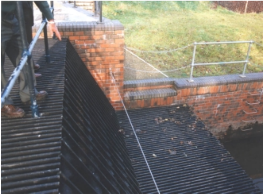
Figure 2.3 General view of the screen. The top handrail position makes raking difficult, also the steps down to the lower working platform have different rises. The screen rake is steeper than recommended in the Manual.
