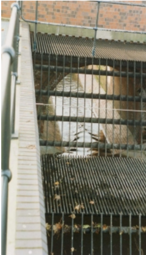
Figure 2.4 Trash clearance from the screen using rakes is made difficult by;
