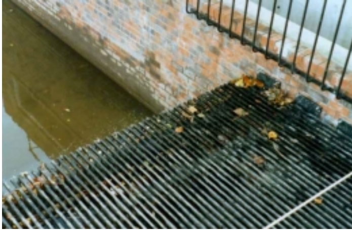
Figure 3.1 The vertical bars at top right protect the entry to the emergency overflow channel. These were fitted after initial commissioning.
