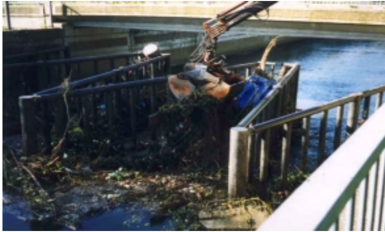
Figure 3.1.3 Large items of debris are removed by mechanical grab once the event has subsided.
