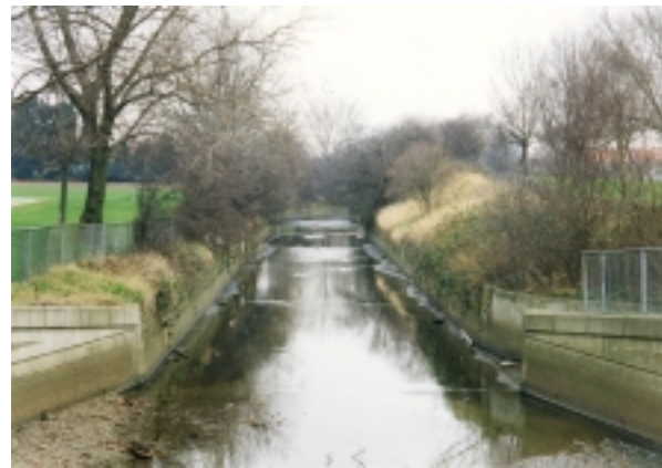
Figure 2.4.2 View upstream, under normal flow conditions. There can be a significant build up of transported river bed material collected in the silt trap.
