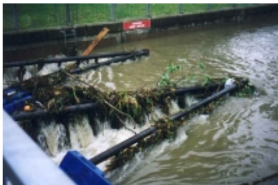
Figure 3.1.1 Debris collecting on the screen prior to the event reaching its peak. The weir effect of the structure is clearly visible.
