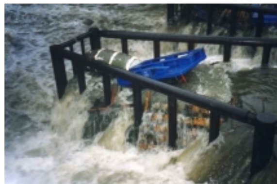
Figure 3.1.2 Debris collected on the screen during a significant event. The type of debris oil drums and pallets have the potential to damage the
