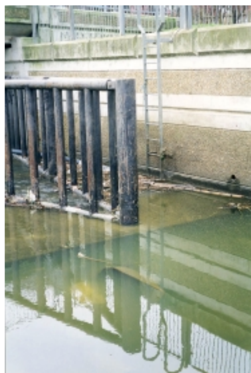
Figure 3.3 Entry to the channel can be from the ladder as shown in the photograph or by vehicle ramp. However the silt trap poses an additional safety risk as it is between the ramp and the structure. The step down is clearly visible in the photograph.
