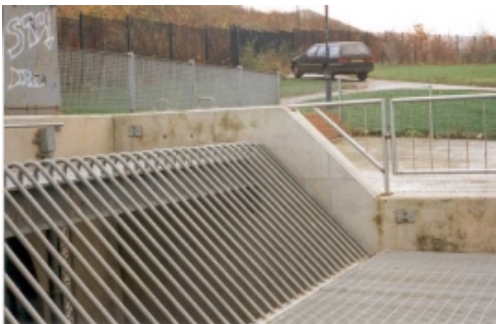
Figure 2.5 The screen site includes a concrete hard standing and areas for turning vehicles. The access road is dedicated to the screen.
