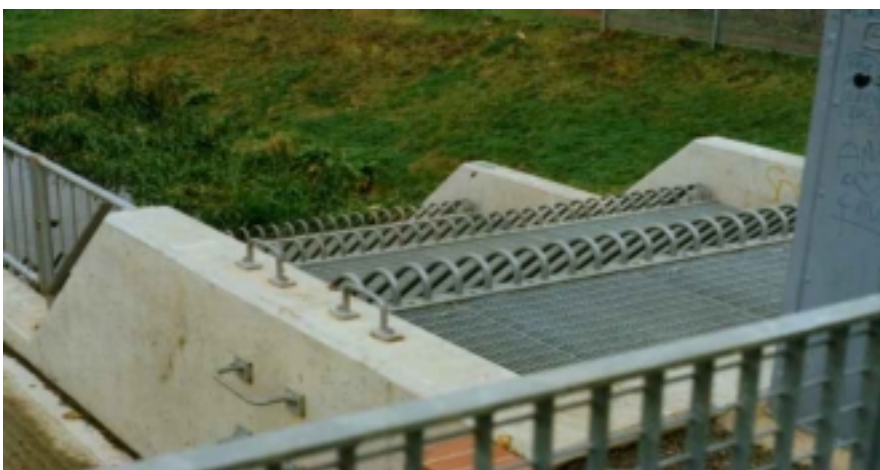
Figure 2.3 General view of the screen clearly showing the three stages and the heavy duty construction materials.
