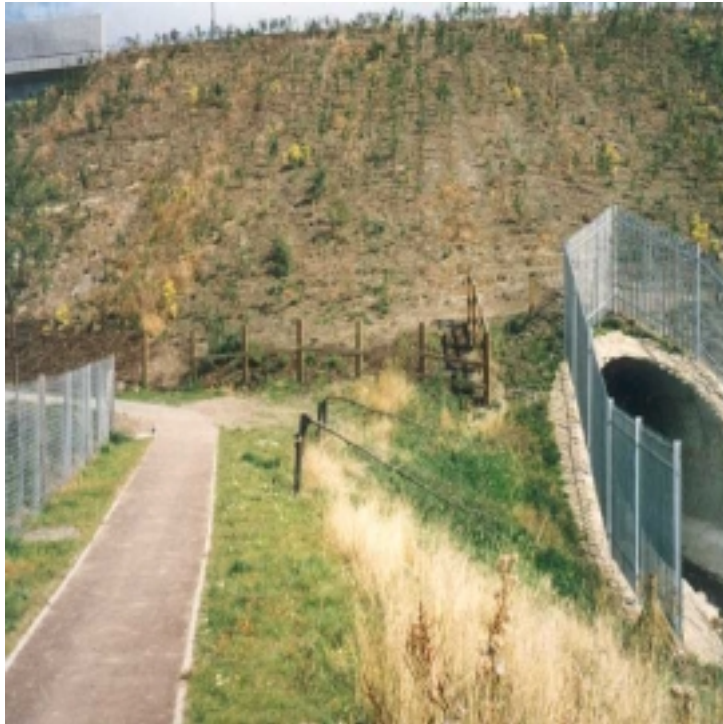
Figure 1.4 View showing the public footpath running adjacent to the new culvert and the inadequacy of the fencing.
