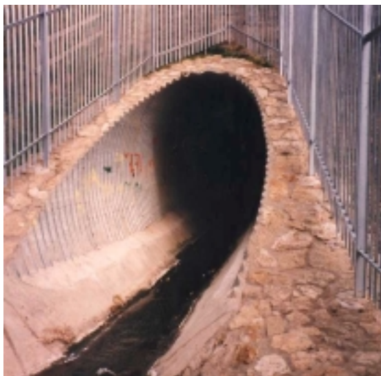
Figure 1.2 View on the new armco culvert, note the concrete haunching allowing access into the culvert. The fence was installed after the fatal accident. However, it did not deter children from entering the culvert.
