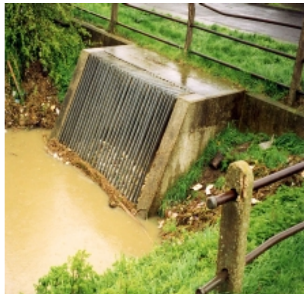
Figure 3.1.2 View of the screen at 1 in 20 year event. The water level is below peak at this point. Notice that there is debris behind the screen.
