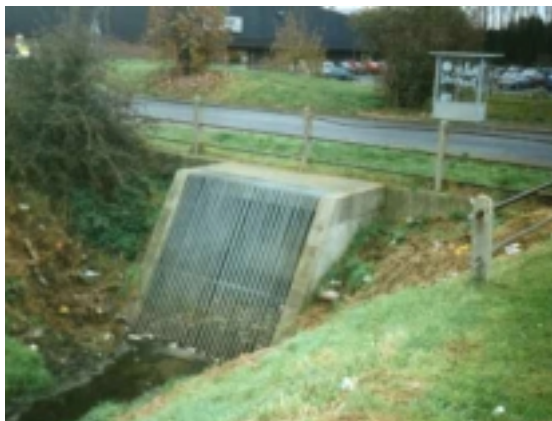
Figure 3.1.1 View of the screen under normal flow conditions.
