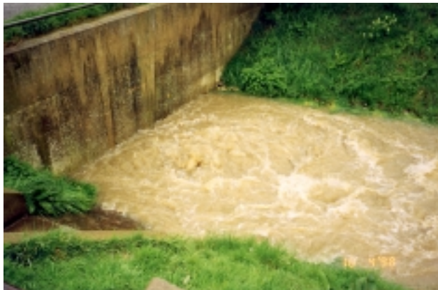
View of the syphon outlet downstream of the screen during high flows. The syphon creates significant turbulence downstream
