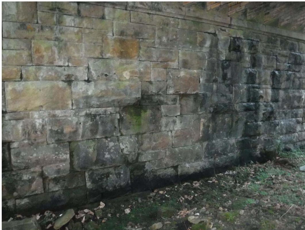
Photo No.2: Possible further deterioration: To the eroded stonework areas.
