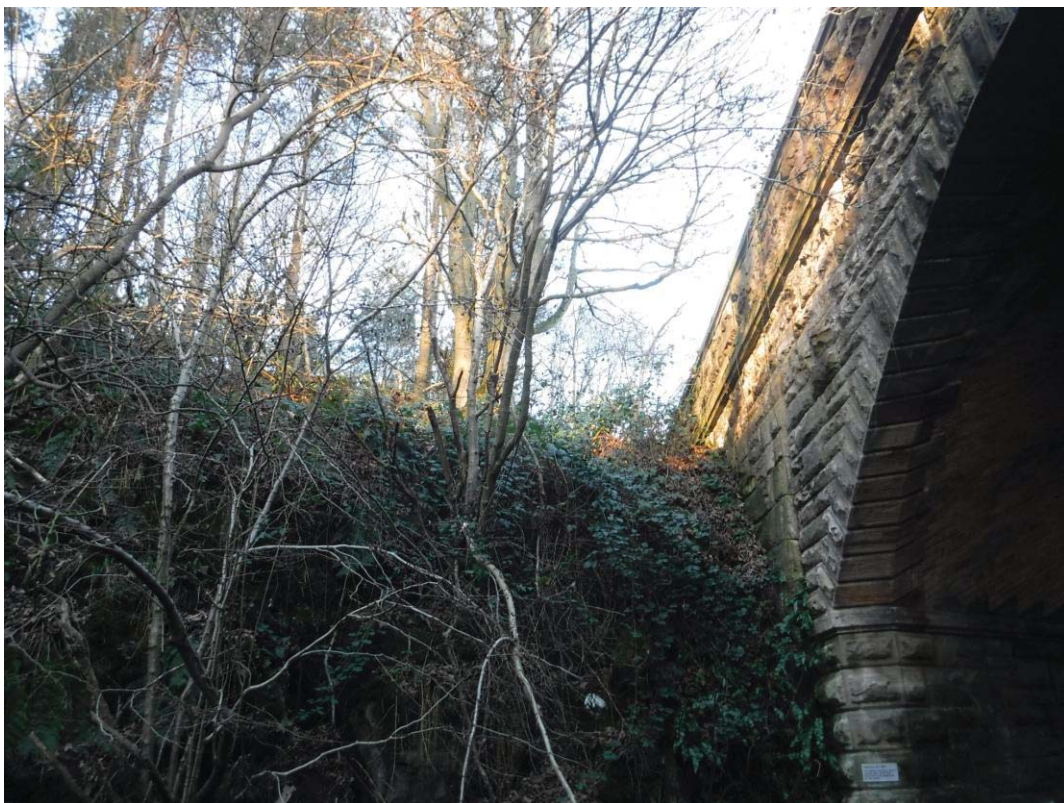
Photo No.1: Mature tree growth: Within of the proximity of the structure.
