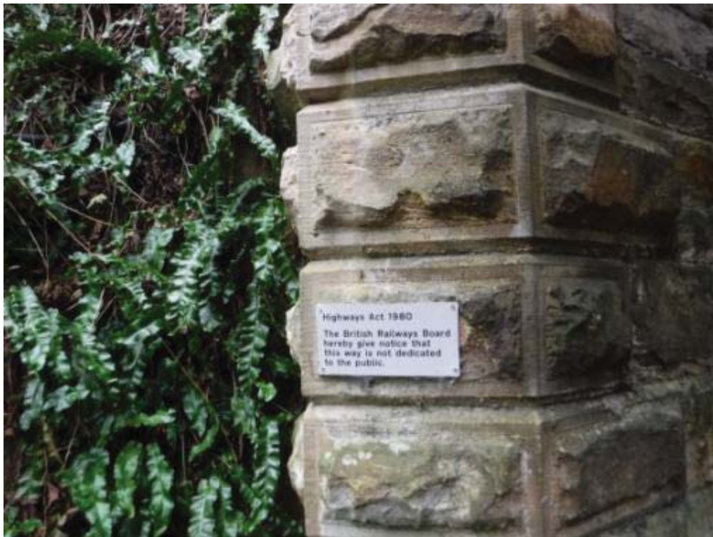
Photo No: 6 - Non - Dedication plate: Typical example of the condition. {BRB}
