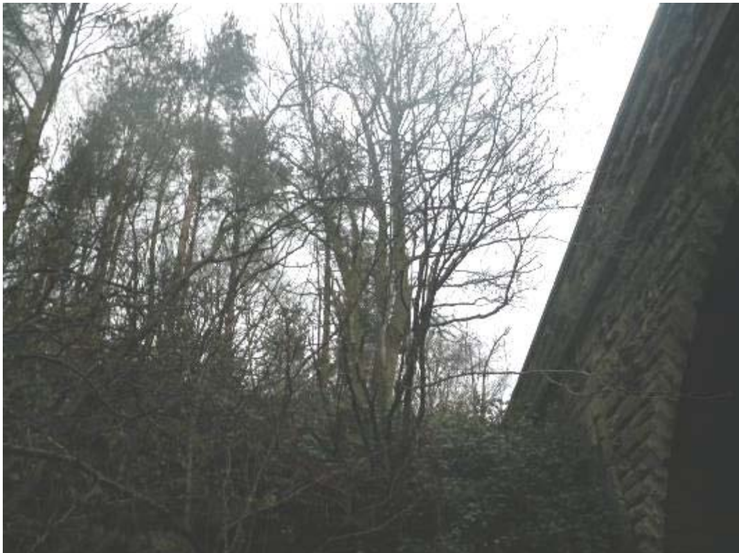
Photo No.1: Mature tree growth: Within the proximity of the structure.
