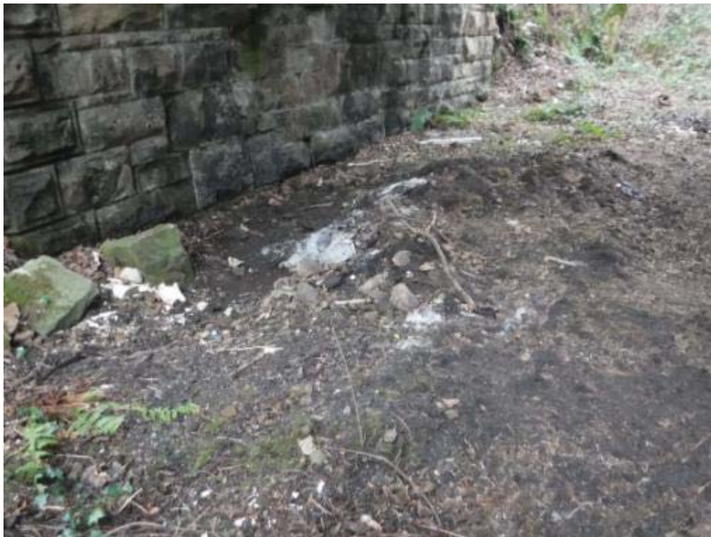
Photo No: 2 – Area under the structure: Evidence of extinguished fire.
