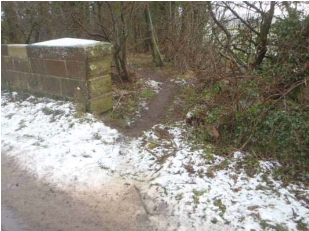
Photo No.3: Approach road fencing/walling: Typical example of the condition at S/E end.
