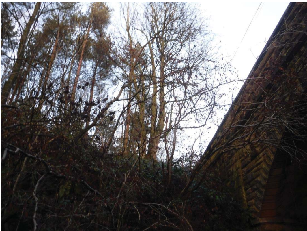
Photo No.1: Mature tree growth: Within of the proximity of the structure.
