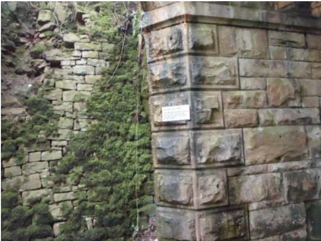
Photo No.9: Non - Dedication plate: Provided to the abutment.
