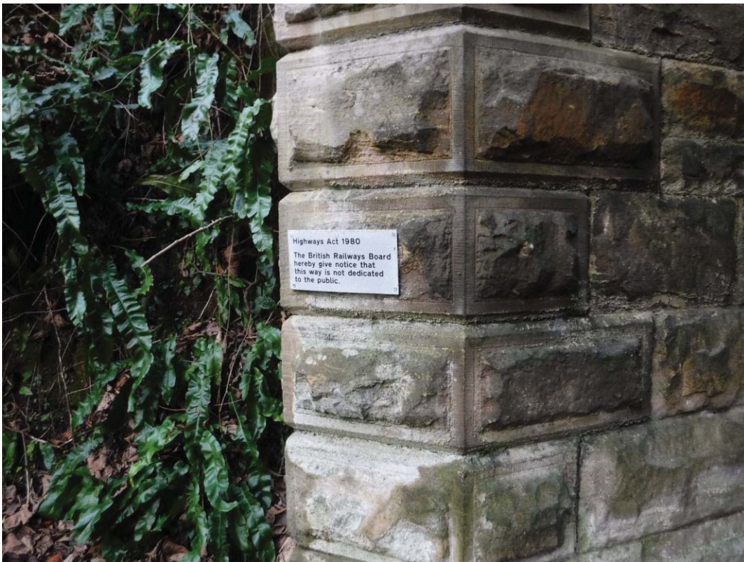
Photo No.5: Non - Dedication plate: Typical example of the condition. {BRB}
