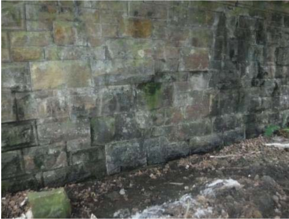
Photo No: 3 – Erosion to the stonework: Typical example.
