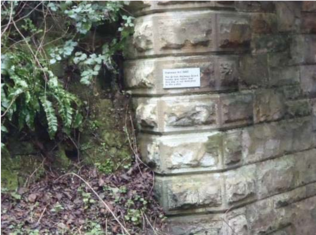
Photo No.8: Non - Dedication plate: Provided to the abutment.
