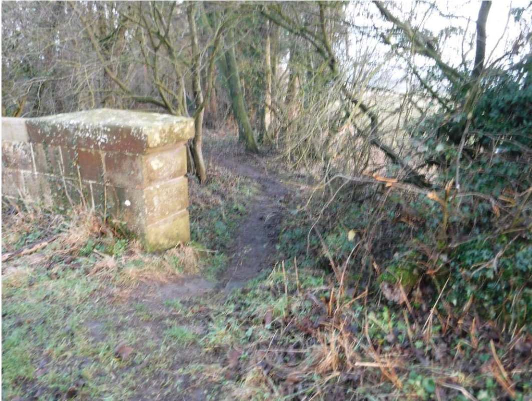
Photo No.4: Approach road walling: Typical example of the condition at S/E end.
