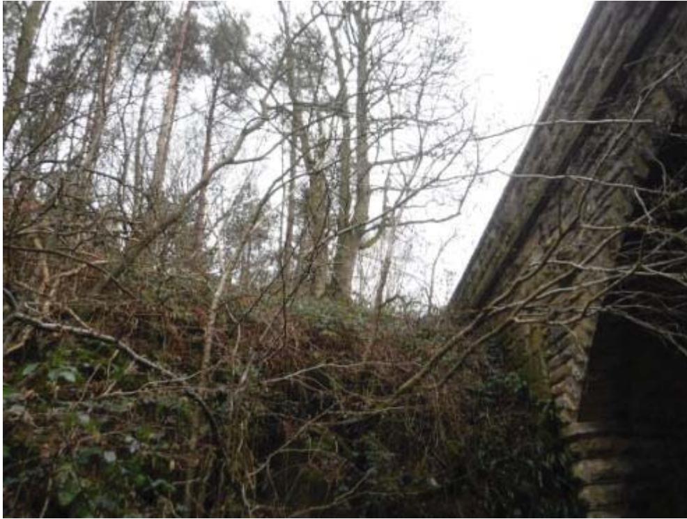
Photo No: 1 – Mature tree growth: Within of the proximity of the structure.
