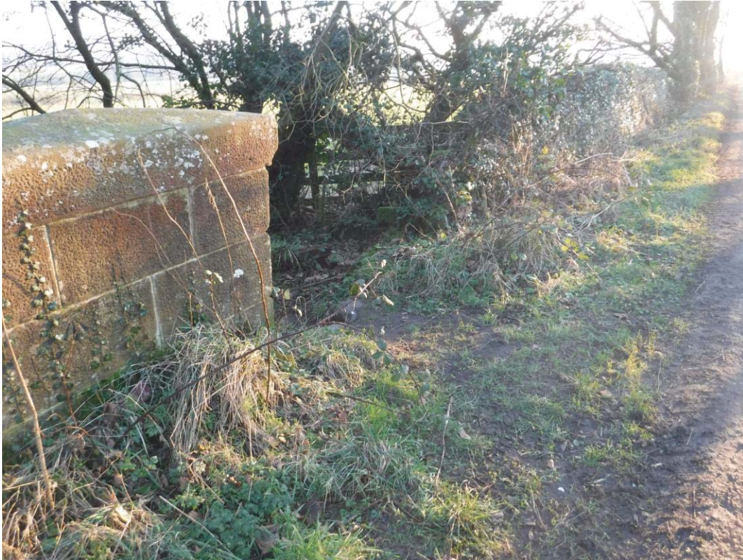
Photo No.4: Approach road walling: Typical example of the condition at S/E end.
