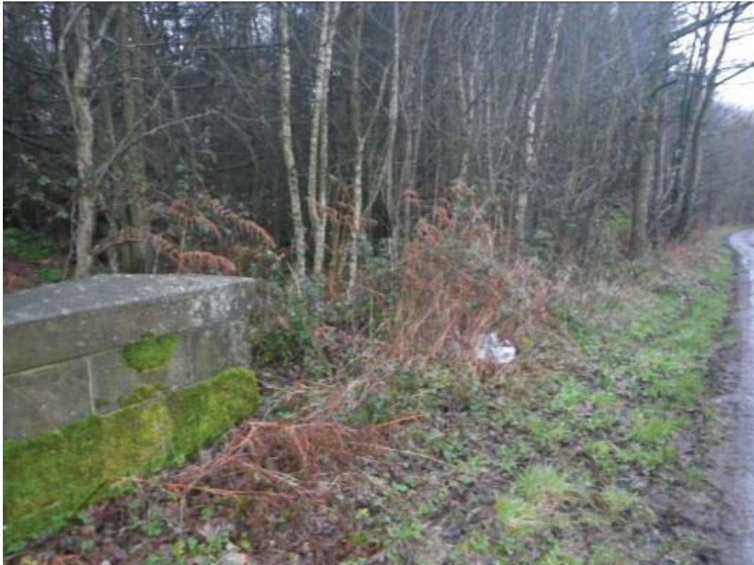
Photo No.4: Approach road fencing/walling: Typical example of the condition at N/W end.
