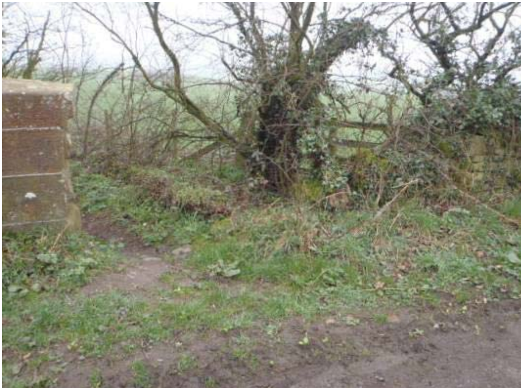
Photo No.10: Approach road fencing/walling: Typical example of the condition at S/E end.
