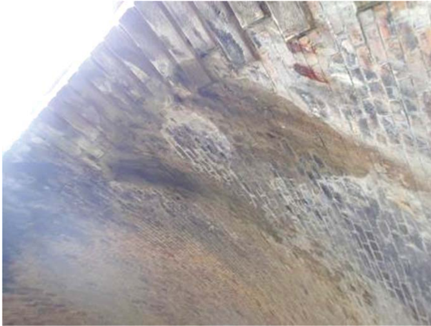
Photograph 10: example of water ingress through the soffit
