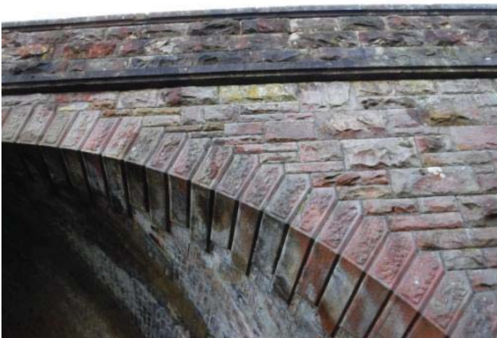
Photo No.28 - North arch ring face: Typical example of the condition.
