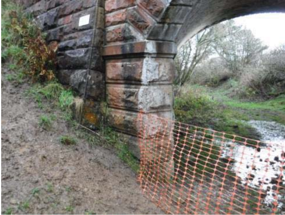
Photo No.63 - East abutment: Typical example of the condition at the N/E return section.
