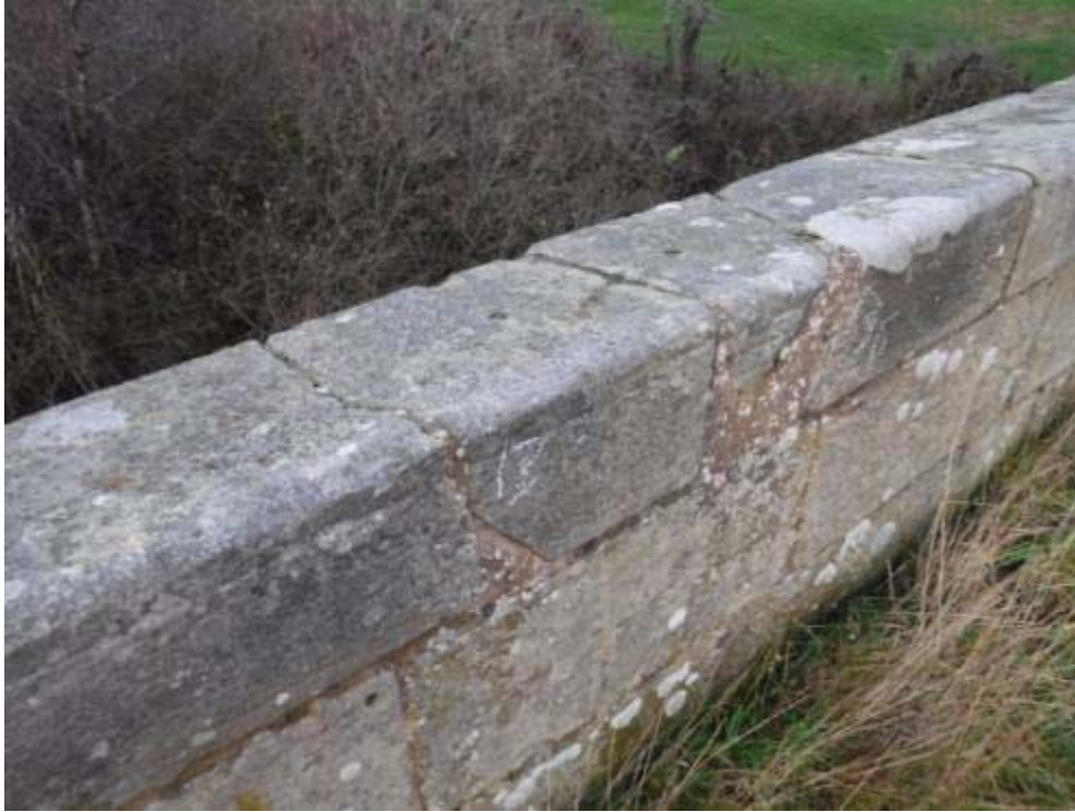
Photo No.105 - North roadside parapet: Fractured coping stones at 13.00m. & 13.60m.
