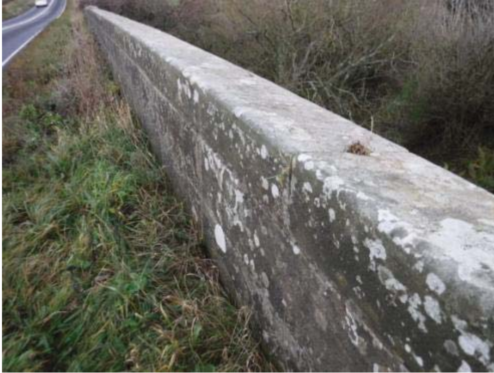
Photo No.129 - South roadside parapet: Displacement to the coping stones.
