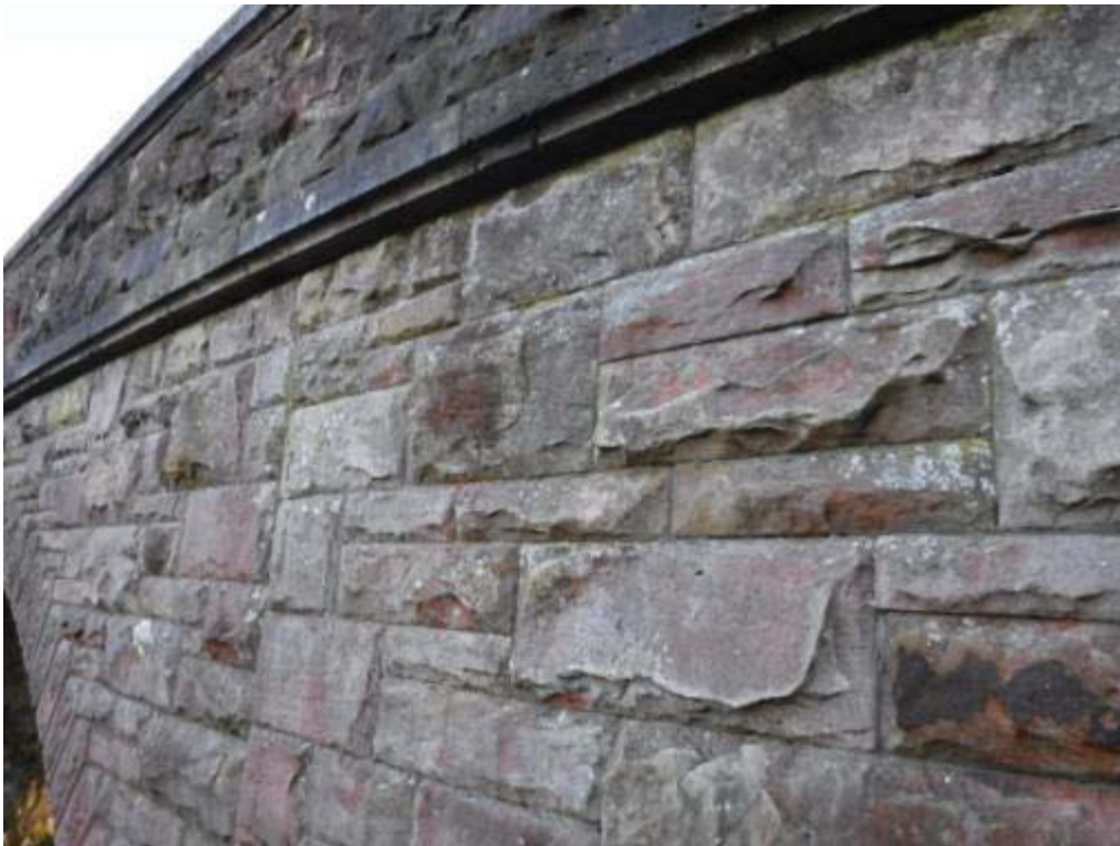
Photo No.84 - N/W wing wall: Typical example of the condition.
