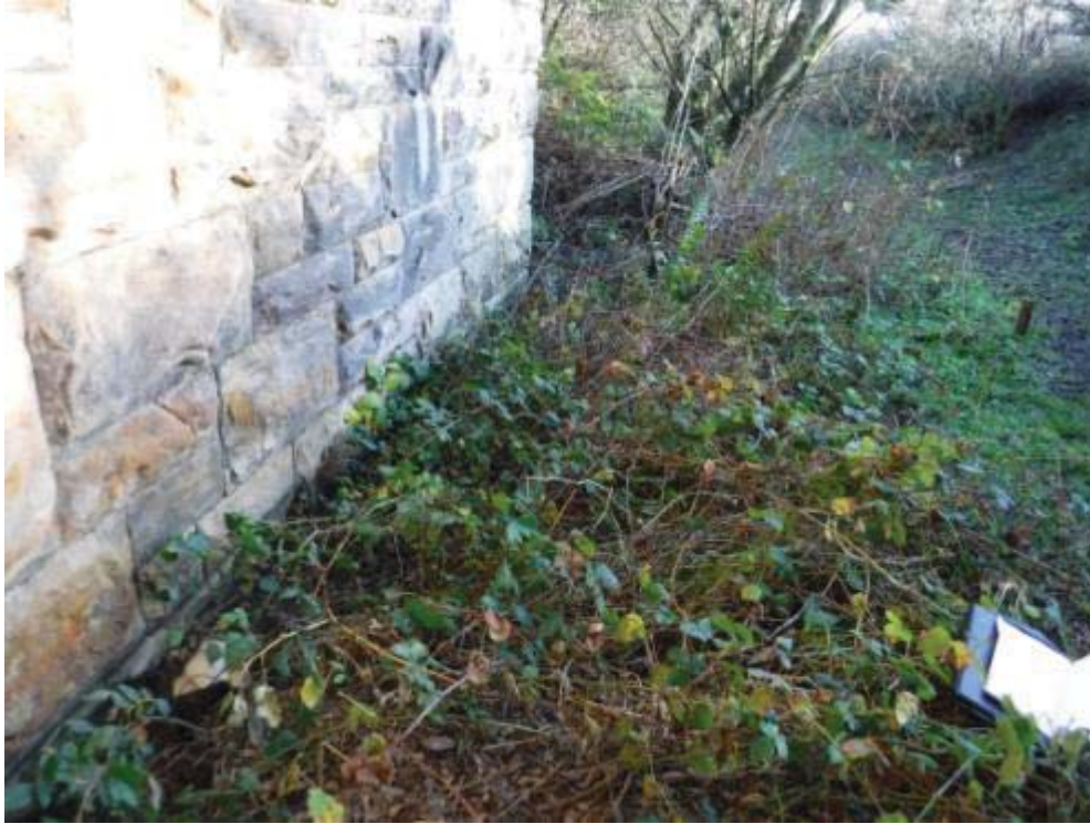
Photo No.65 - East abutment: Standing water at the S/E end.
