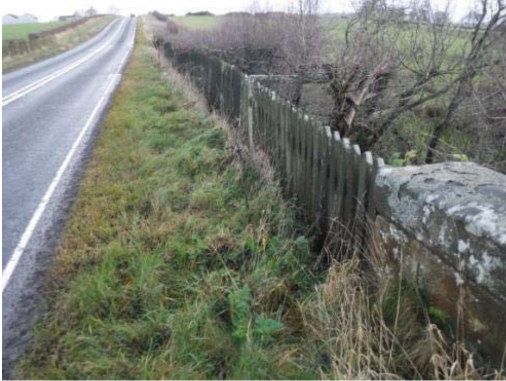
Photo No.161 - Approach road fencing: Typical example of the condition at S/E end.
