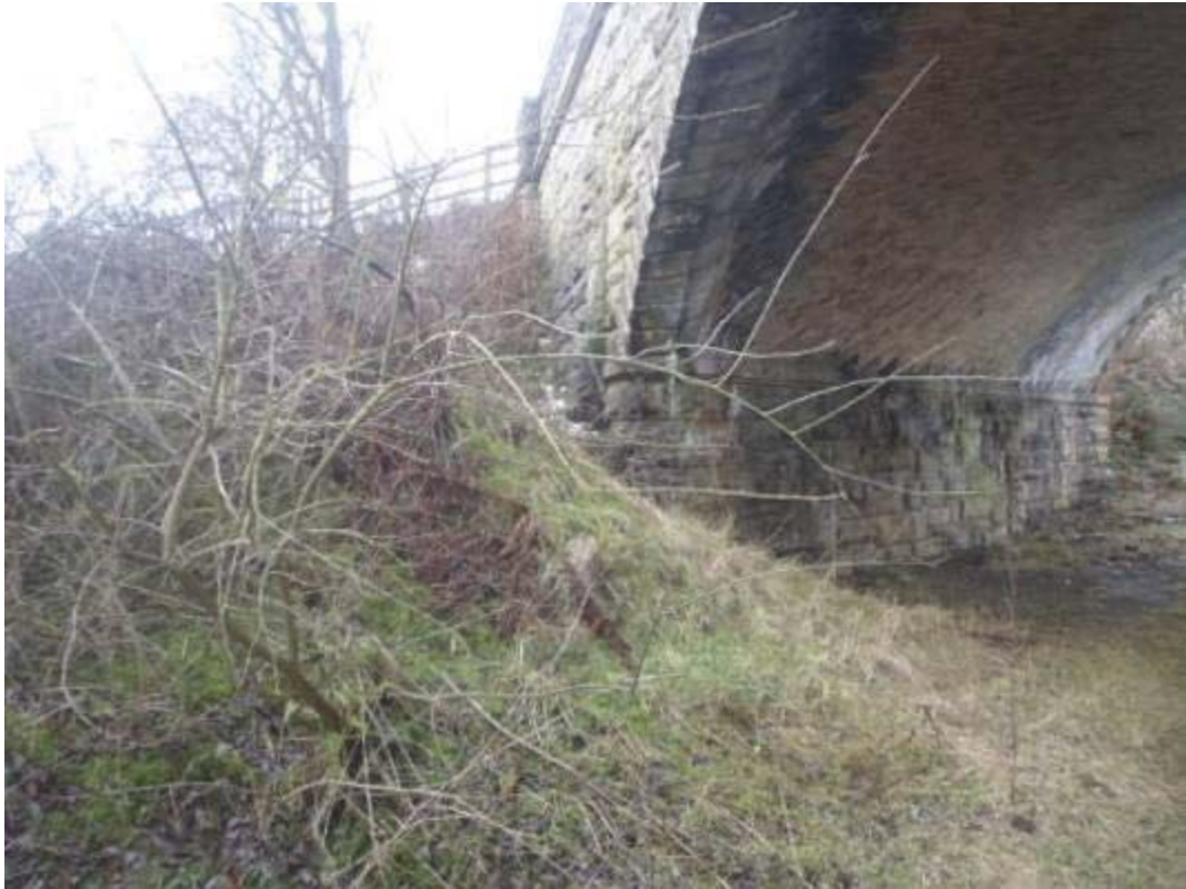
Photo No.4: Vegetation: Typical example.
