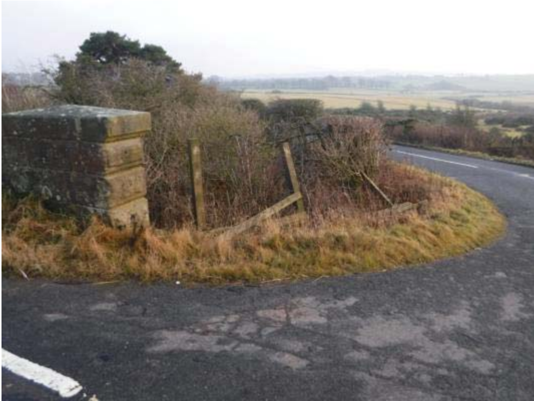
Photo No.2: Approach road fencing: Typical example of the condition at S/W end.
