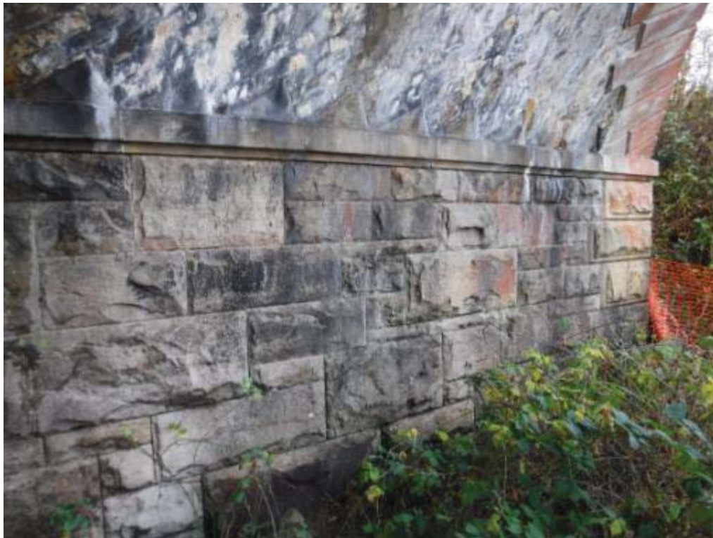
Photo No.70 - West abutment: Typical example of the condition.
