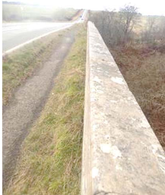
Photograph 14: long-standing leaning action is noted along the north parapet
