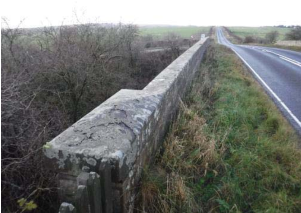
Photo No.136 - South roadside parapet: Typical example of the alignment & condition of the coping stones.
