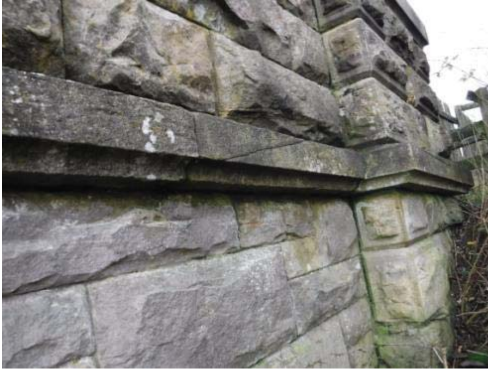
Photo No.155 - String course: Fissure type fractured stonework.
