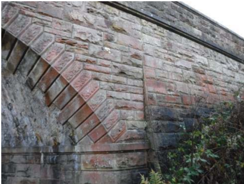
Photo No.44 - North spandrel: Typical example of the condition.
