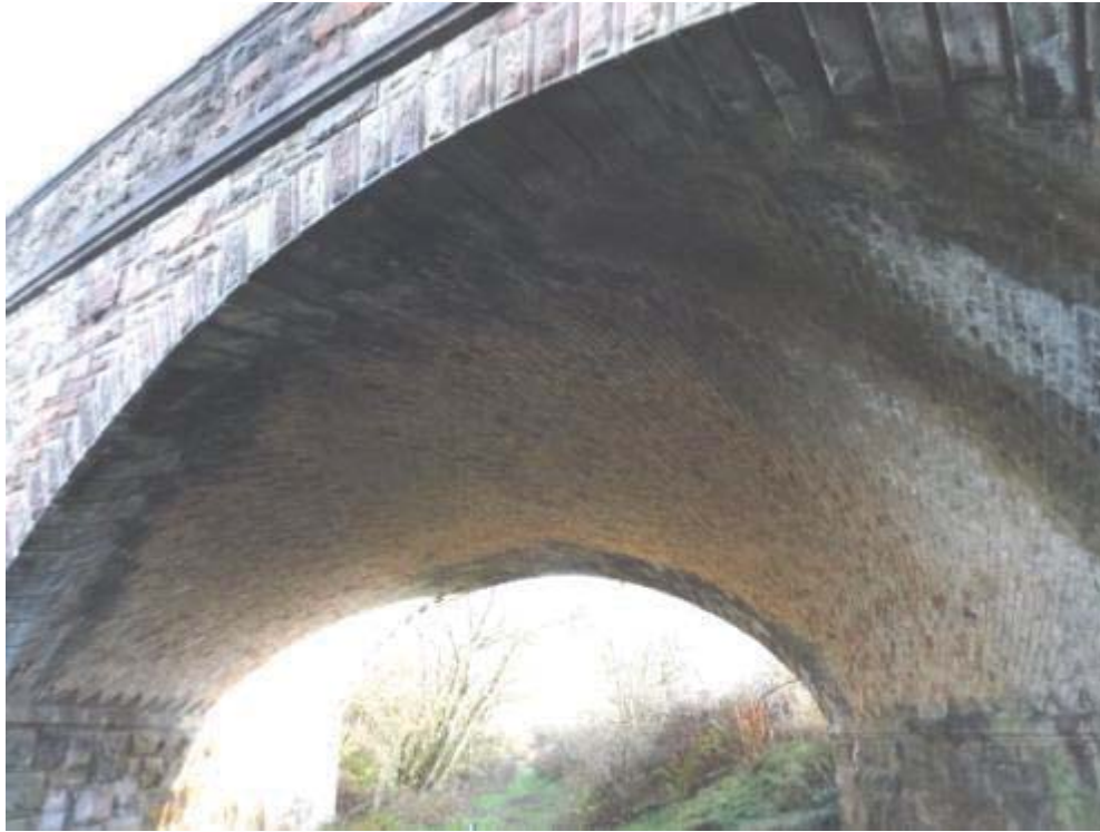
Photo No.15 - Arch ring soffit: Typical example of the condition.
