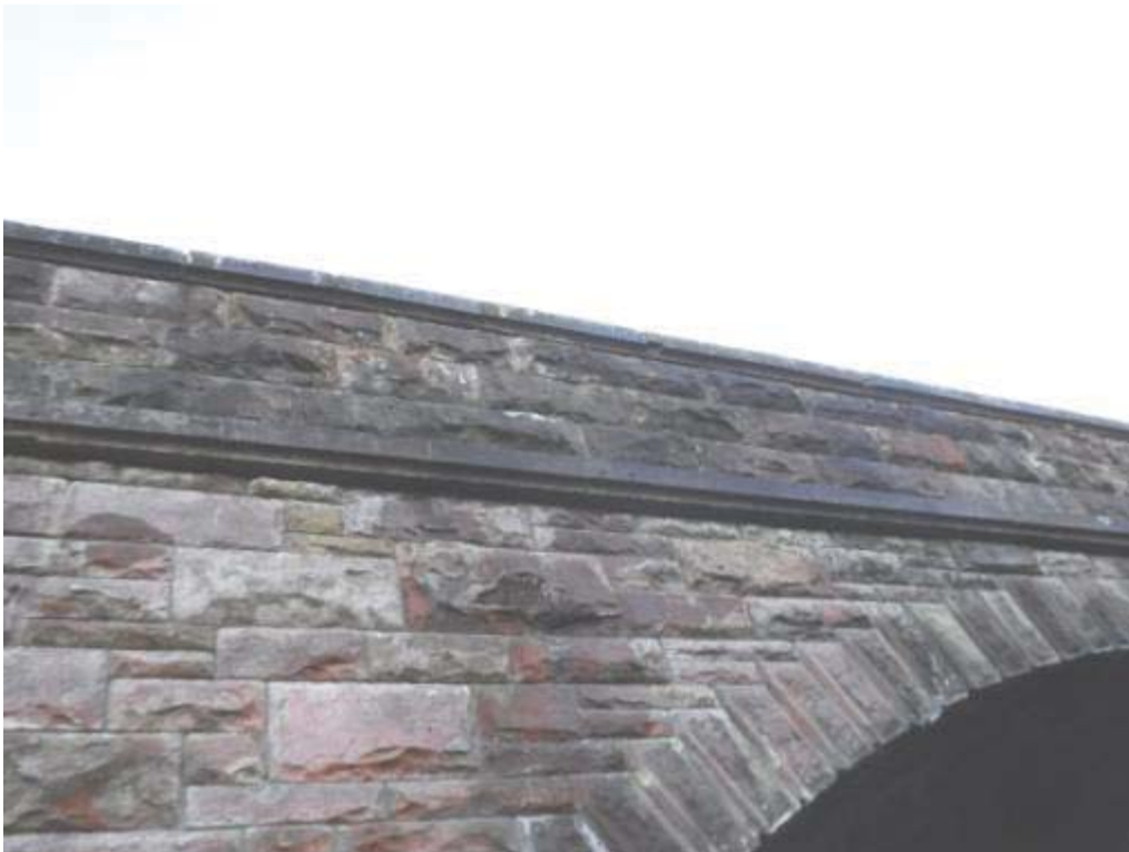
Photo No.42 - North spandrel: Typical example of the condition.
