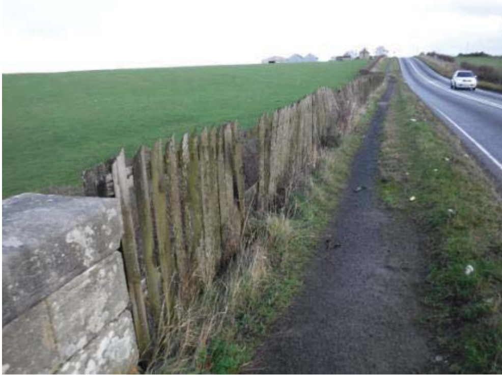
Photo No.159 - Approach road fencing: Typical example of the condition at N/E end.
