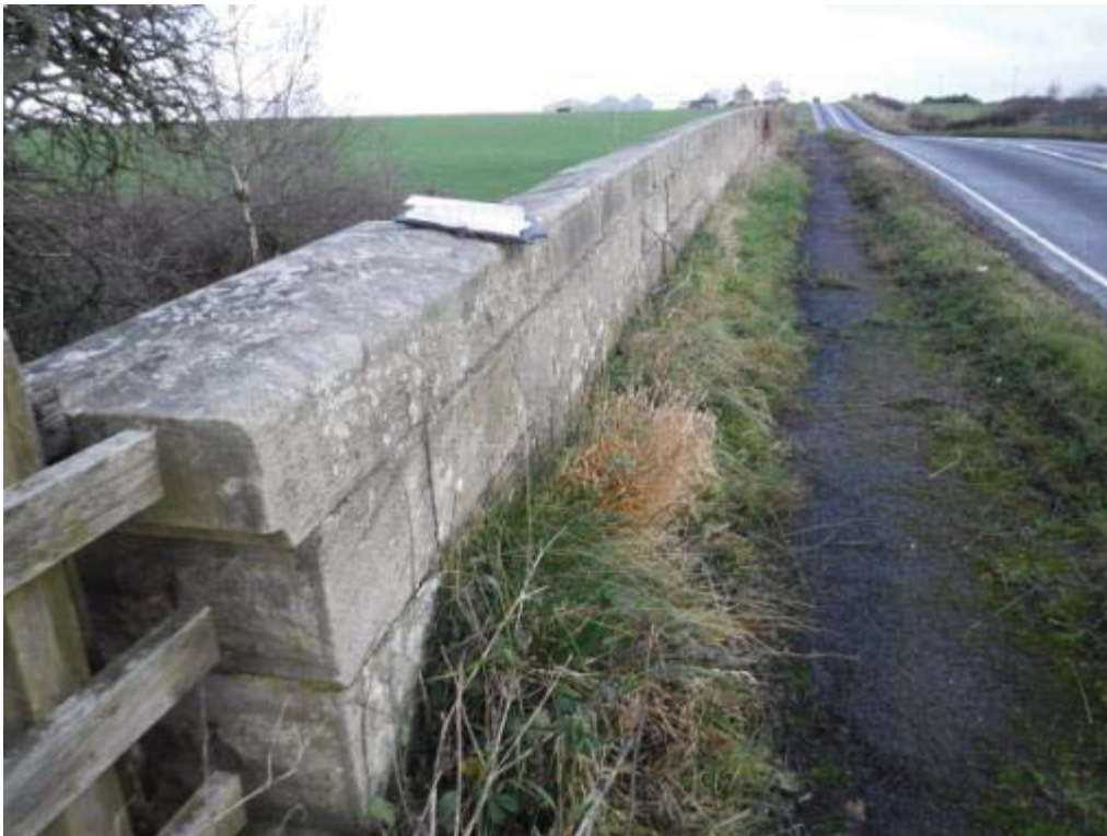
Photo No.102 - North roadside parapet: Displacement to the stonework at the N/W end.
