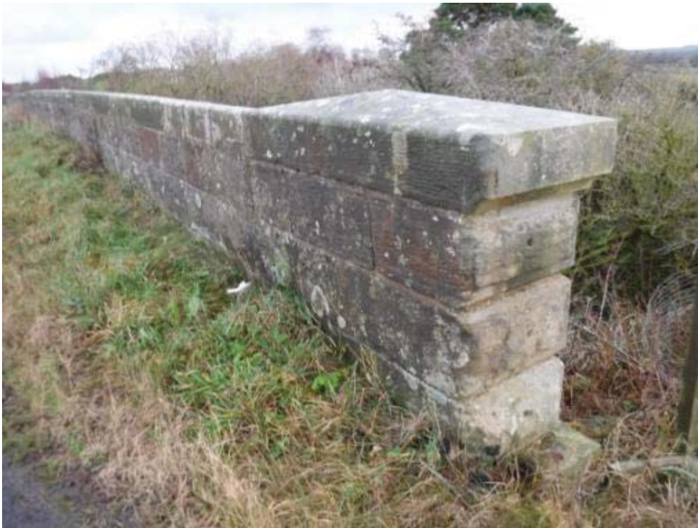
Photo No.128 - South roadside parapet: Previous vehicle impact damage to the S/W pilaster region rebuilt.
