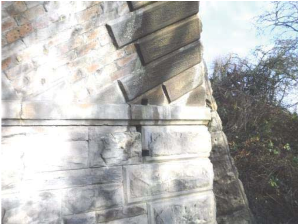
Photo No.148 - East springer course: Former S&T fixing void to the S/E end.
