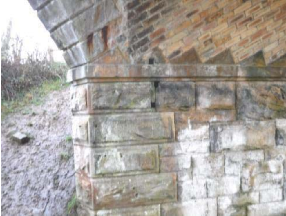
Photo No.55 - East abutment: Former S&T fixing voids to the stonework at the N/E end.
