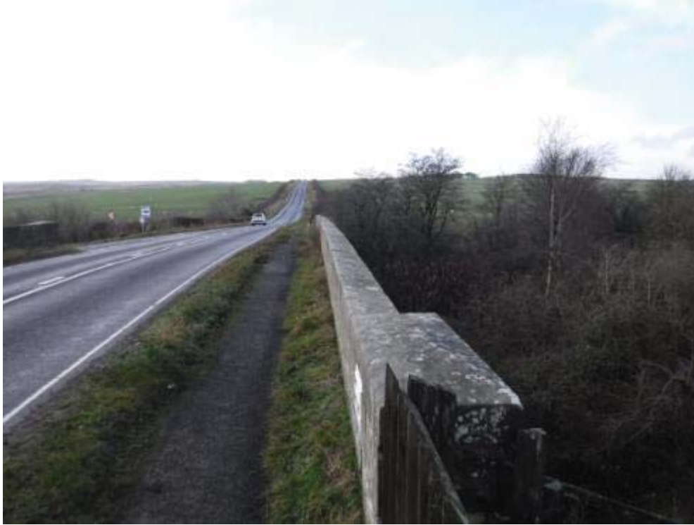
Photo No.115 - North roadside parapet: Typical example of the alignment & condition of the coping stones.
