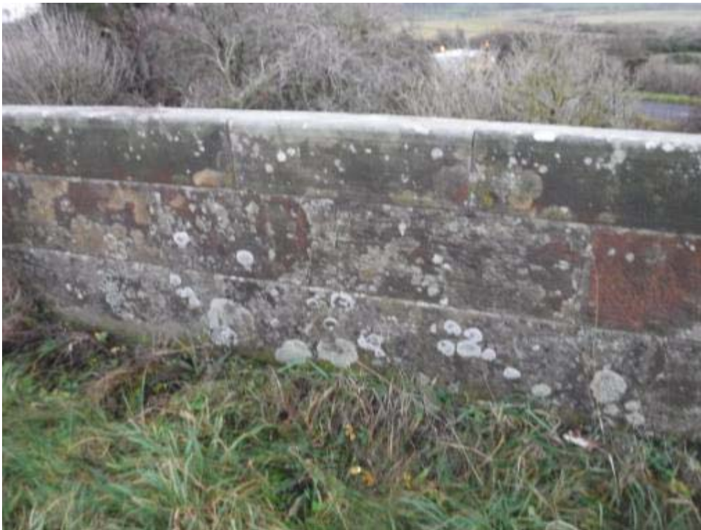
Photo No.130 - South roadside parapet: Typical example of the condition.
