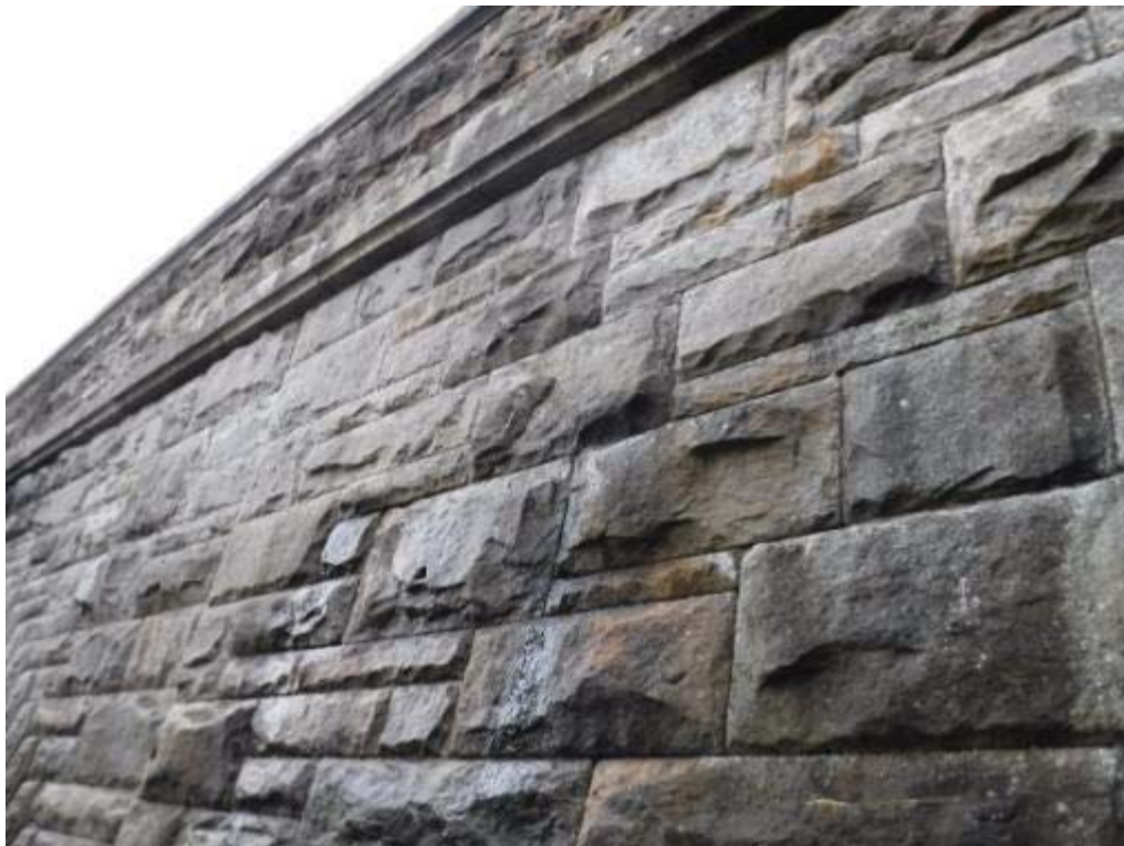
Photo No.92 - S/E wing wall: Typical example of the condition.
