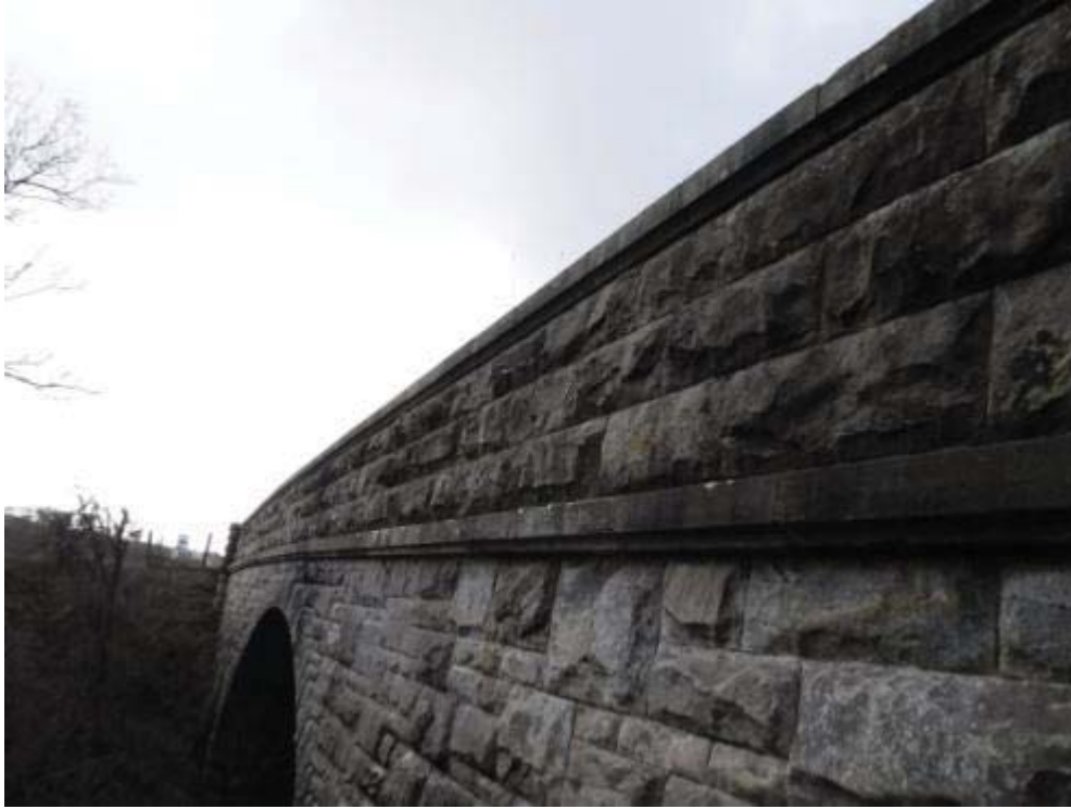
Photo No.143 - South outer parapet: Typical example of the condition.
