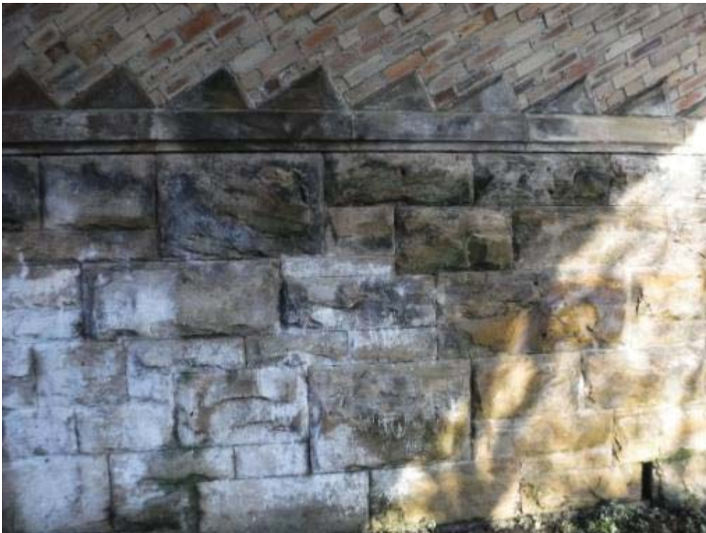
Photo No.58 - East abutment: Typical example of the condition.
