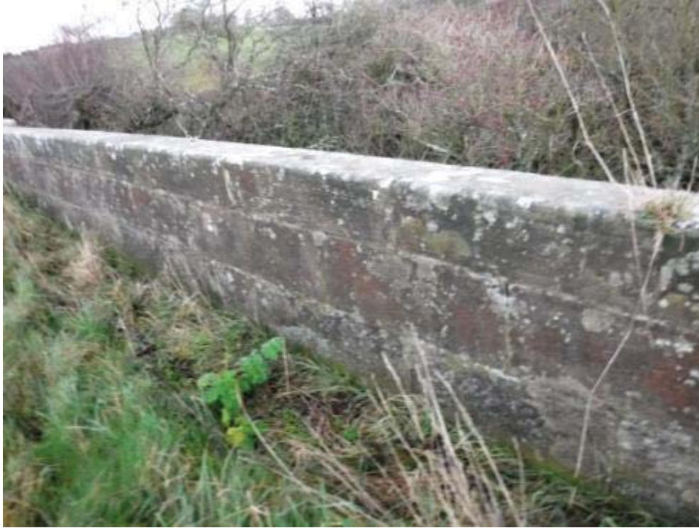
Photo No.133 - South roadside parapet: Typical example of the condition.
