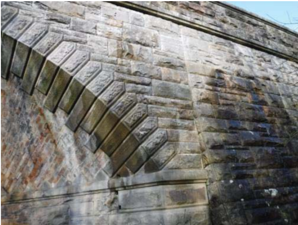
Photo No.48 - South spandrel: Typical example of the condition.
