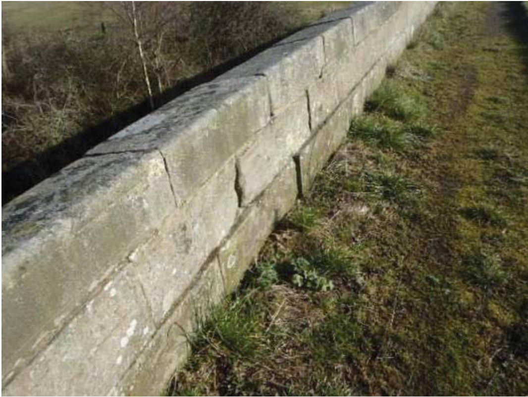
Photo No.2: North roadside parapet: Evidence of previous vehicular impact damage to the stonework.
