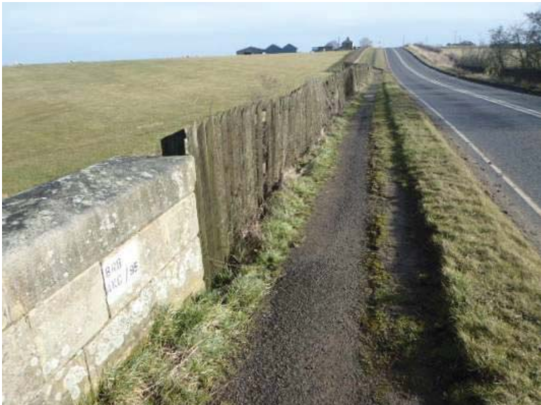
Photo No.1: Approach road fencing: Typical example of the condition at N/E end.
