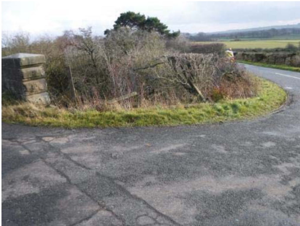
Photo No.162 - Approach road fencing: Typical example of the condition at S/W end.
