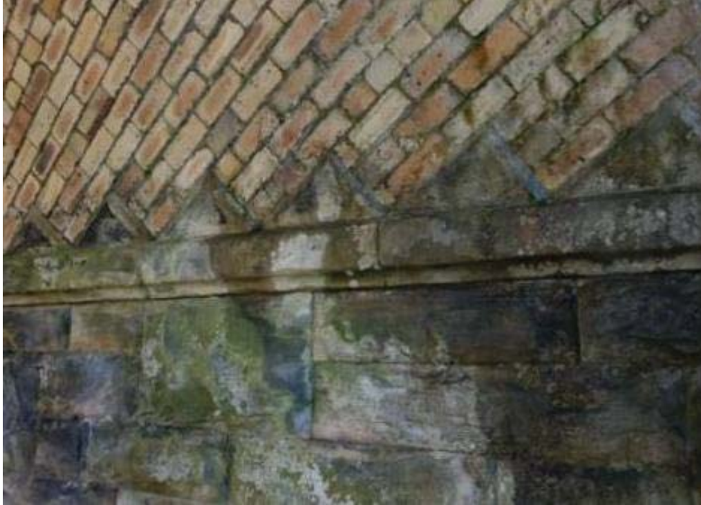
Photo No.151 - West springer course: Typical example of the condition.
