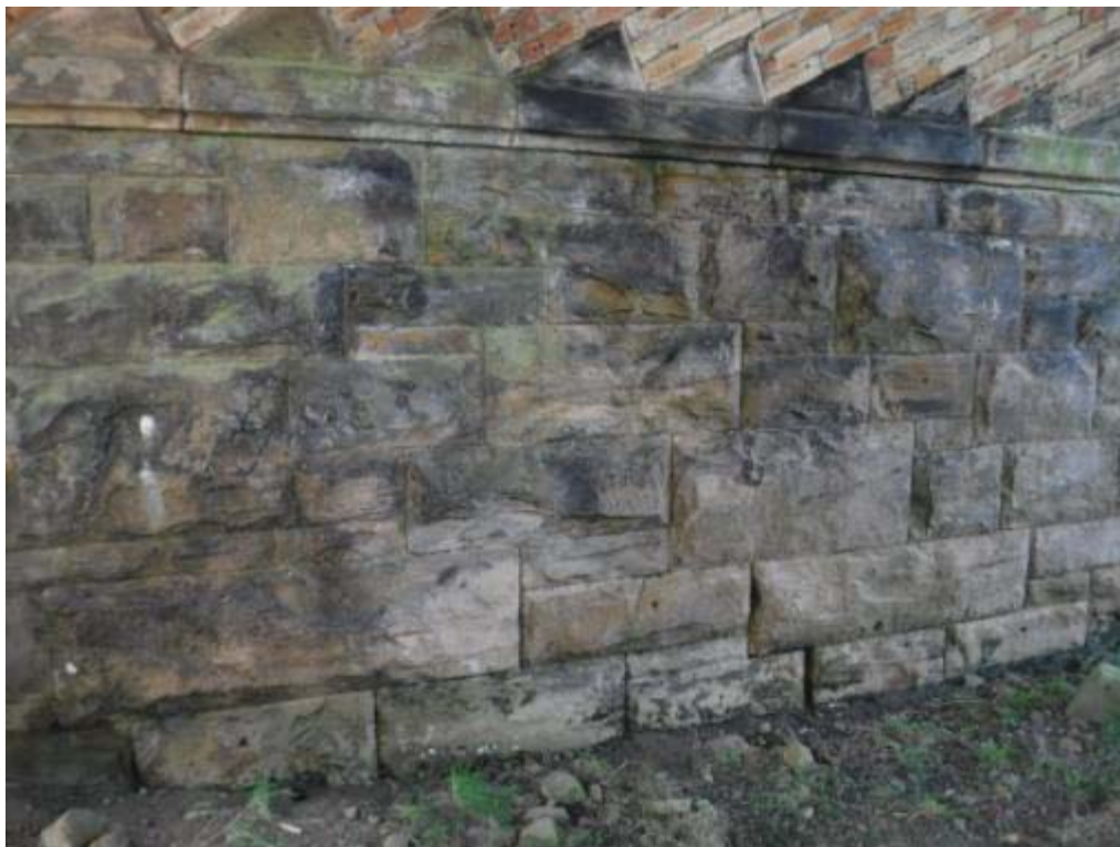
Photo No.68 - West abutment: Typical example of the condition.
