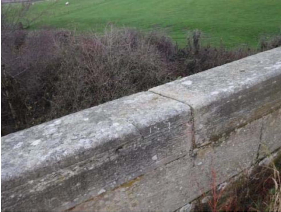
Photo No.107 - North roadside parapet: Fractured coping stone at 15.90m.
