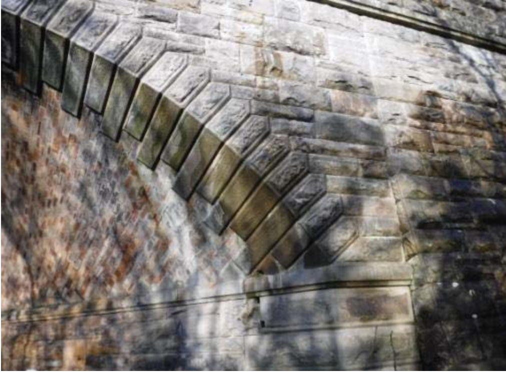
Photo No.23 - South arch ring face: Typical example of the condition.
