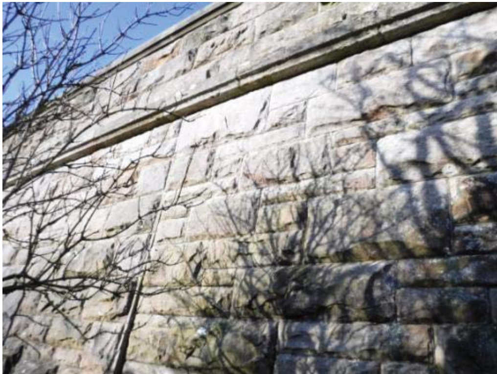
Photo No.52 - South spandrel: Typical example of the condition.
