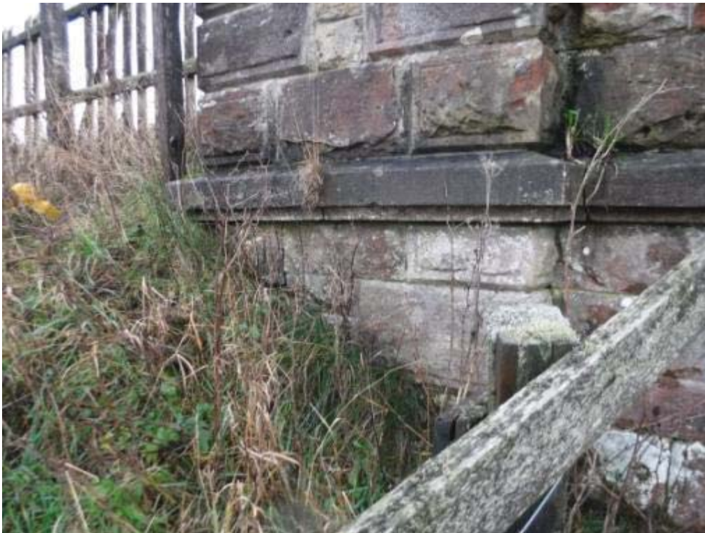
Photo No.80 - N/E wing wall: Typical example of the condition of the newel post.
