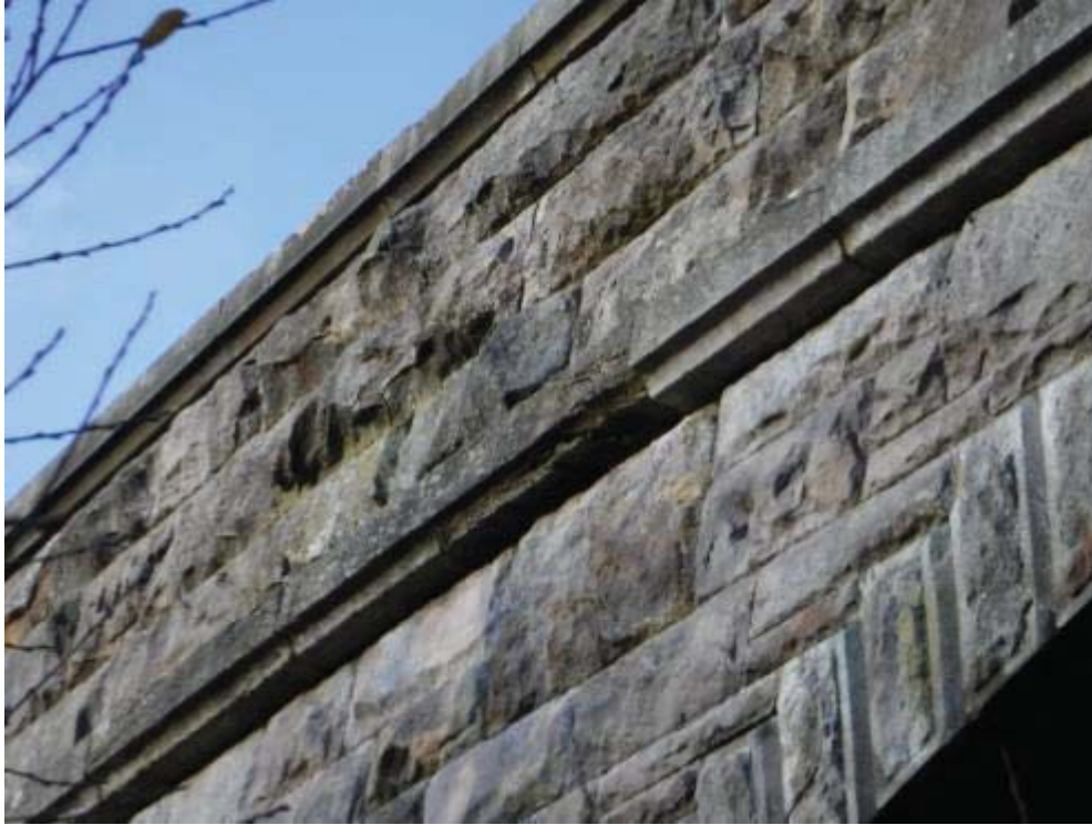
Photo No.153 - String course: Erosion to stonework with loss of face above the S/W ¼ point of the spandrel.
