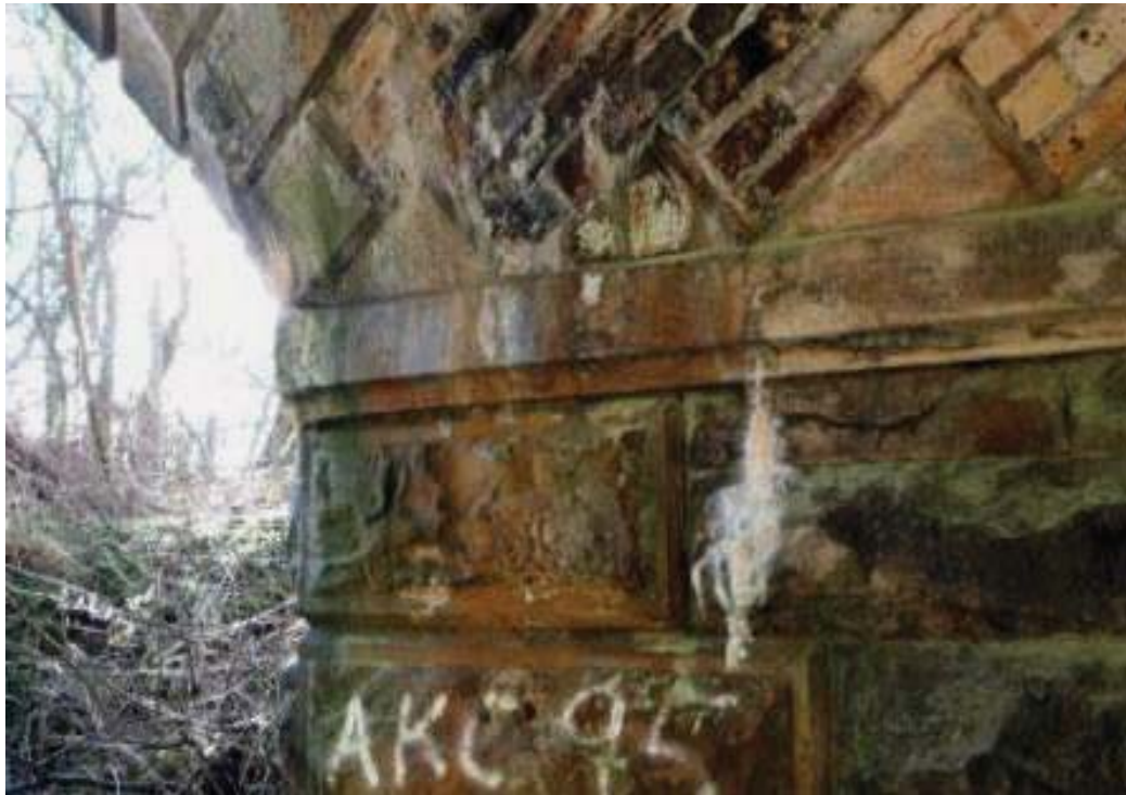
Photo No.152 - West springer course: Typical example of the condition at S/W return section.
