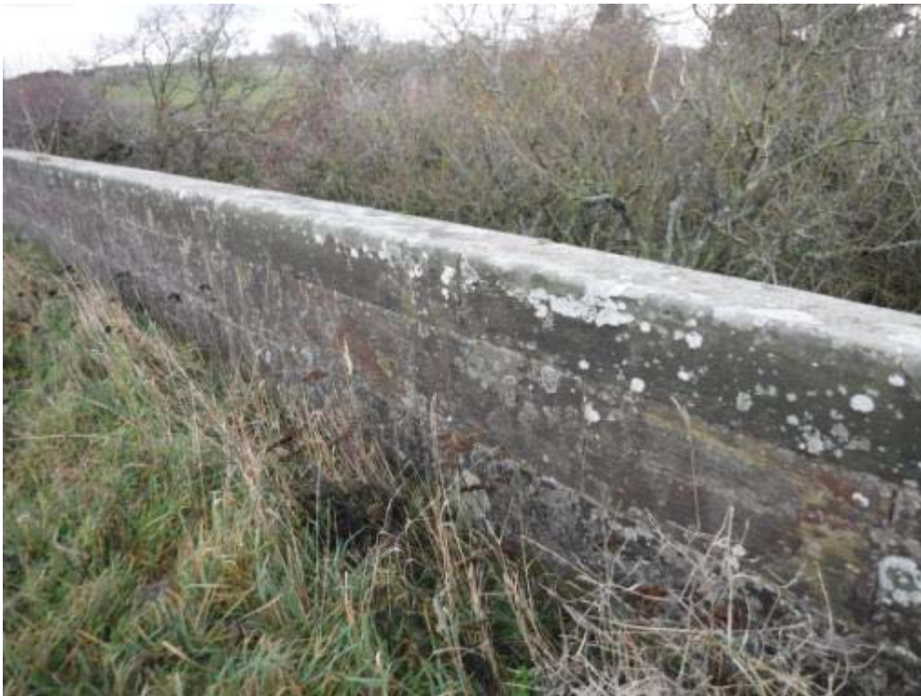
Photo No.132 - South roadside parapet: Typical example of the condition.
