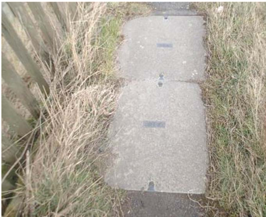
Photograph 9: BT chambers are located within the footpath
