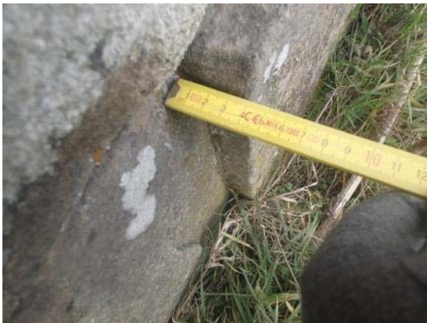
Photograph 13: the displacement was noted up to 40mm
