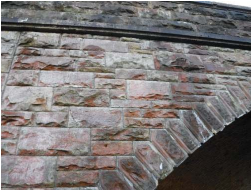
Photo No.40 - North spandrel: Typical example of the condition.
