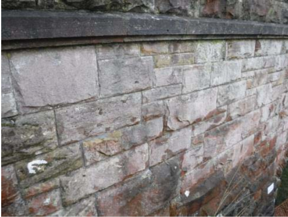
Photo No.77 - N/E wing wall: Typical example of the condition.
