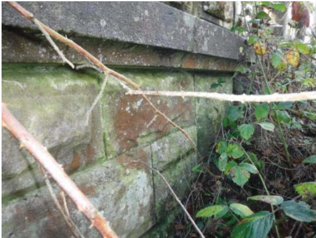
Photo No.86 - N/W wing wall: Typical example of the condition of the newel post.
