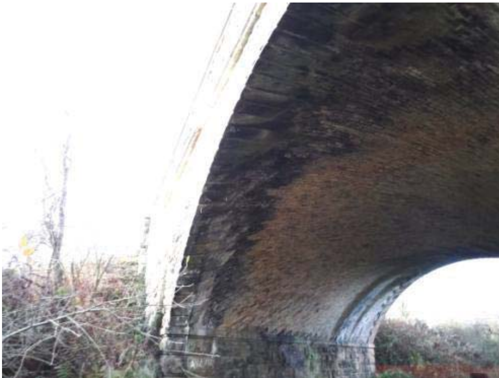
Photo No.24 - South arch ring face: Typical example of the condition of the underside.
