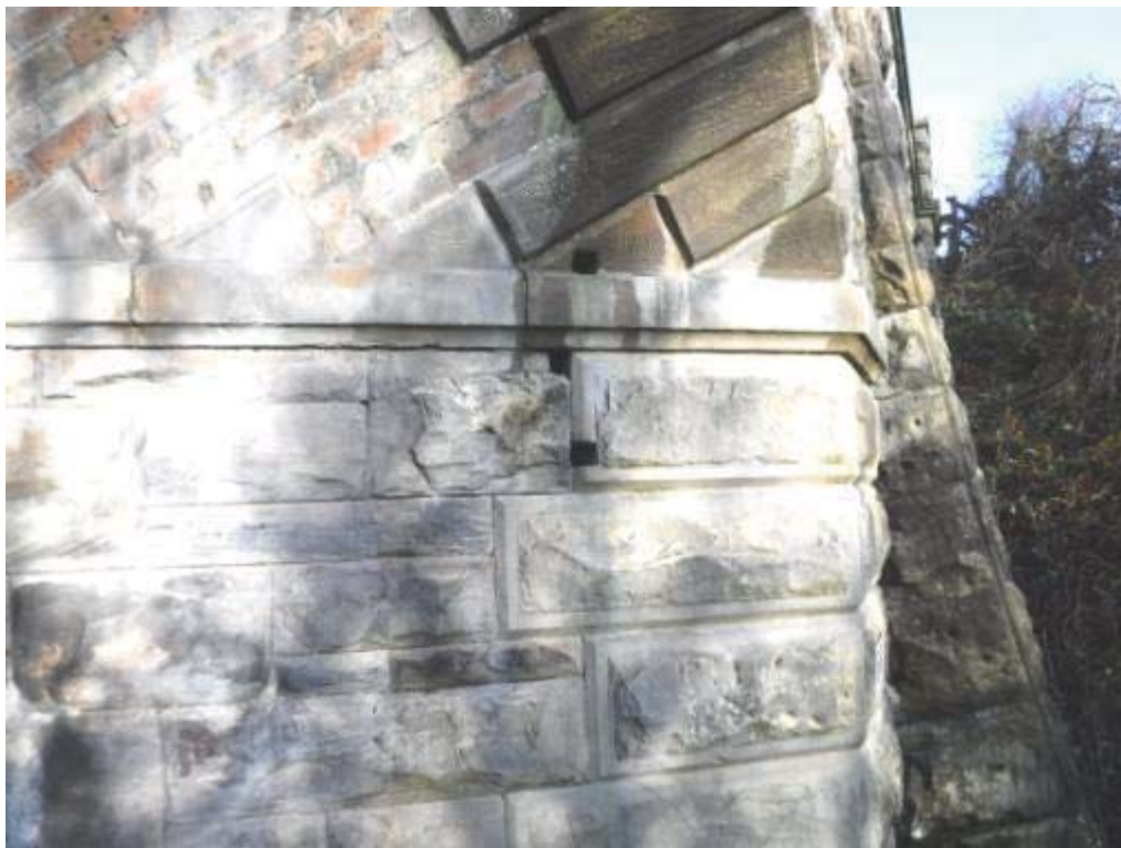
Photo No.56 - East abutment: Former S&T fixing voids to the stonework at the S/E end.
