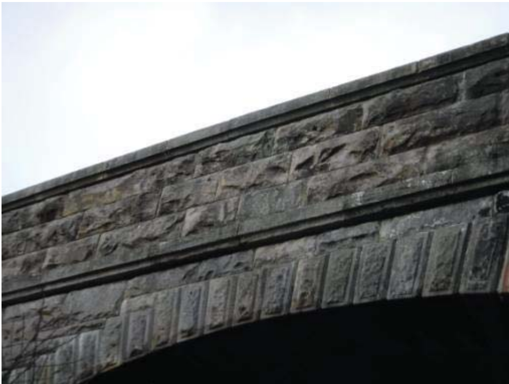
Photo No.142 - South outer parapet: Typical example of the condition.
