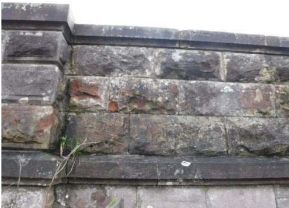
Photo No.124 - North outer parapet: Typical example of the condition.
