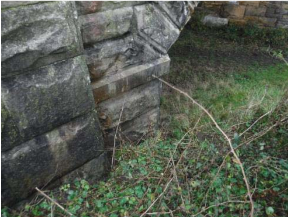
Photo No.73 - West abutment: Typical example of the condition at the S/W return section.
