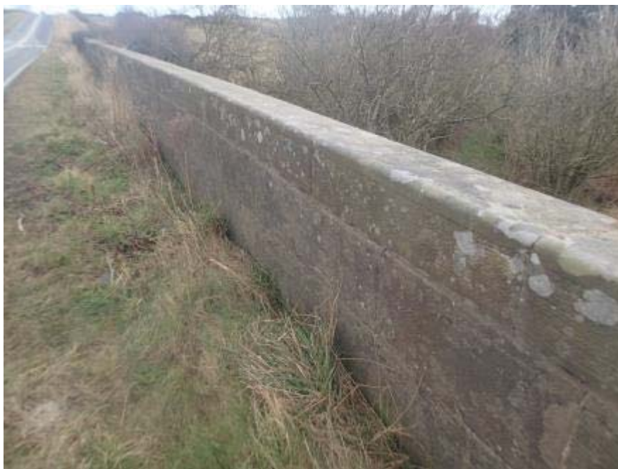
Photograph 15: example of long-standing displacement noted along the copings upon the south parapet
