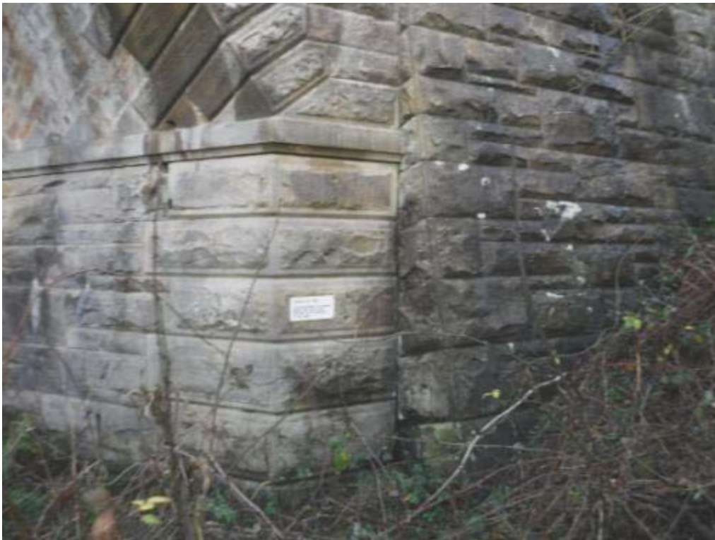
Photo No.64 - East abutment: Typical example of the condition at the S/E return section.
