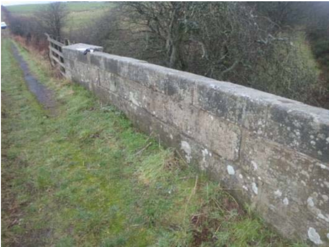
Photo No.7: Parapets: Evidence of previous vehicular impact damage to the stonework.
