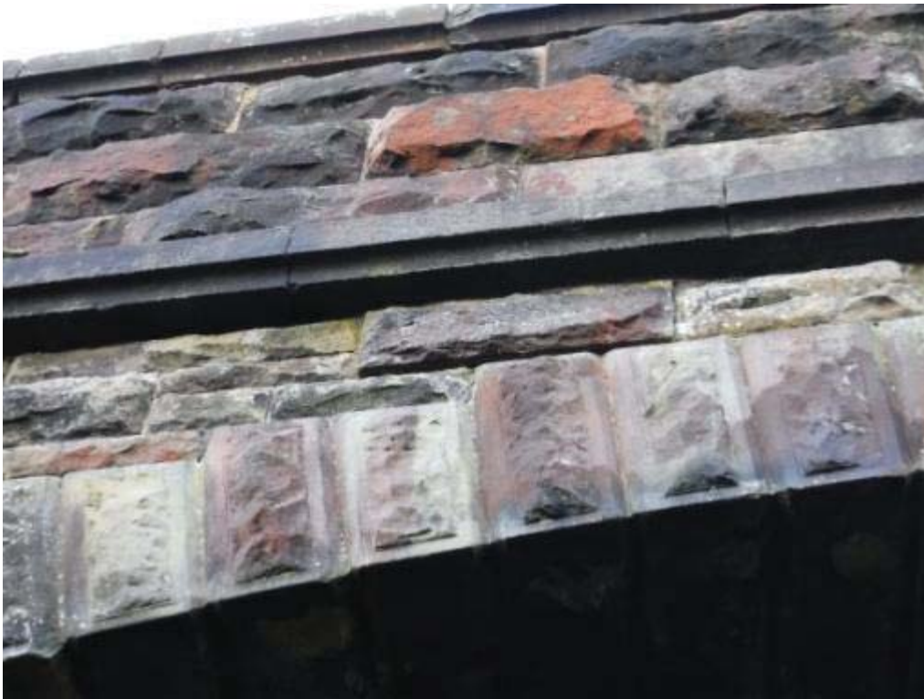
Photo No.38 - North spandrel: Oversailing to stonework at the N/E elevation.
