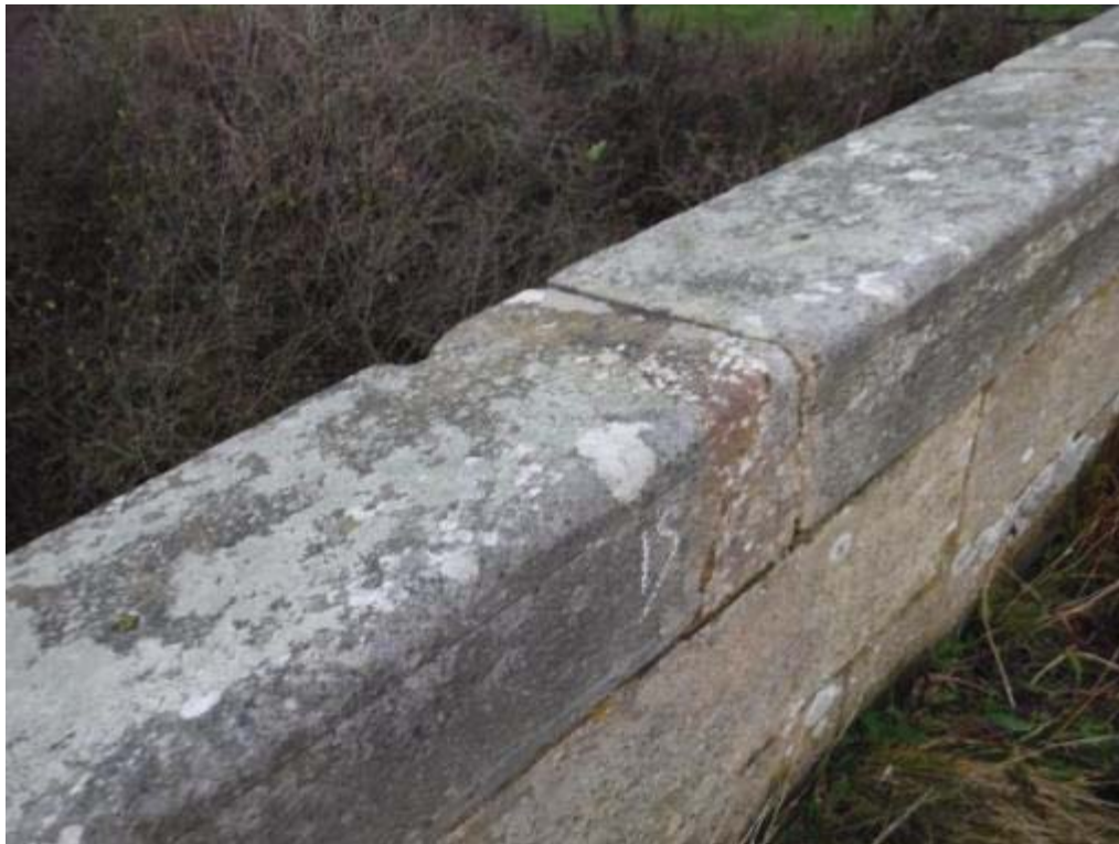
Photo No.106 - North roadside parapet: Fractured coping stone at 15.00m.
