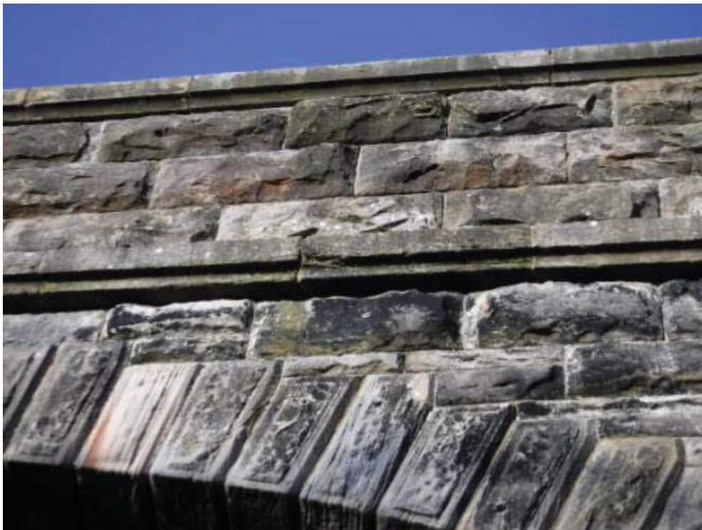
Photo No.154 - String course: Erosion to stonework with loss of face above the S/E ¼ point of the spandrel.
