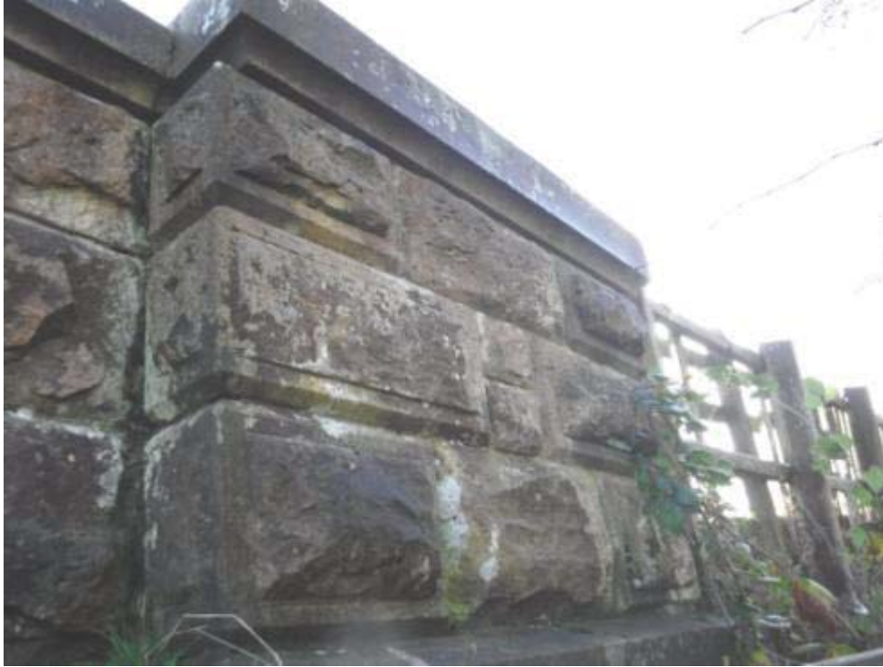
Photo No.117 - North outer parapet: Typical example of the condition of the N/W pilaster.
