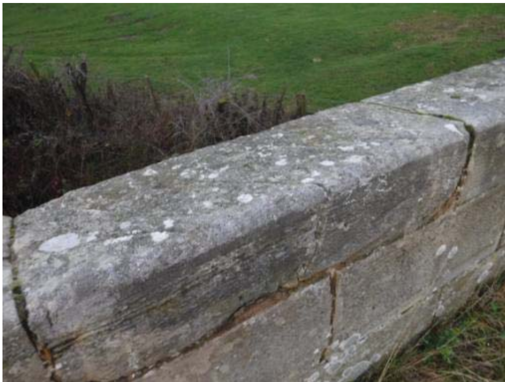
Photo No.110 - North roadside parapet: Fractured coping stone at 23.80m.
