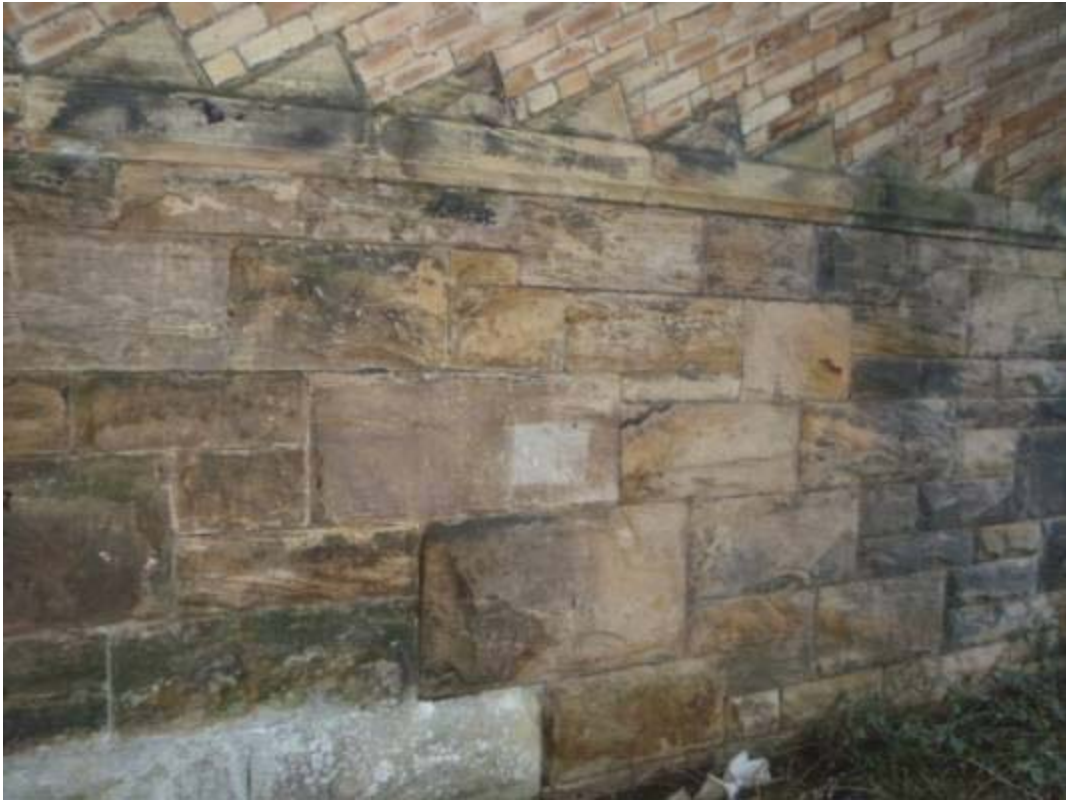
Photo No.6: BRB lettering: Erased.
