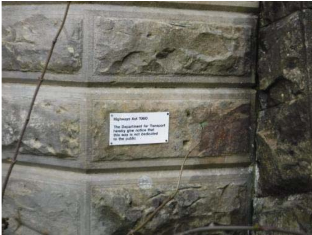
Photo No.166 - Non - Dedication plate: Typical example of the condition.
