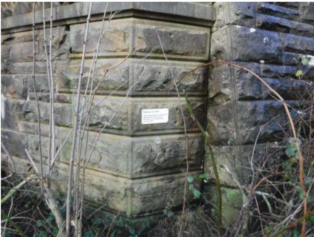
Photo No.3: Non - Dedication plate: Typical example of the condition.
