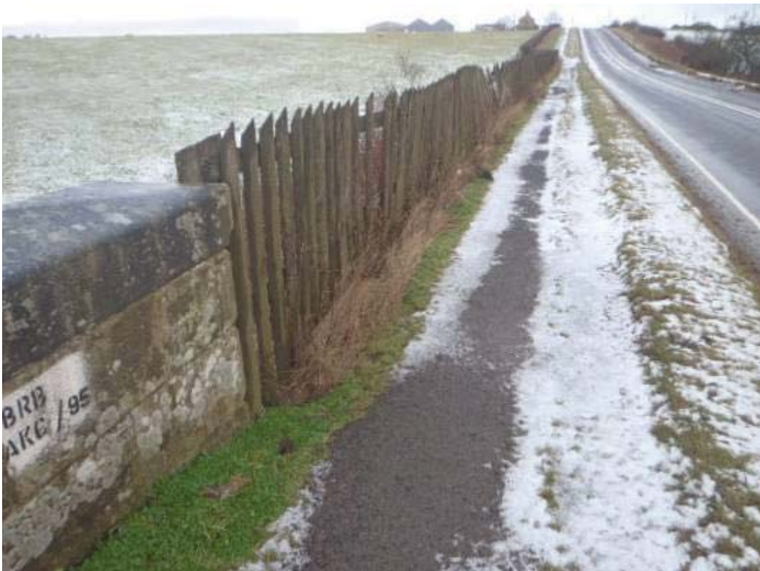
Photo No.3: Approach road fencing: Typical example of the condition at N/E end.
