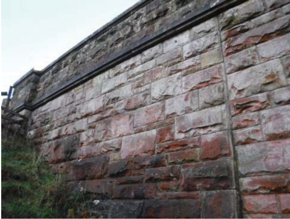
Photo No.79 - N/E wing wall: Typical example of the condition.
