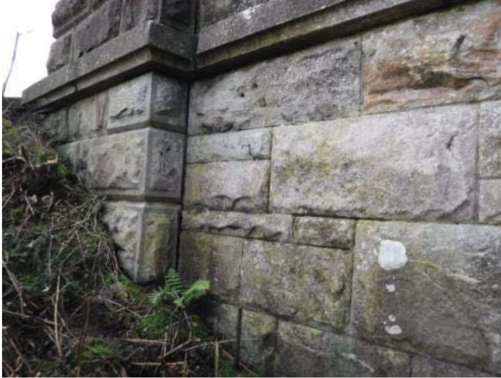
Photo No.95 - S/W wing wall: Typical example of the condition.
