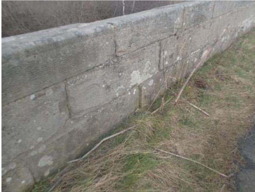
Photograph 12: example of long-standing displaced stonework noted along the north parapet
