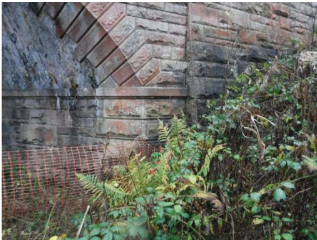
Photo No.74 - West abutment: Typical example of the condition at the N/W return section.
