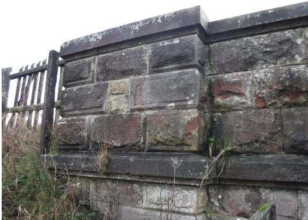
Photo No.125 - North outer parapet: Typical example of the condition of the N/E pilaster.
