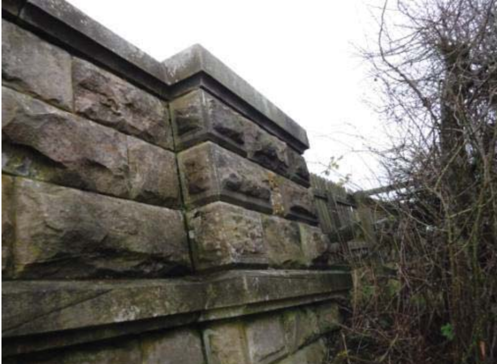
Photo No.145 - South outer parapet: Typical example of the condition of the S/E pilaster.
