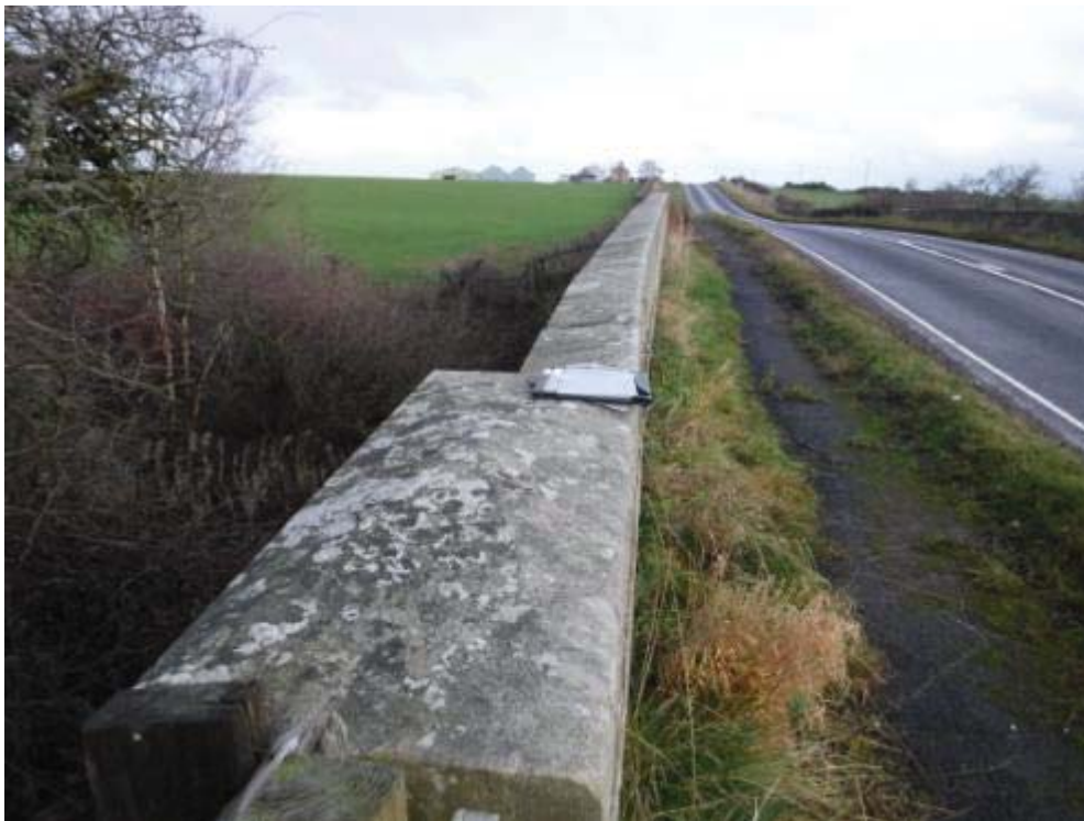
Photo No.114 - Typical example of the alignment & condition of the coping stones.
