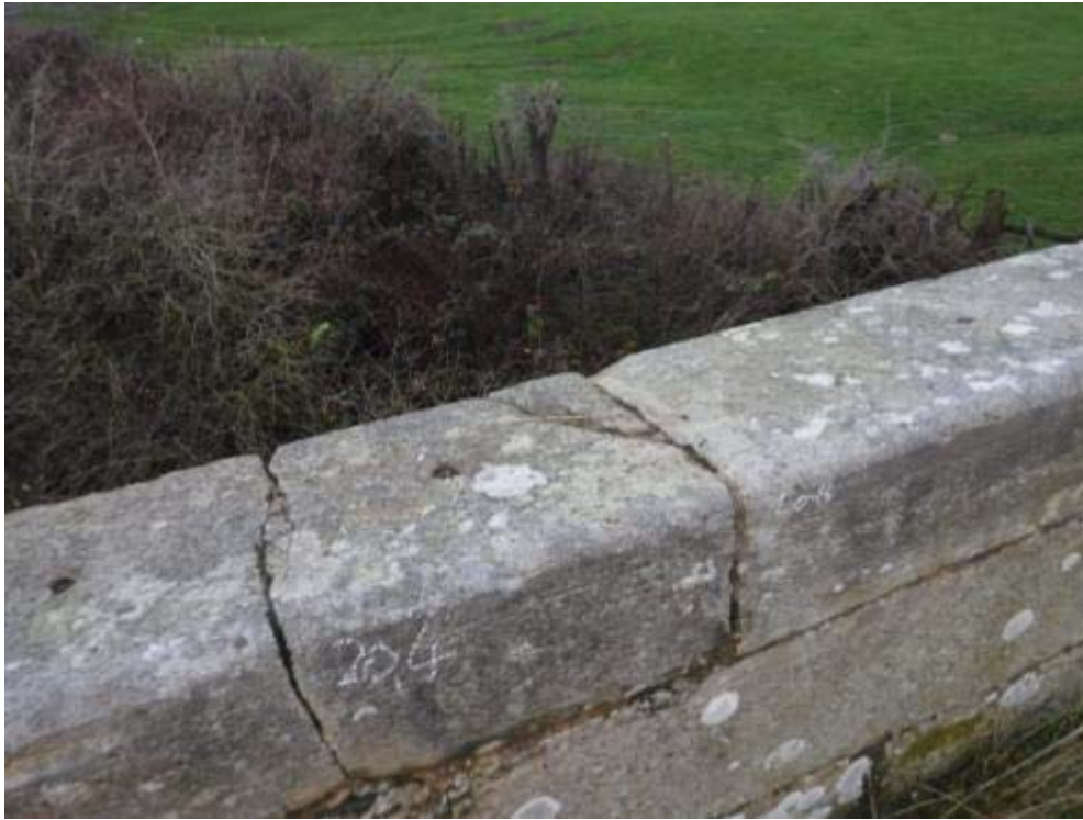
Photo No.109 - North roadside parapet: Fractured coping stone at 20.40m & 20.80m.
