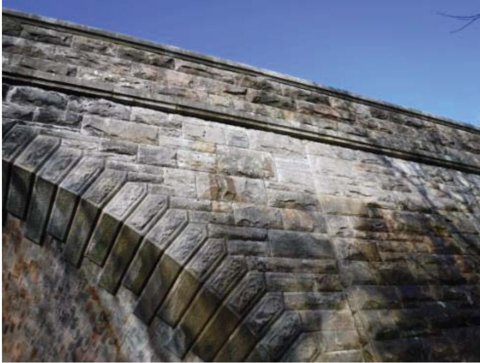
Photo No.49 - South spandrel: Typical example of the condition.
