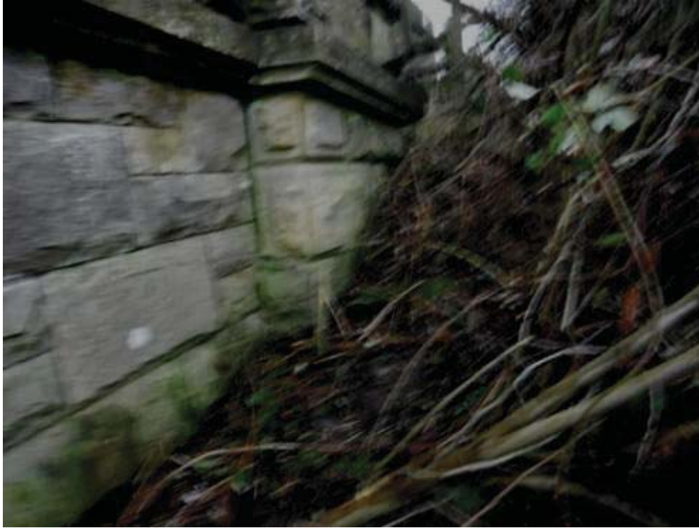
Photo No.93 - S/E wing wall: Typical example of the condition of the newel post.
