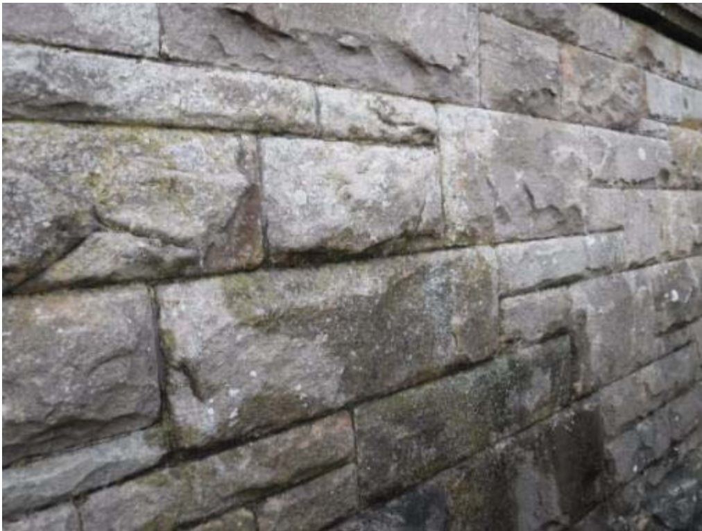
Photo No.96 - S/W wing wall: Typical example of the condition.
