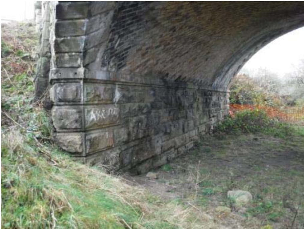
Photo No.72 - West abutment: Typical example of the condition.
