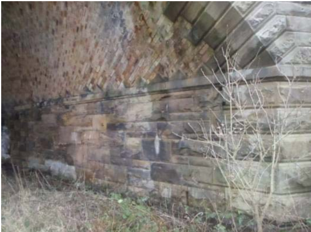
Photo No.1: Possible further deterioration: To the eroded stonework areas.
