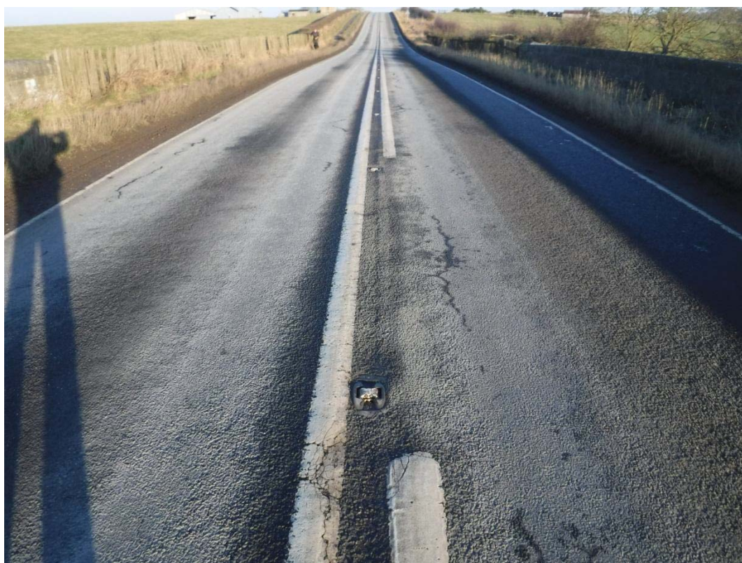
Photo No.3: Road surface: Typical example of the condition.
