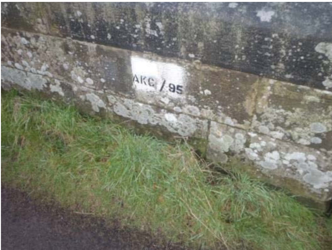
Photo No.5: BRB lettering: Erased.
