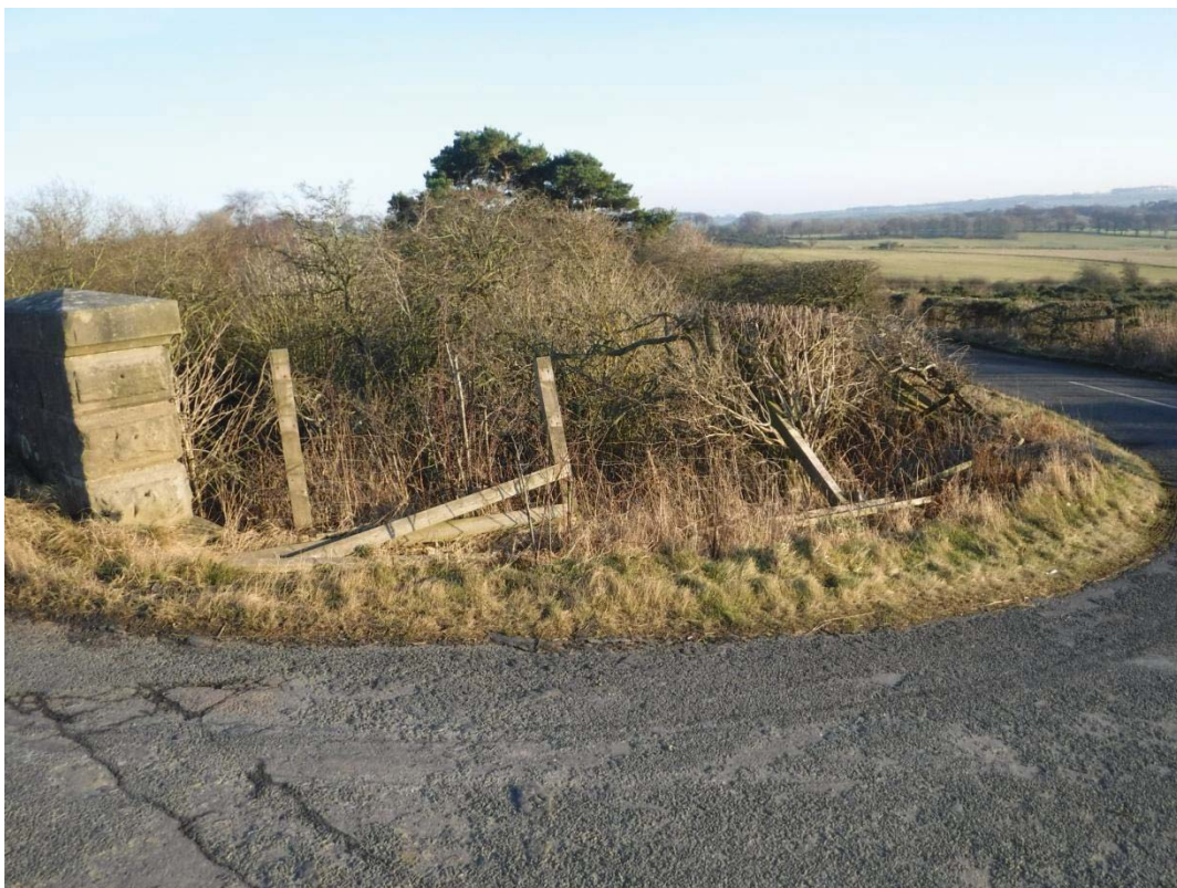
Photo No.1: S/W Approach road fencing: Possible vehicle impact damage.
