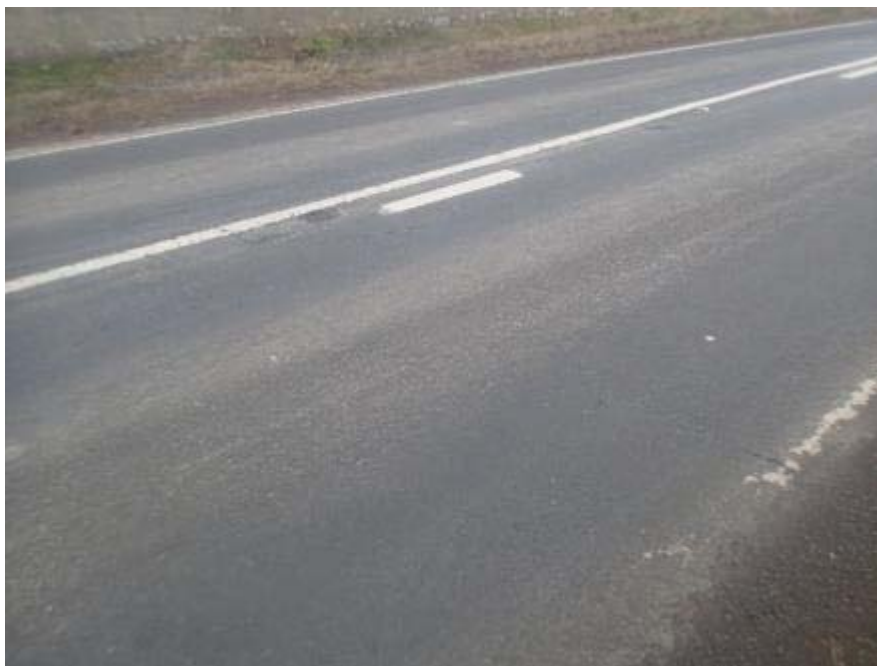
Photograph 21: odd surface fractures were noted within the asphalt
