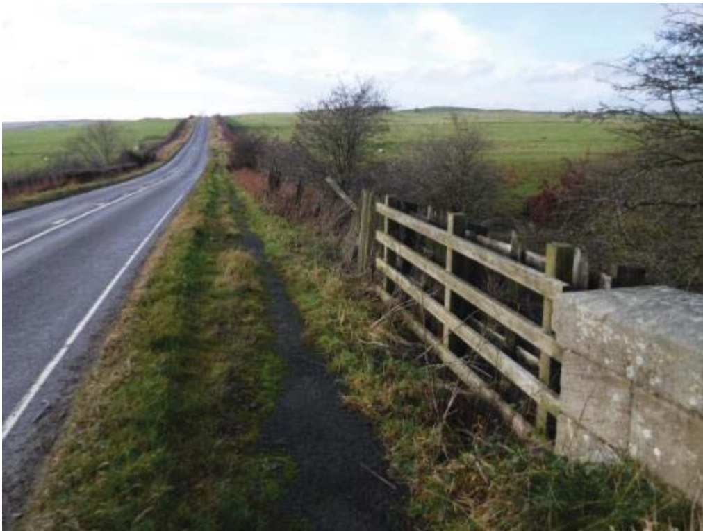
Photo No.160 - Approach road fencing: Typical example of the condition at N/W end.
