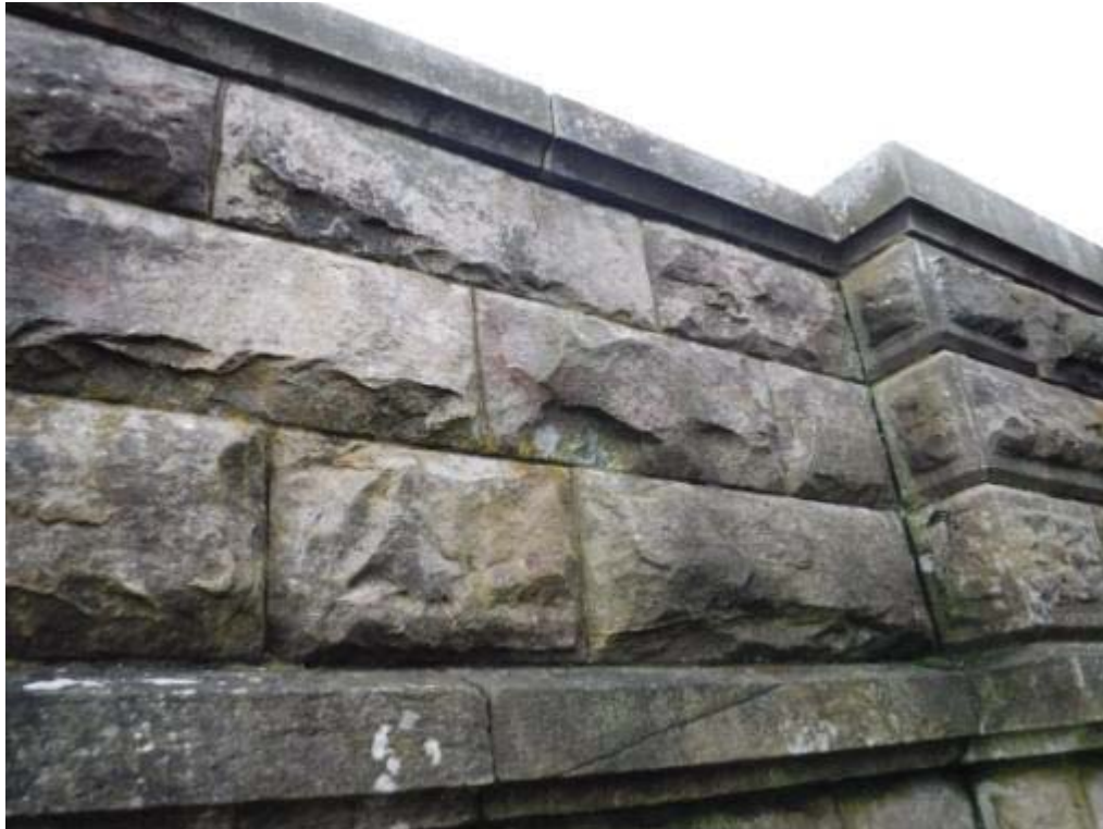
Photo No.144 - South outer parapet: Typical example of the condition.
