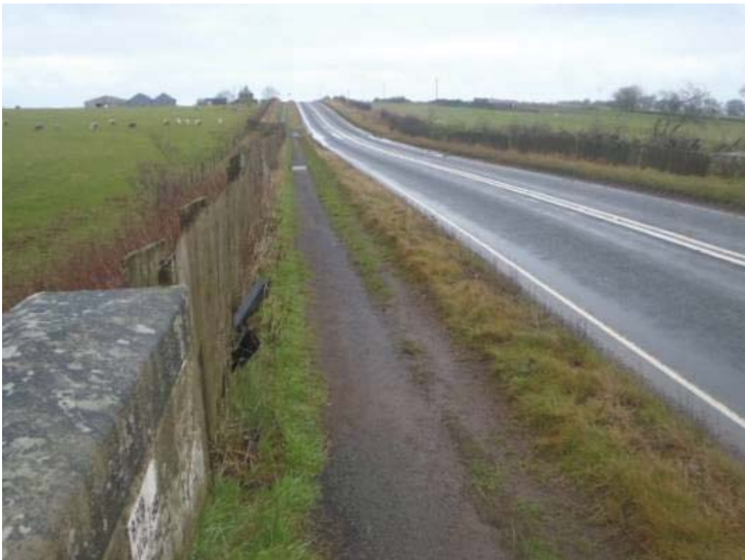
Photo No.3: Approach road fencing: Typical example of the condition at N/E end.
