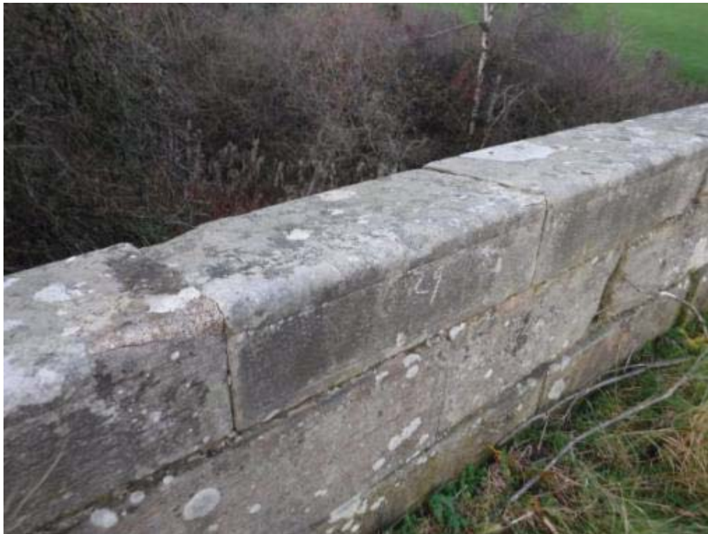
Photo No.104 - North roadside parapet: Fractured coping stone at 2.90m.
