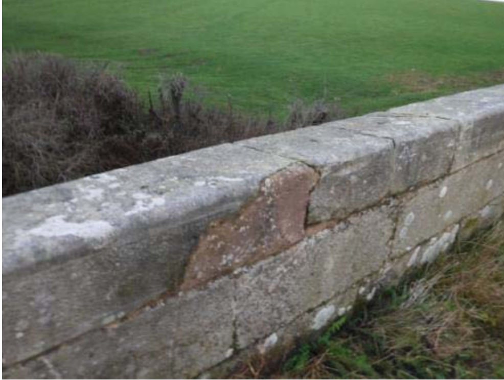
Photo No.111 - North roadside parapet: Previous render repair.
