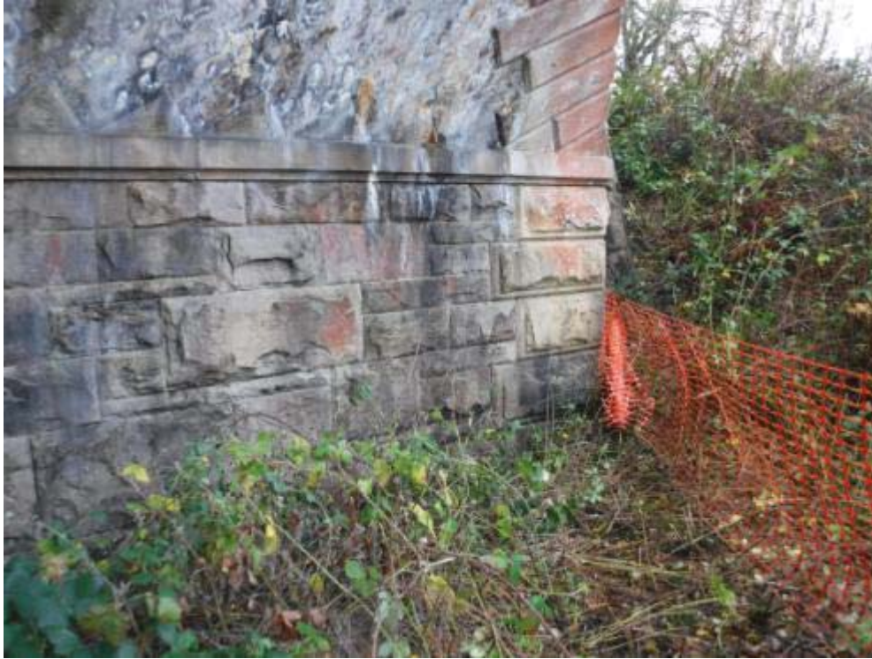
Photo No.71 - West abutment: Typical example of the condition.
