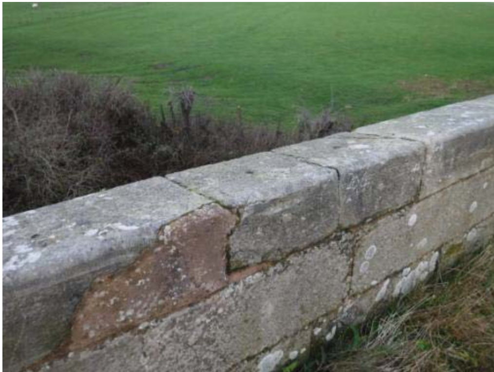
Photo No.108 - North roadside parapet: Fractured coping stone at 20.40m.
