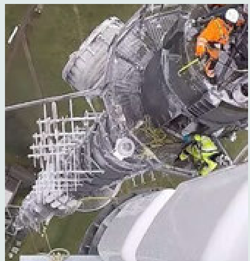
A new antenna being lifted into place onto the top of a mast by a helicopter. Note the engineer waiting to "catch it".
