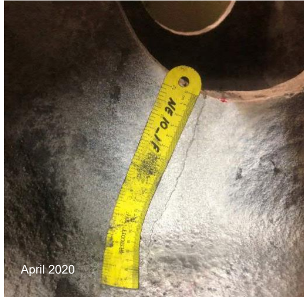
Figure 2.4 – Crack NE10 April 2020 Inside Face
