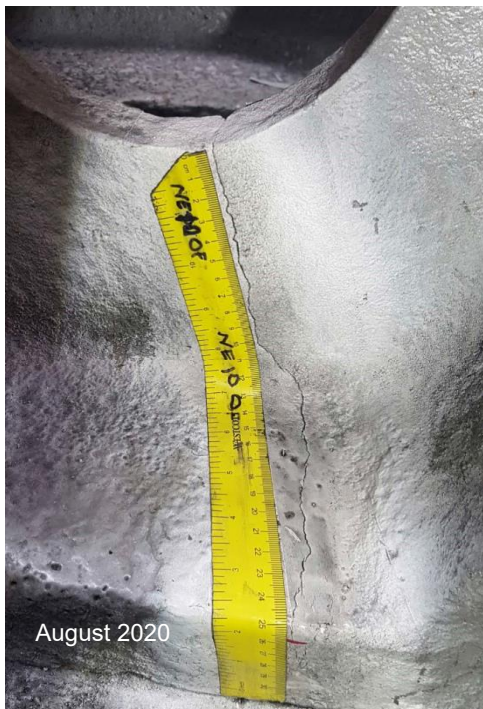
Figure 2.5 – Crack NE10 August 2020 Outside Face (source all pictures: MM)
