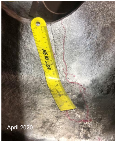
Figure 2.3 – Crack NE10 April 2020 Outside Face
